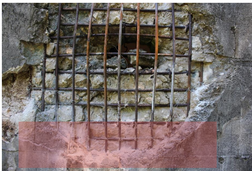
Figure 23. Battle-damage on east side. Shaded box indicates area of the realkalization trial.
