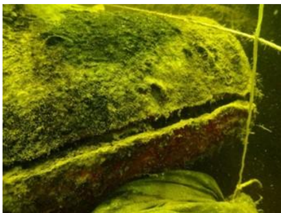
1. Crack along the welding seam
