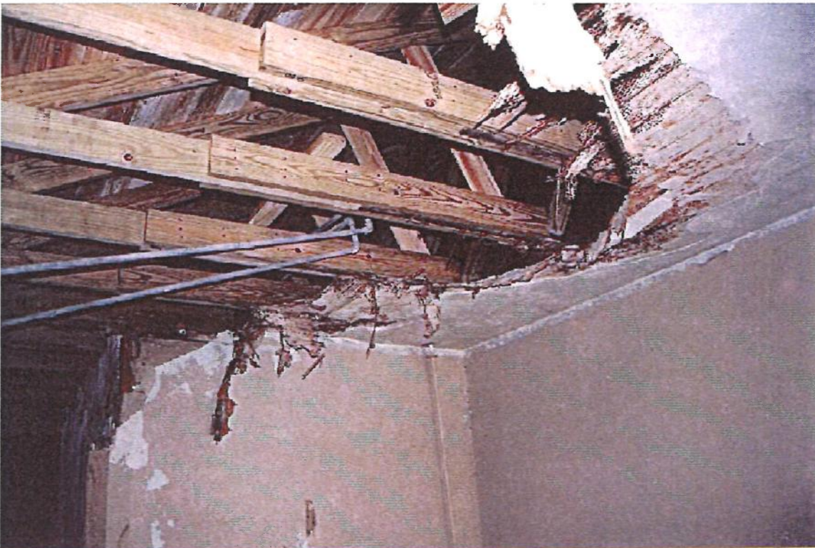
Figure 12: Deteriorated condition of plaster ceiling in the first aid room.
