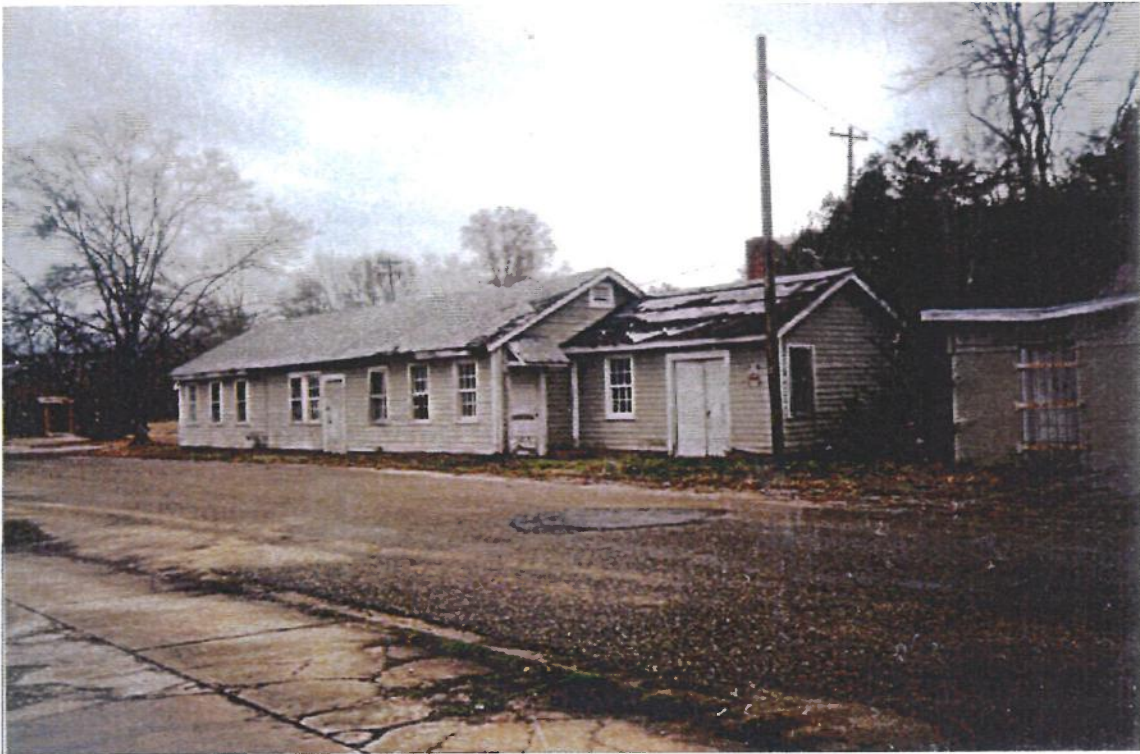
Figure 7: Oil Storage Shed prior to stabilization work. Pond & Company.
