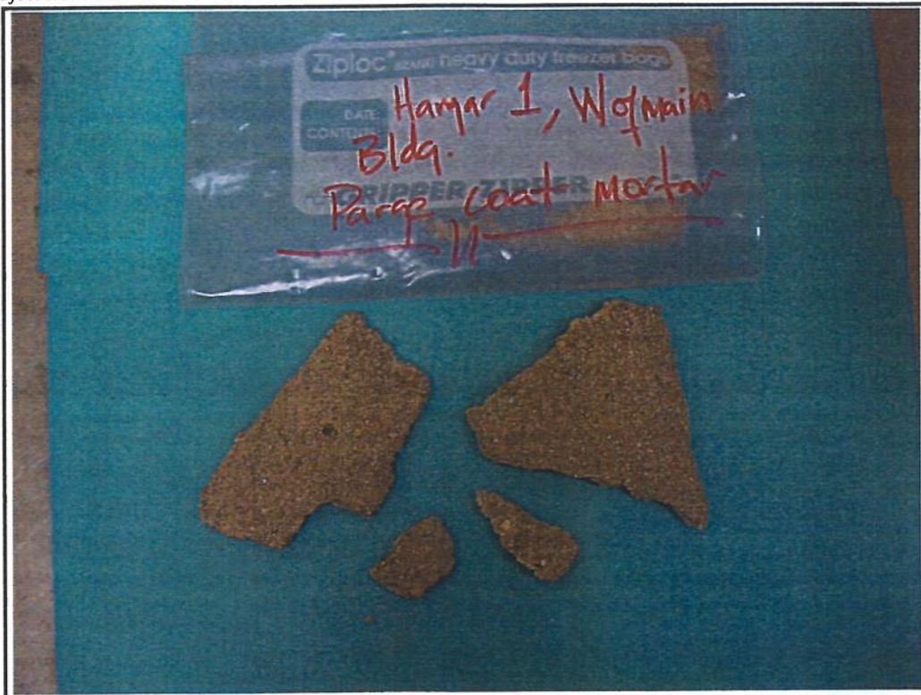
Photo 11. Hangar No. 1, Interior – Parge coat mortar observed. Note sand particles on surface poorly bonded to mortar.
