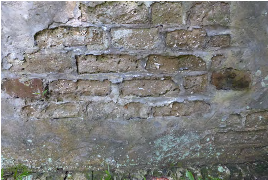
Image 20. Portland cement repair materials have caused deterioration in adjacent tabby brick.
