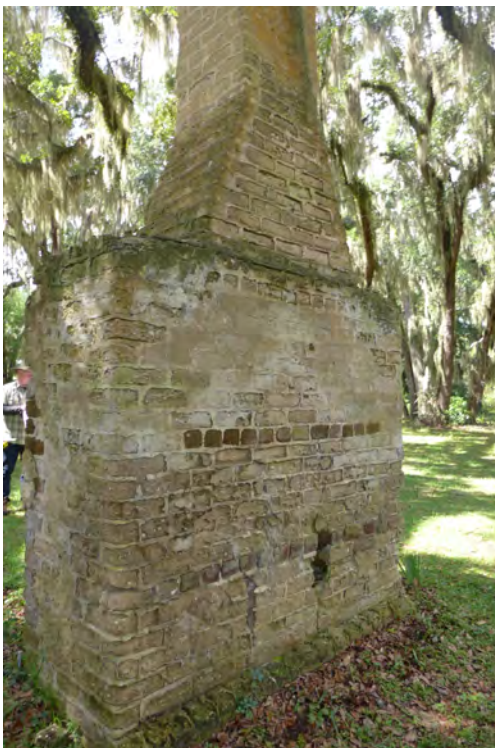
Image 18. The exterior side of the hearth is typically in poor condition on most chimneys, as is visible in this photograph.
