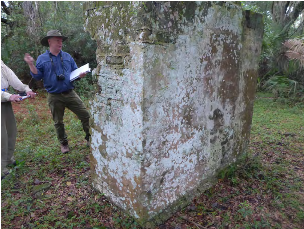
Image 17. The thin, brown-colored parging that is present on some of the chimneys (usually in partial form) is visible on this chimney.
