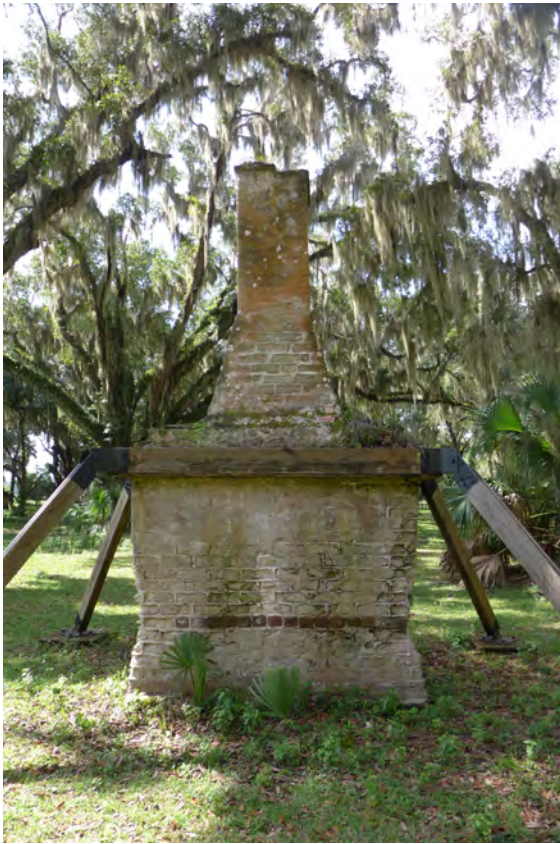
Image 19. This chimney clearly exhibits the typical deterioration pattern of eroded corners of the chimney base.
