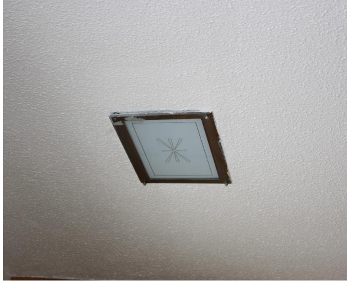
Figure 39. Recessed ceiling mounted etched glass light cover in kitchen.
