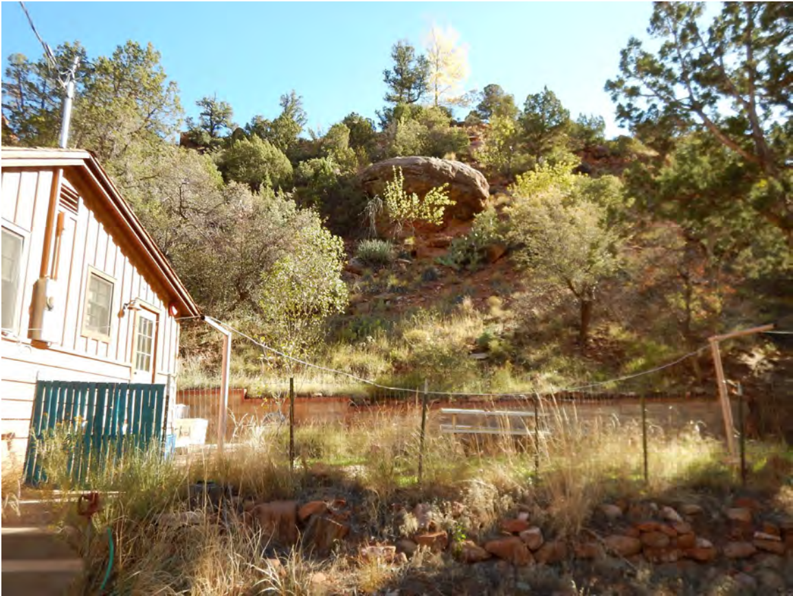
Figure 1435C: Photograph of slope above residence with unstable boulders.
