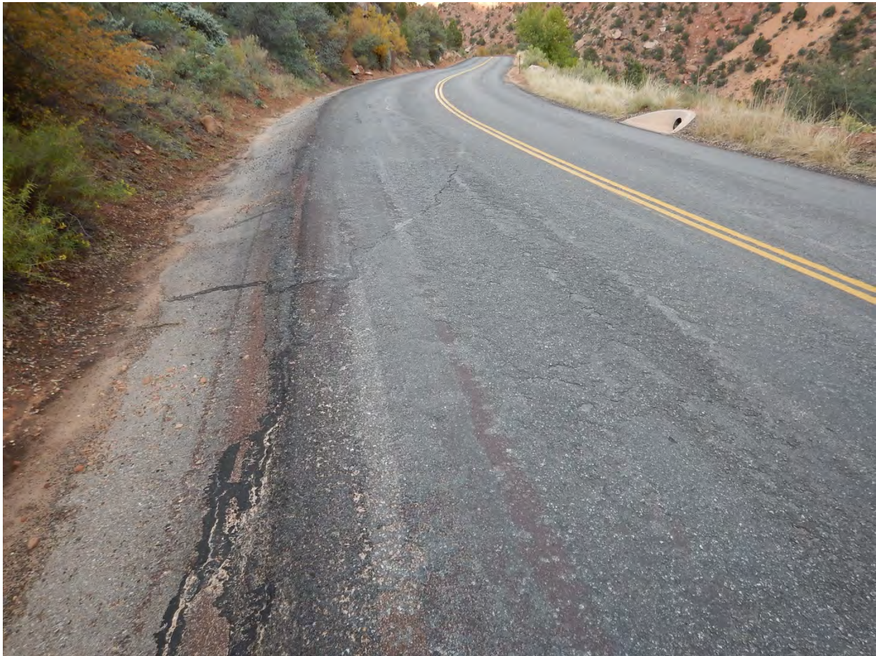
Figure 2-4 Arcuate Shaped Road Distress at "Carl's Bend" Landslide Area.
