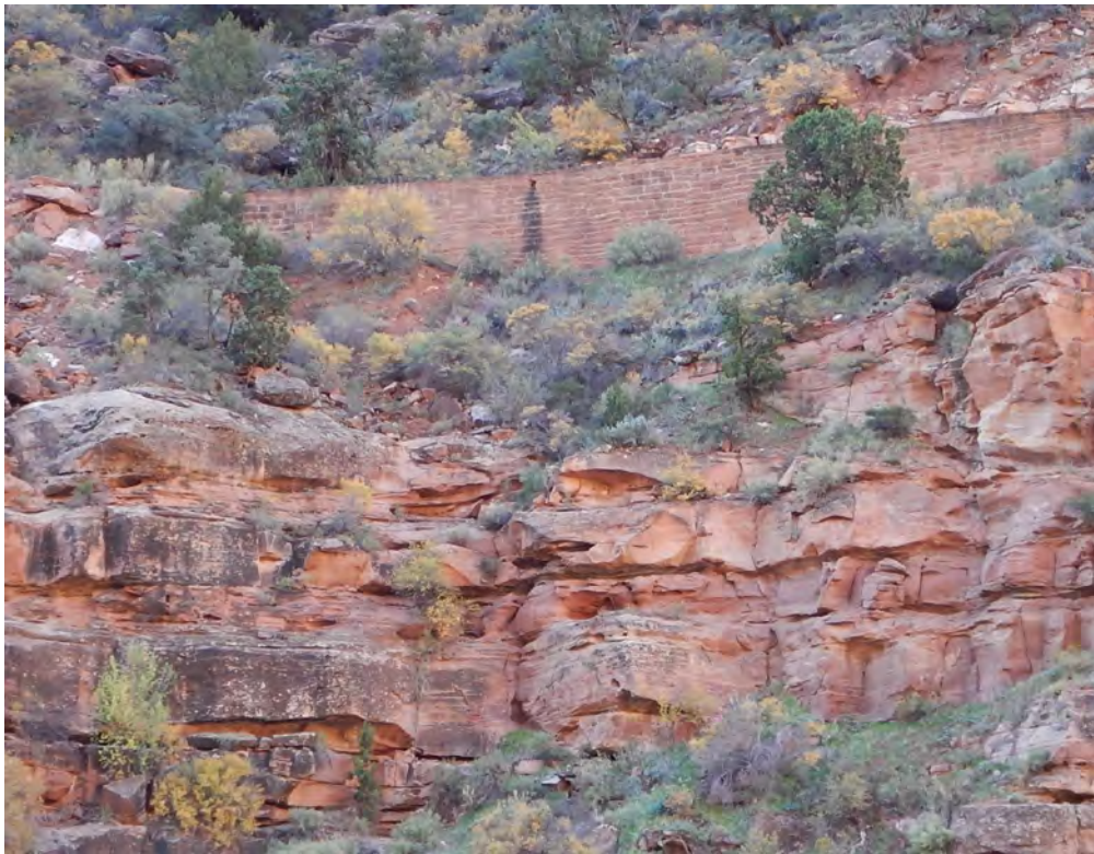
Photograph 1004-B: Drainage 2 from switchback culvert outlet in upper retaining wall at top of cutslope. Recommended riprap rundown for reduction of undercutting erosion at the base of the slope.
