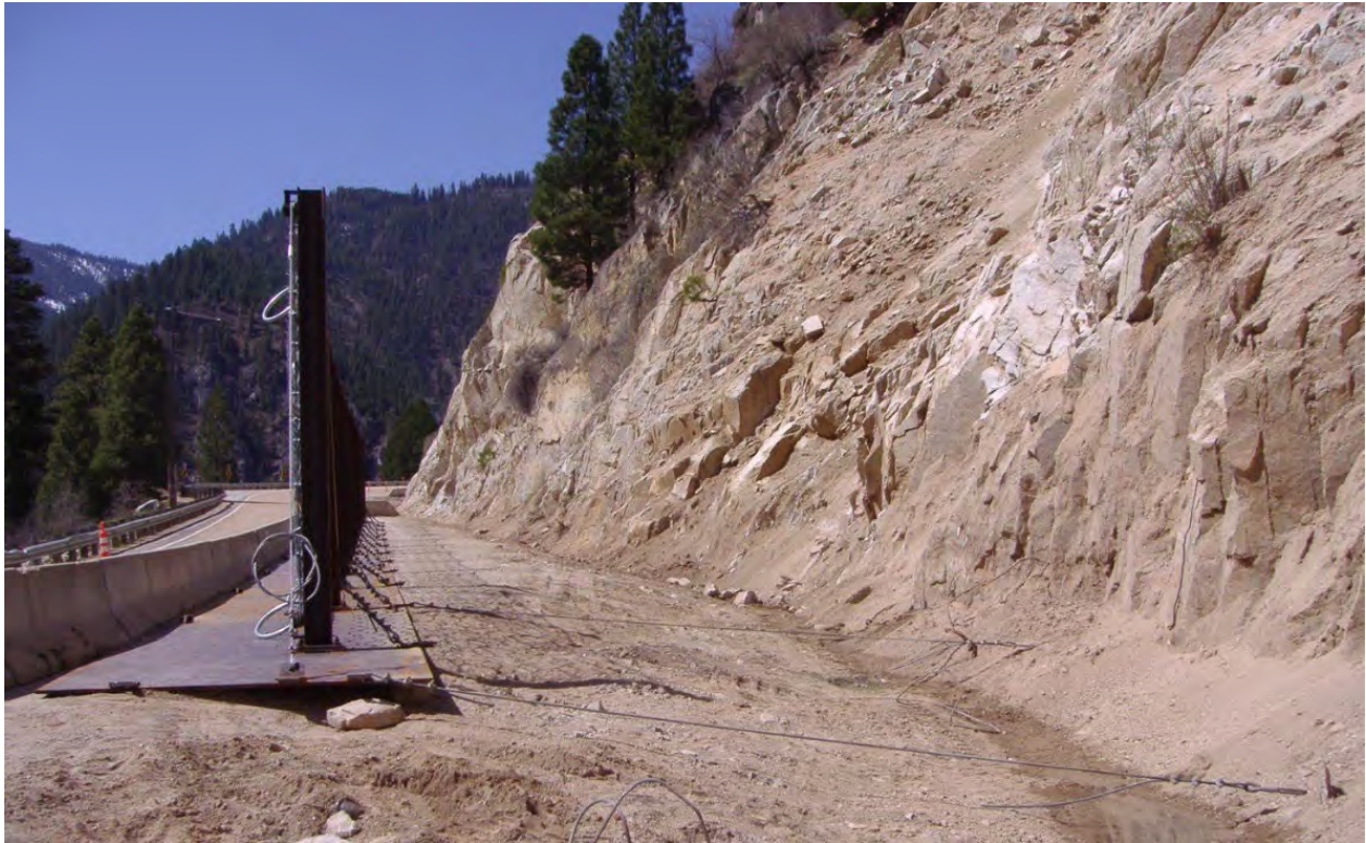
Figure 4-2 Typical Roadside, Movable Flexible Rockfall Fence (from WFLHD).
