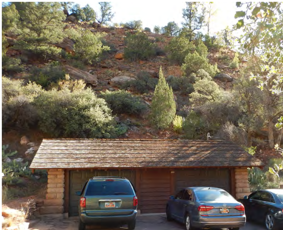
Figure 1435D: Photograph of slope above garage with unstable boulders.
