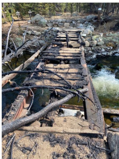
La Poudre Pass bridge post fire.
