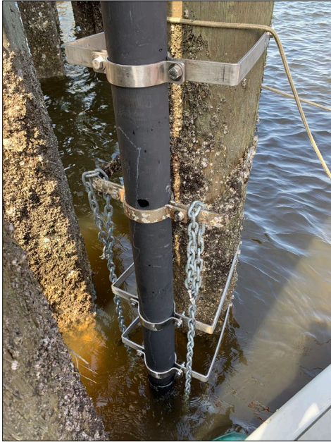
Figure 14. Sonde housing installed with multiple brackets and chain to prevent damage by extreme current velocity during incoming and outgoing tides.
