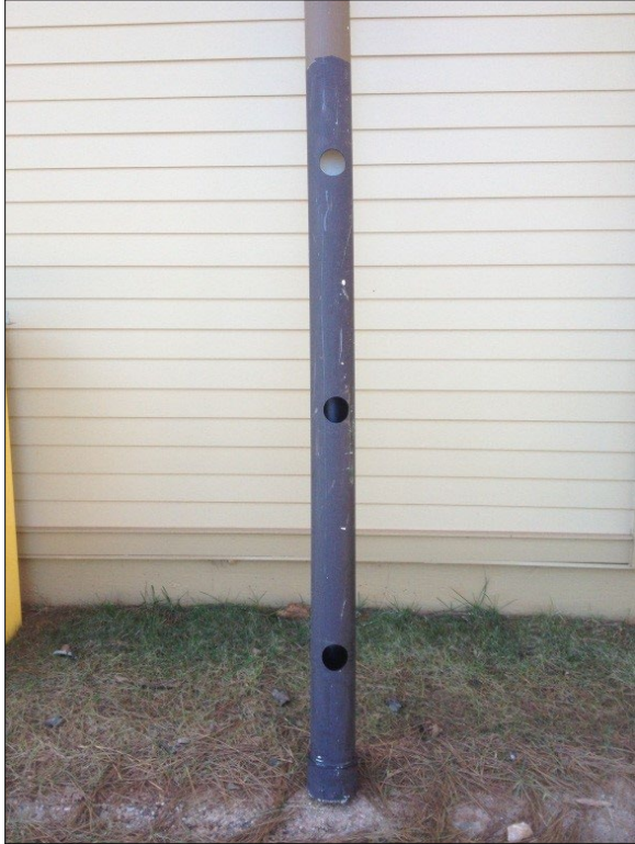
Figure 6. PVC pipe with drain holes.
