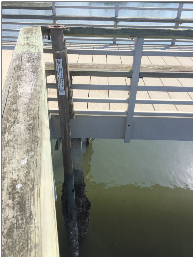
Figure 5. Stainless steel bands and bracket affixing a 4-inch (10.16 cm) schedule 40 PVC sonde housing to a pier at site FOPU1azz01.
