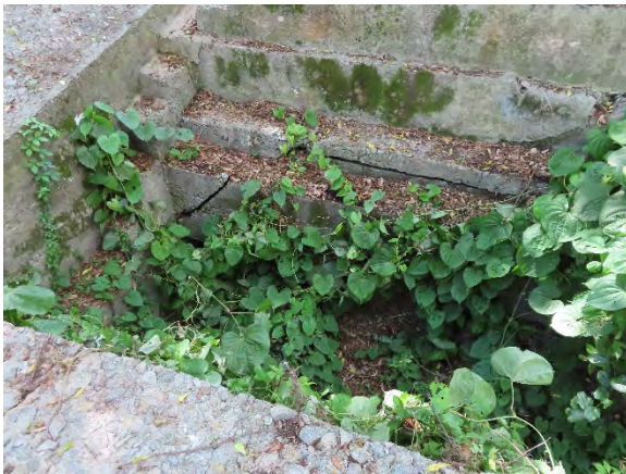
FIGURE 65. Organic growth present on the surface of the major pylon.
