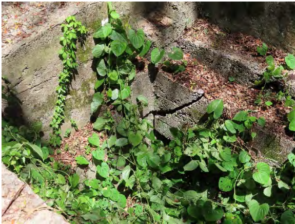
FIGURE 57. A crack observed in the base of the major pylon as seen from the roof of the magazine.
