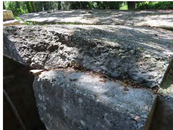
FIGURE 59. A large spall observed at the corner of the roof of the ramp leading to the magazine.
