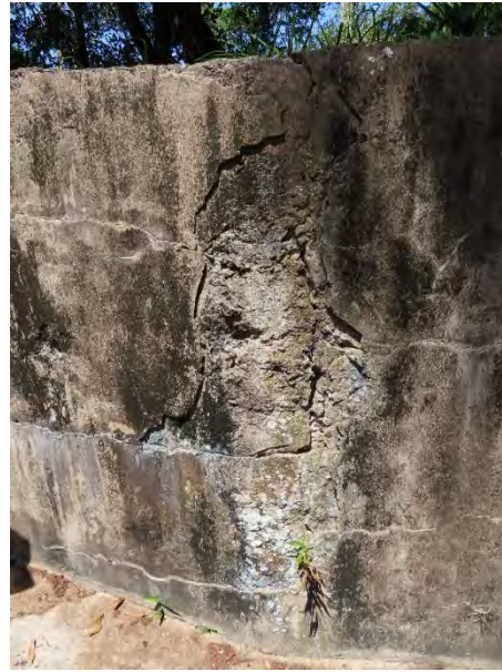
FIGURE 58. A large spall in the wall of the parapet.
