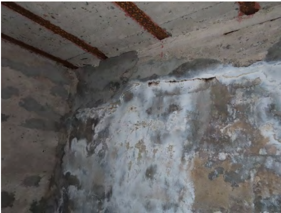
FIGURE 61. Efflorescence on the interior of the magazine. Corrosion of the exposed reinforcing in the ceiling is also visible.
