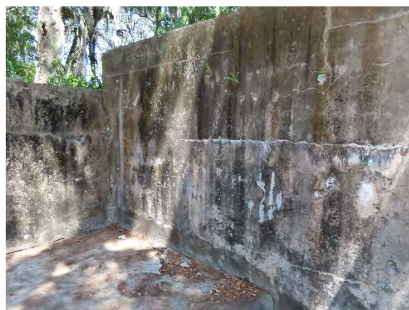
FIGURE 53. Horizontal cracks at cold joints in the traverse wall. Vertical cracking and efflorescence are also visible.
