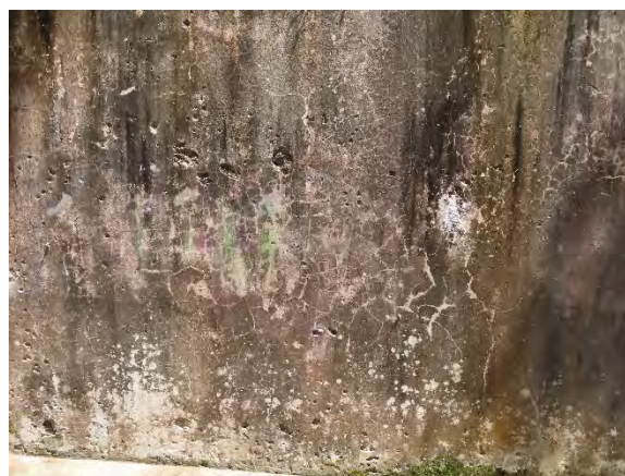
FIGURE 54. Map cracking in the traverse wall and efflorescence.
