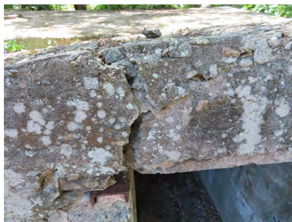
FIGURE 55. Cracks at the roof of the ramp leading to the magazine. Also visible is the corroded iron channel.
