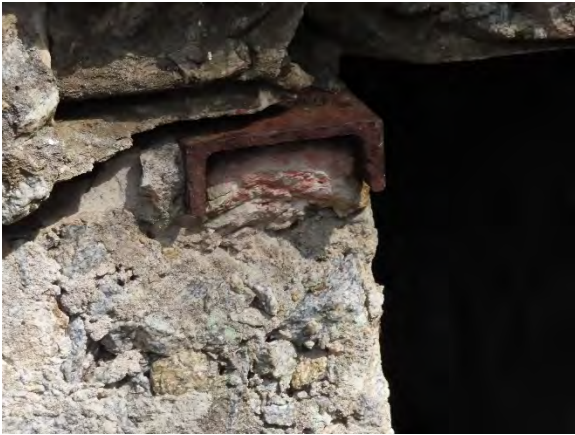
FIGURE 60. Corroded channel at the southwest side of the roof of the ramp to the magazine. Staining of the concrete is also visible beneath the channel.
