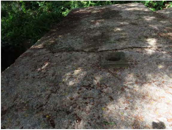
FIGURE 56. A large crack extending along the roof of the magazine. Also visible is the vent shaft located in the roof.
