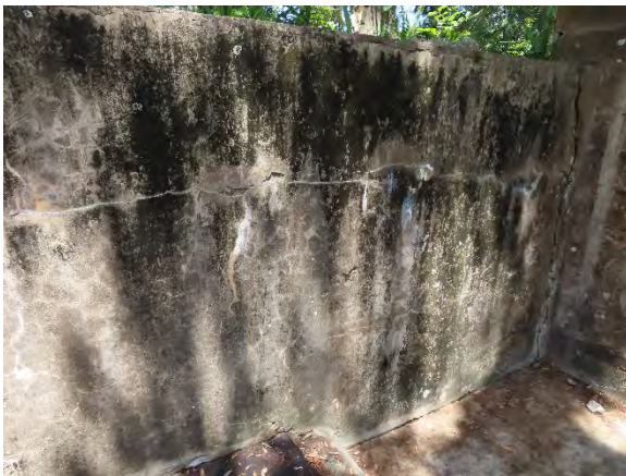
FIGURE 66. Darker organic growth on the parapet wall.
