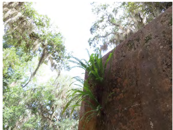
FIGURE 63. Vegetation growing through a crack in the traverse wall.
