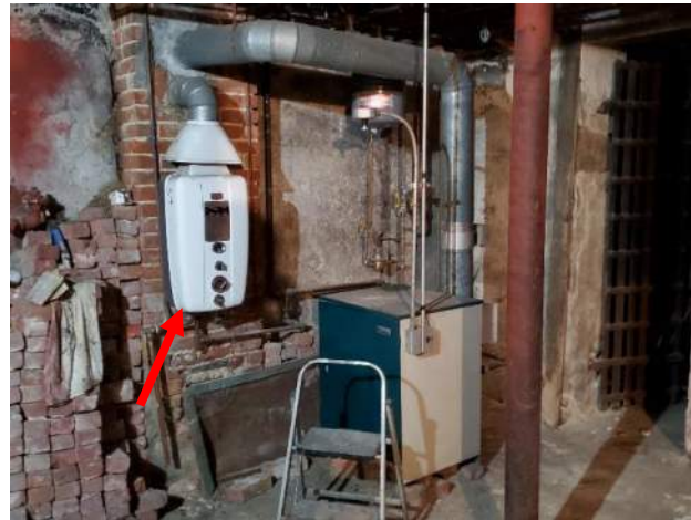
Figure 3.83: Water heater and boiler.
