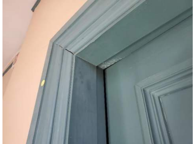
Figure 3.56: Door 2-2 doesn't close.
