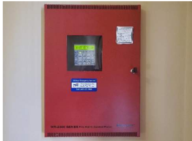
Figure 3.86: Fire Alarm Panel.
