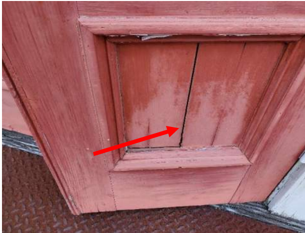
Figure 3.28: South, Back Door – Cracked panel.
