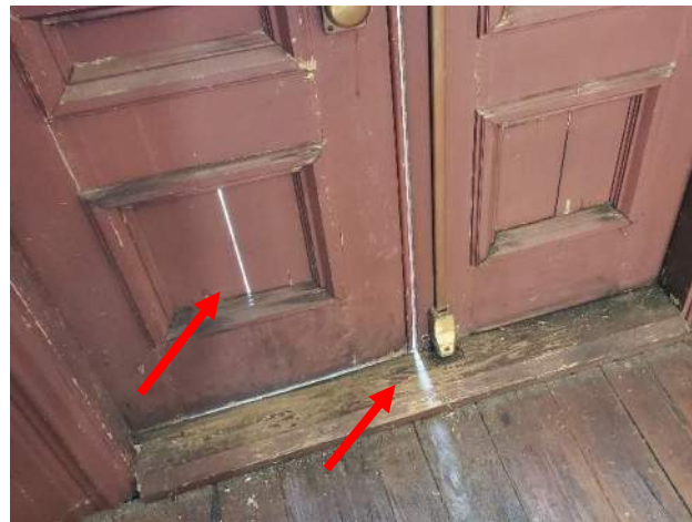
Figure 3.31: South, Back Door – Open joints.
