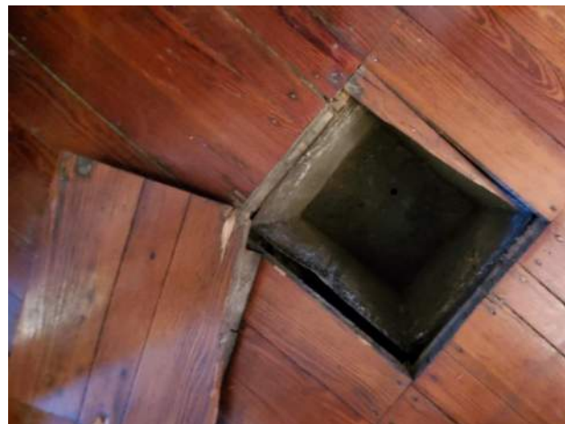
Figure 3.75: Hidden floor box.
