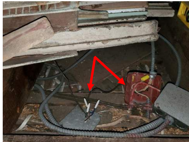
Figure 3.50: Exposed wire connections.
