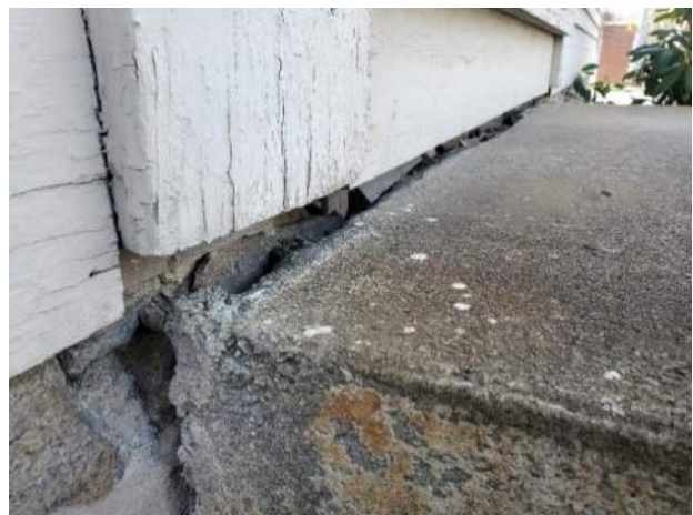
Figure 3.42: Gaps behind front stairs.
