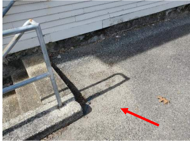
Figure 3.7: Ponding north of basement stair.
