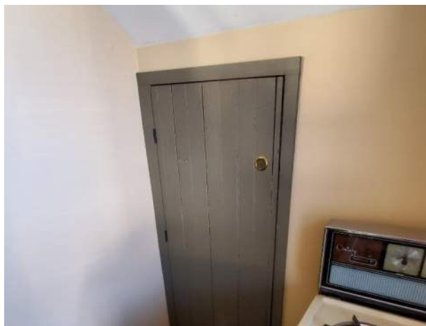
Figure 3.71: Door behind the refrigerator.
