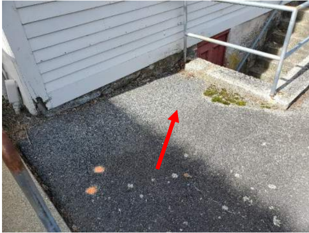
Figure 3.6: Ponding south of basement stair.
