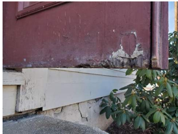
Figure 3.27: North, Front Door – Rot.
