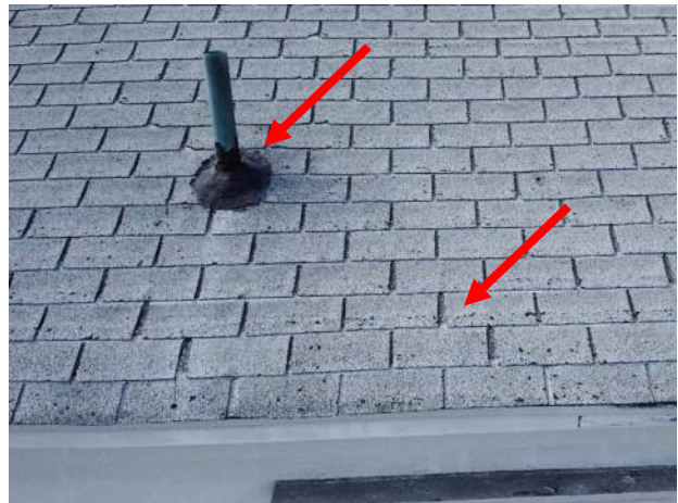
Figure 3.15: Worn shingles and plumbing vent.
