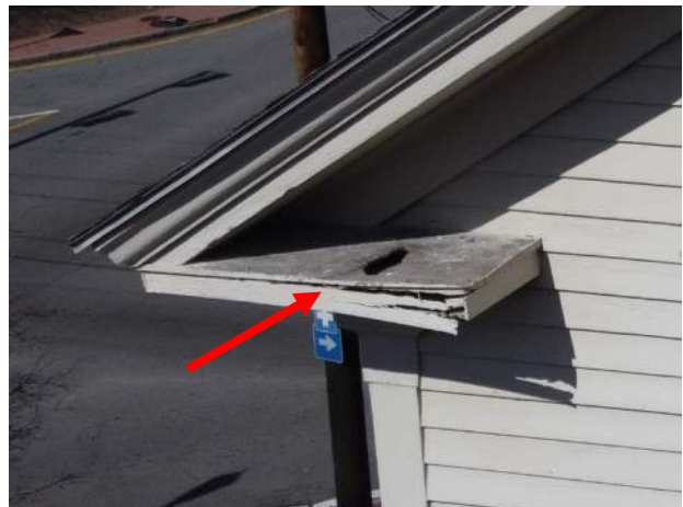
Figure 3.17: Hole in Cornice Return.
