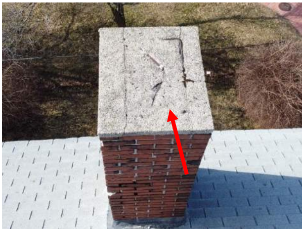
Figure 3.16: Worn chimney cap.
