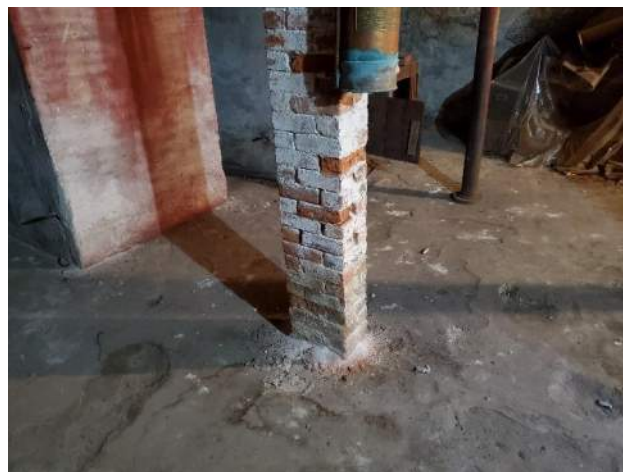
Figure 3.79: Deteriorating brick column.
