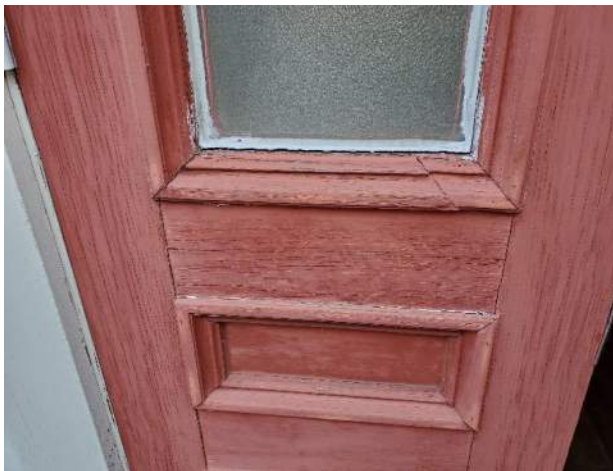
Figure 3.30: South, Back Door – Weathered paint.
