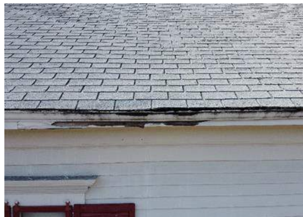
Figure 3.12: Deteriorating roof edge.
