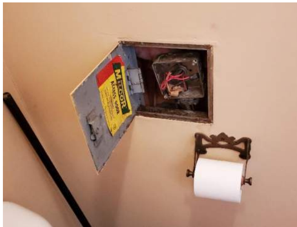
Figure 3.88: Junction box in first floor toilet room.
