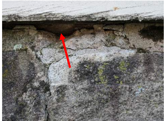
Figure 3.44: The sill plate is exposed in areas.
