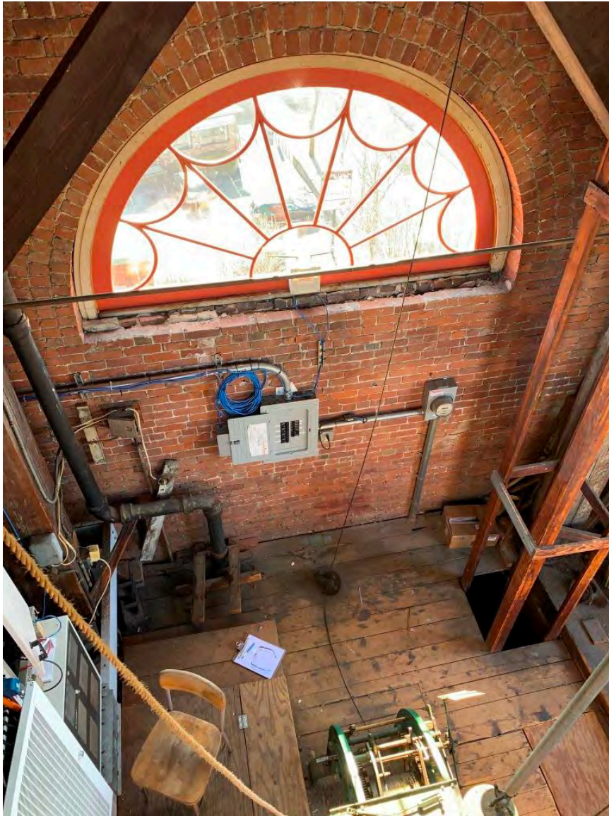
Cumberland Town Hall – Interior – Historic Finishes and Building Elements Tower – Overall View Looking Down to Fifth Floor Window Sill Missing Revealing Back-up Masonry
