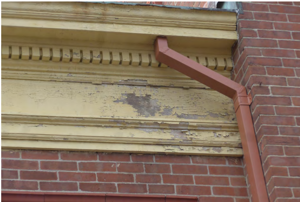
Cumberland Town Hall – Exterior – Wood Elements East Elevation – Above Entrance Porch Worn/Peeling Paint
