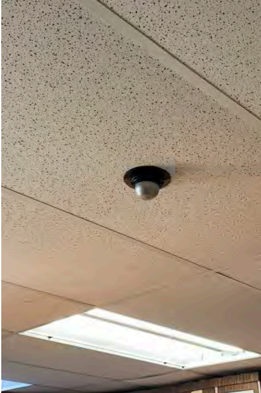
Cumberland Town Hall - Code Compliance Conditions Basement – Storage Room Existing Fire Sensor
