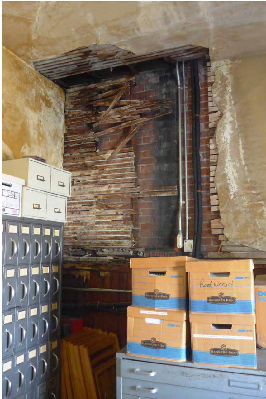
Cumberland Town Hall – Interior – Plaster Walls and Ceilings - Storage Third Floor – East Storage Area Severe Unrepaired Damage from Previous Leak; Excessive Storage Creating Substantial Load
