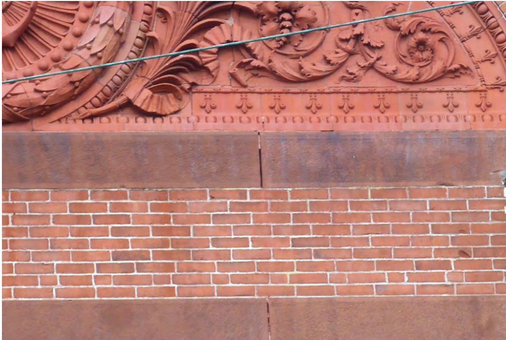
Cumberland Town Hall – Exterior - Masonry South Elevation – Central Pavilion – Second Floor (Currently Attic Level) - Detail Open Joints, Staining
