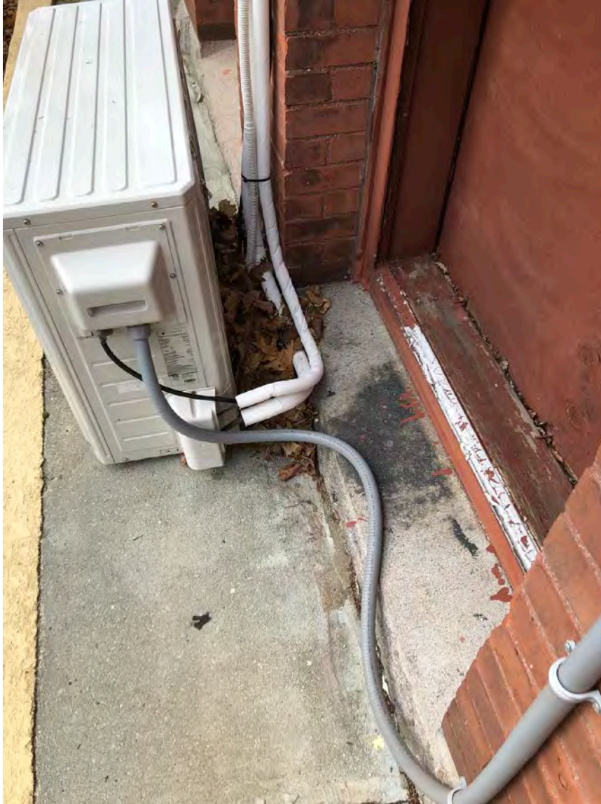
Cumberland Town Hall – Exterior – Landscaping Elements South Elevation – Concrete Pavement adjacent to Building Accumulate Debris behind AC Compressor
