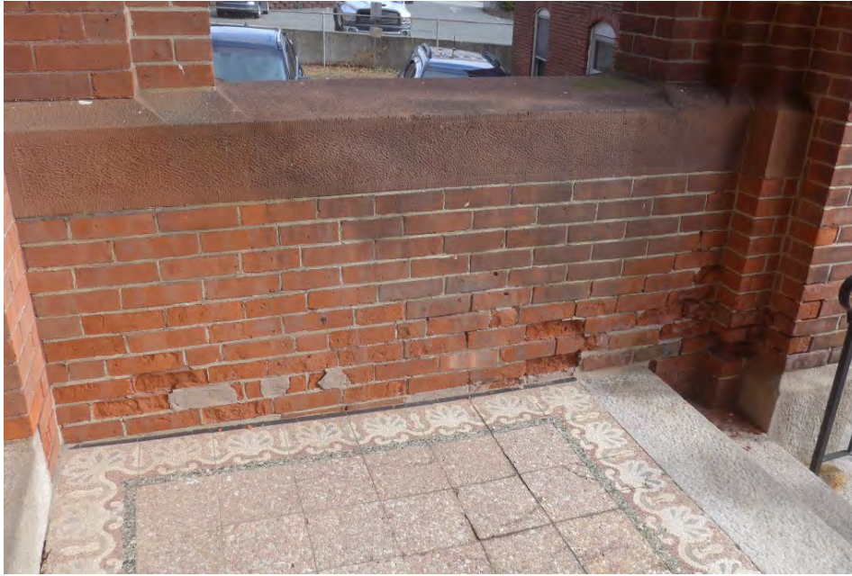
Cumberland Town Hall – Exterior - Masonry Southeast Corner – Entrance Porch Open Joints, Deteriorated/Missing Brickwork; Staining
