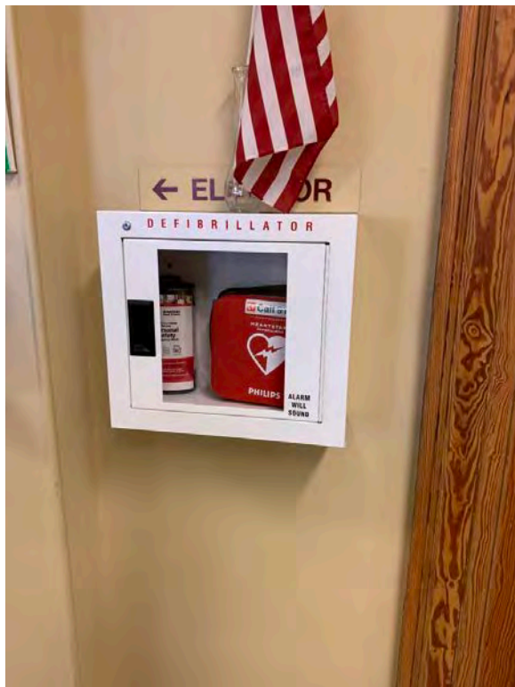
Cumberland Town Hall - Code Compliance Conditions First Floor - Main Hallway Left: Fire Alarm and Smoke Sensor; Right: Defibrillator
