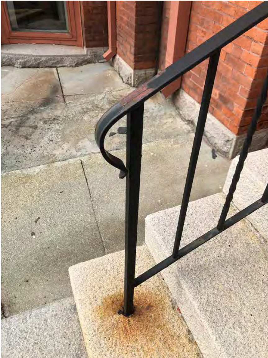
Cumberland Town Hall – Exterior – Metal Elements South Elevation – Entrance at Southeast Corner Worn Paint; Rusting; Staining Granite Steps
