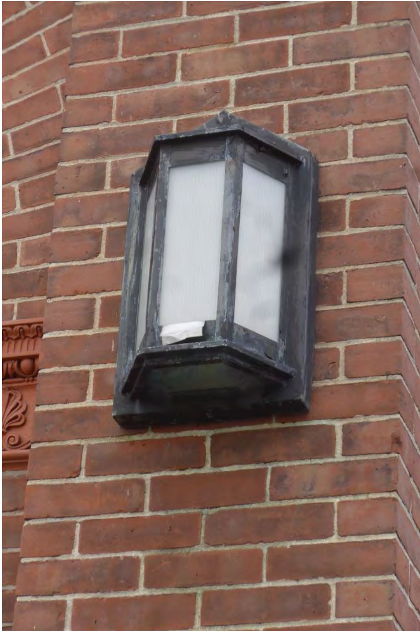
Cumberland Town Hall – Exterior – Historic Finishes and Building Elements West Elevation – at Main, West Entrance Historic Light Fixture In Fair Condition
