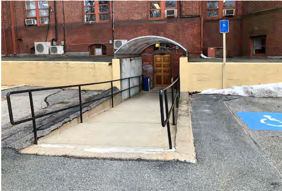
Cumberland Town Hall – Accessibility Conditions West Entrance at Porte Cochere Handicapped Parking and Code Compliant Ramp Provided
