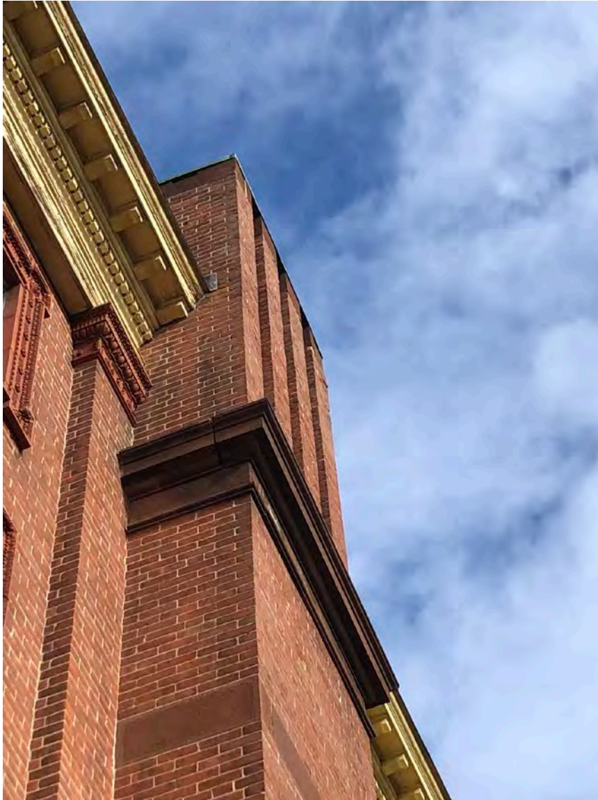
Cumberland Town Hall – Exterior - Masonry South Elevation – Chimney Top of Chimney has been Removed
