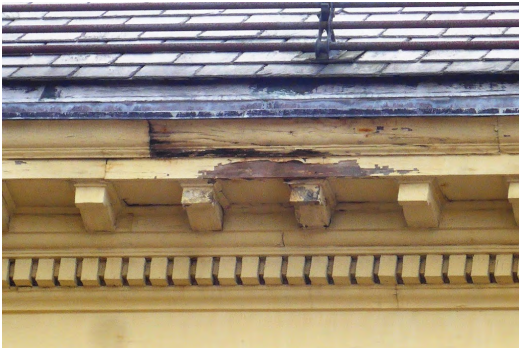
Cumberland Town Hall – Exterior – Wood Elements North Elevation – Central Pavilion – Cornice - Detail Worn/Peeling Paint; Deteriorated Wood Elements
