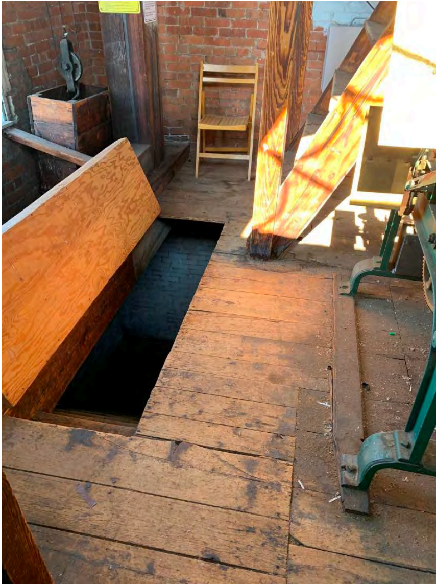
Cumberland Town Hall – Interior – Code Compliance Tower – Fifth Floor Open Stair Hatch with No Railing
