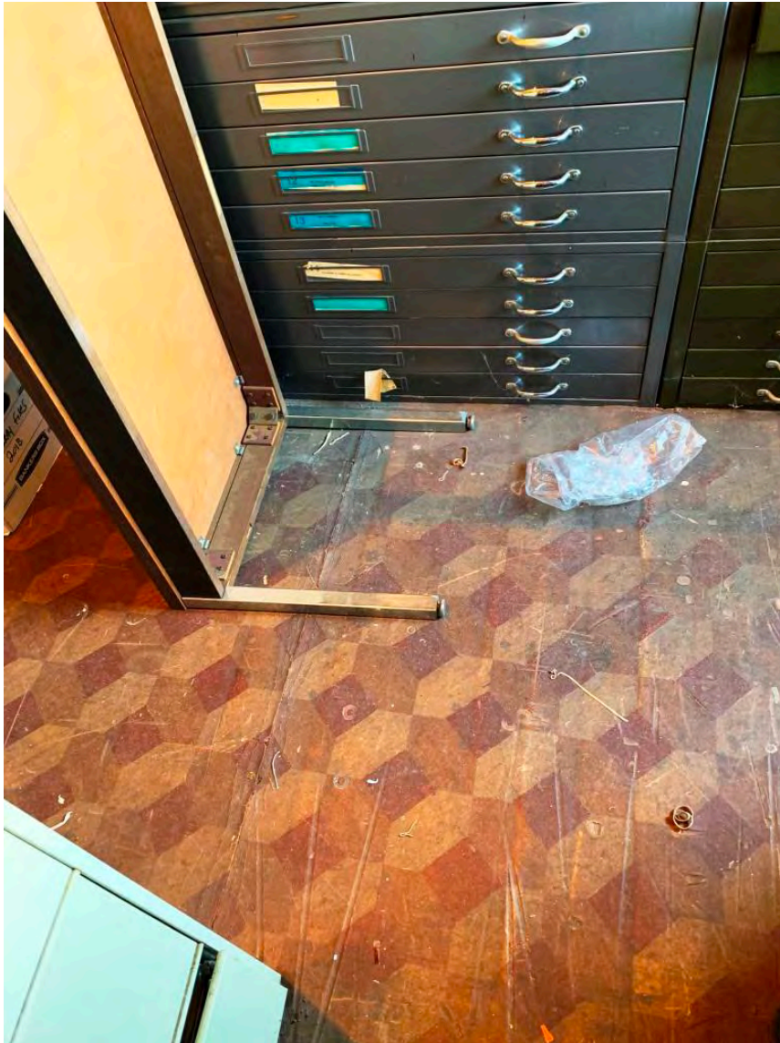
Cumberland Town Hall – Interior – Historic Finishes and Elements - Storage Third Floor – Southwest Corner Room 1930s-era Inlaid Wood Floor Damaged from Storage-related Abuse Excessive Storage Creating Substantial Load
