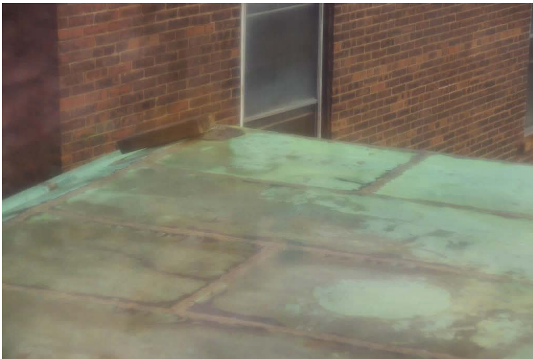
Cumberland Town Hall – Roofing, Flashing, Gutters, Leaders, Metal Trim and Roofing Elements Roof Above Southeast Entrance Porch - Detail Metal Roof in Good Condition Overall; Metal Lifting at Corner
