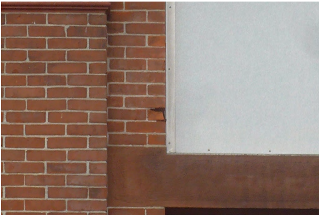
Cumberland Town Hall – Exterior - Masonry South Elevation – Central Pavilion - Third Floor (Currently Attic Level) - Detail Damaged Brick
