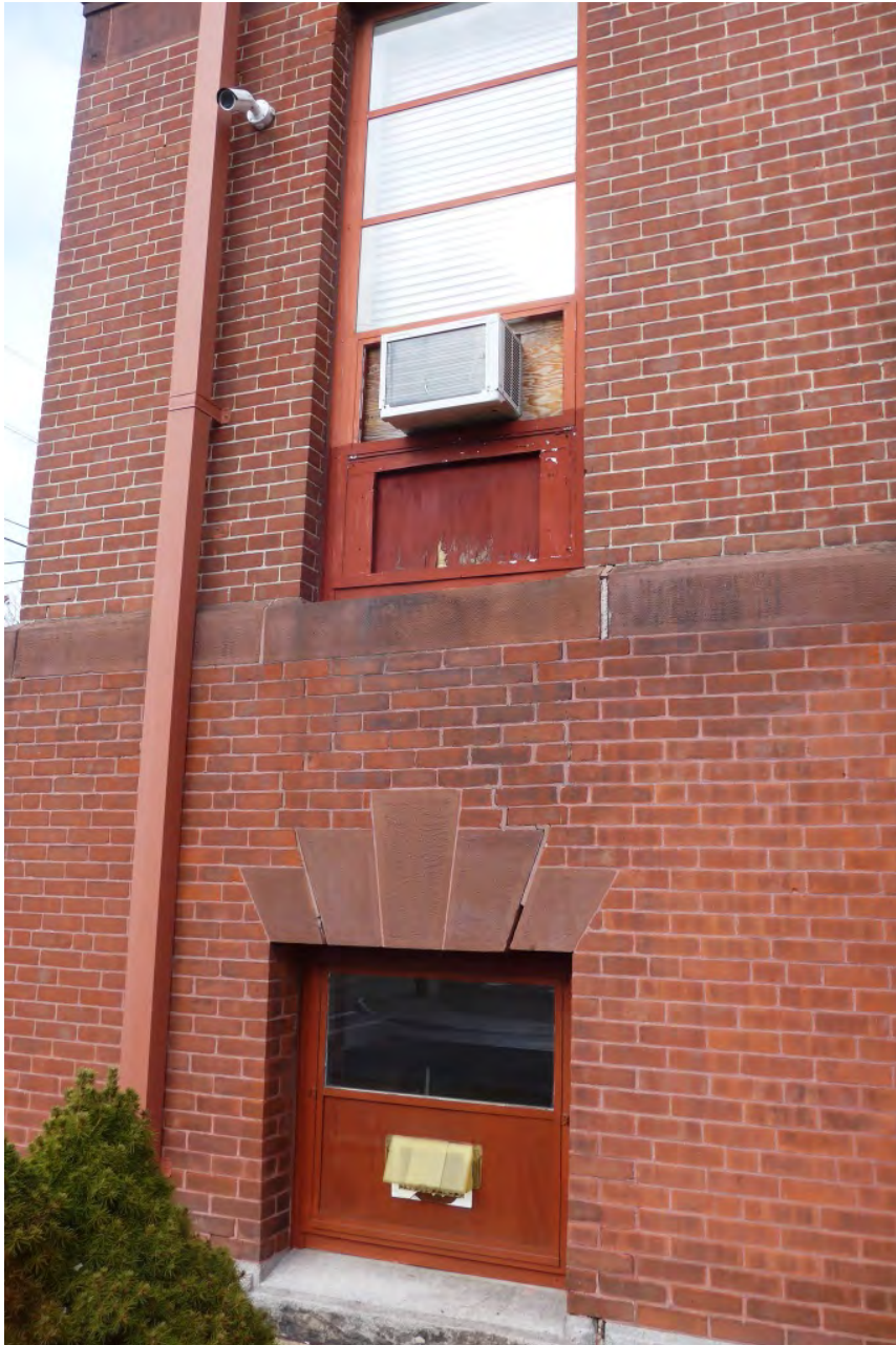
Cumberland Town Hall – Exterior - Masonry South Elevation – West Pavilion – West Bay - Basement Level/First Floor Open Joints, Staining
