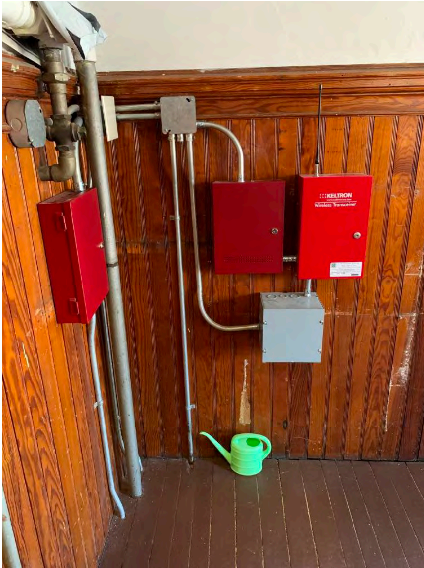
Cumberland Town Hall - Code Compliance Conditions First Floor – Landing at Top of Main Basement Stair Fire Alarm System
