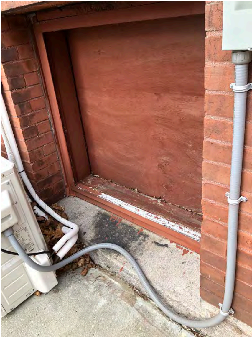
Cumberland Town Hall – Exterior - Windows, Doors and Hardware South Elevation – Basement Level Window Removed and Replaced with Plywood
