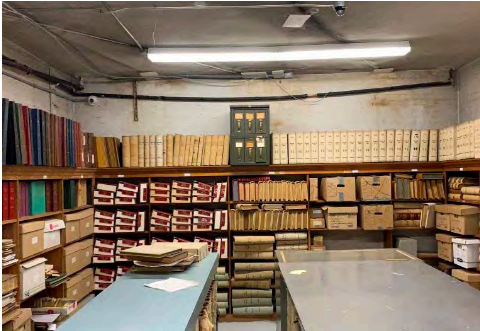
Cumberland Town Hall – Interior - Overall Basement – Vault under West Entrance Stair Typical Conditions – Fair Overall – Moisture Issues at Upper Portion of Walls and Ceiling
