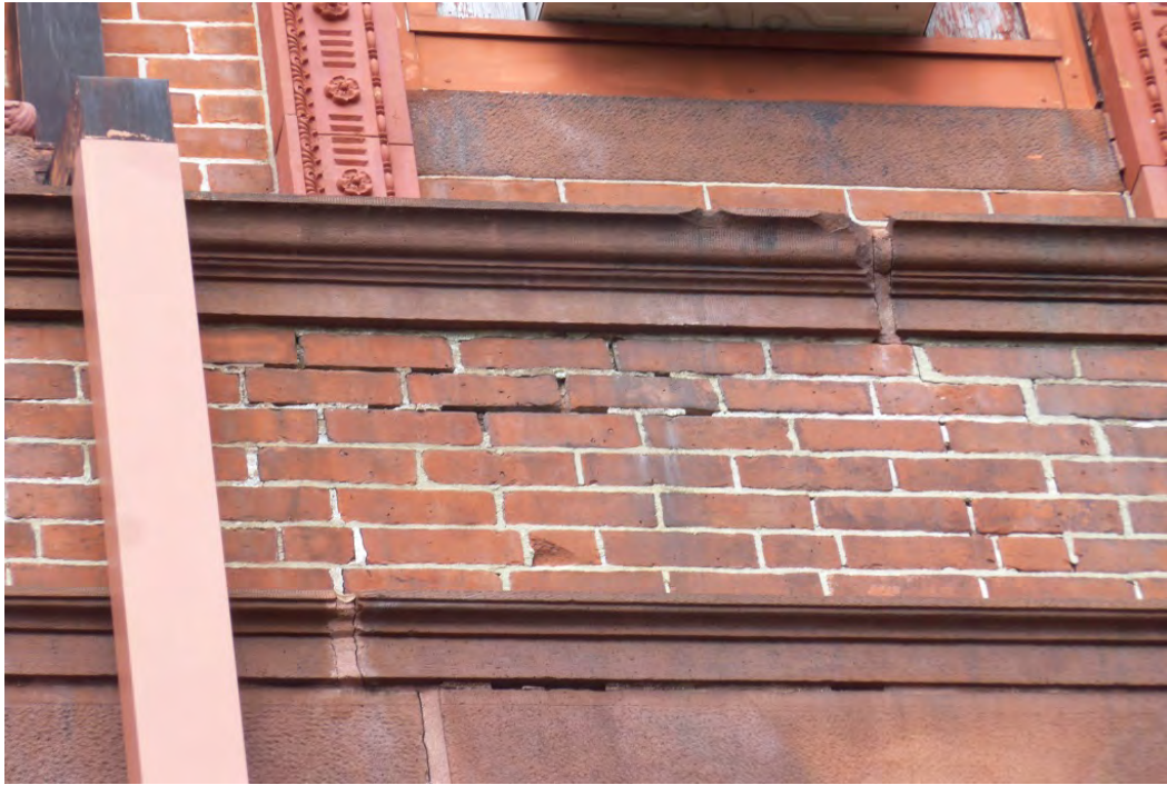
Cumberland Town Hall – Exterior - Masonry South Elevation – West Pavilion – West Bay - Second Floor Open Joints, Cracked and Missing Brownstone, Staining
