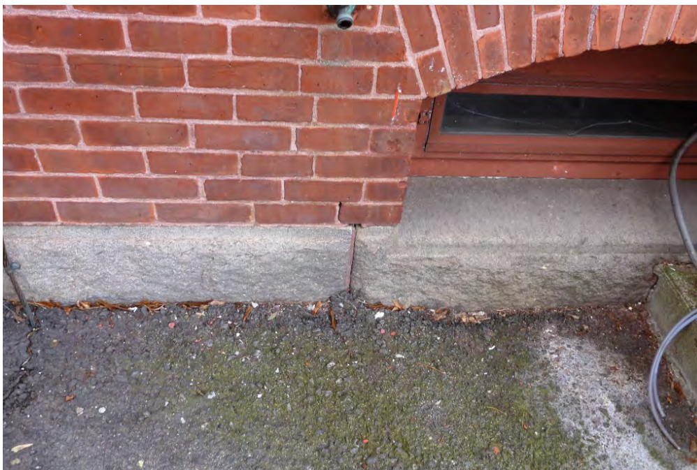
Cumberland Town Hall – Exterior - Masonry North Elevation – Base of Building Open Joints in Masonry
