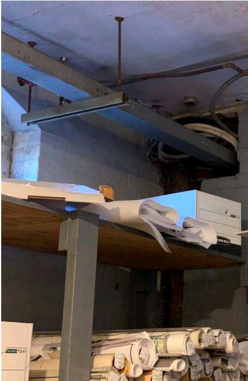
Cumberland Town Hall – Interior - Overall Basement – Storage Area Off Boiler Room Unsealed Penetrations; Papers Stored Inappropriately in Mechanical Areas
