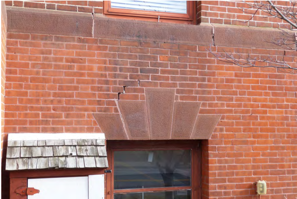
Cumberland Town Hall – Exterior - Masonry West Elevation – South Pavilion – North Window - Basement Level Open Joints, Step Crack
