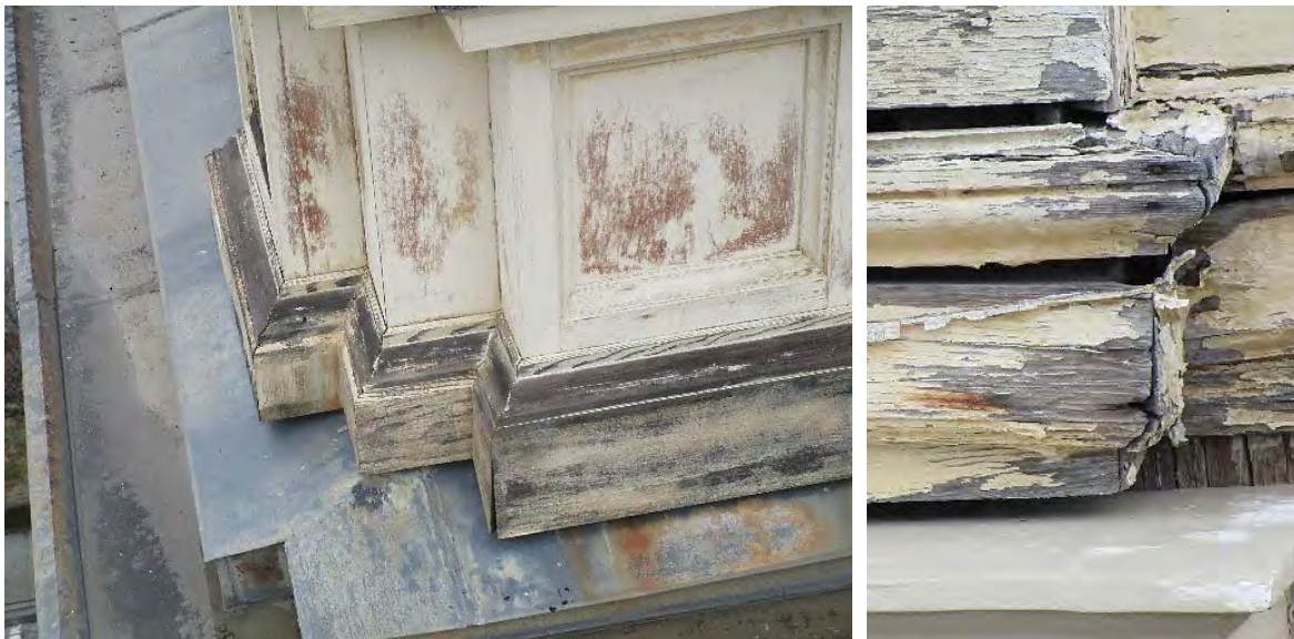
Cumberland Town Hall – Exterior – Wood Elements Tower – Lower Balustrade at Clock Level (Sixth Floor) Flaking and Deteriorated Paint – Some Deteriorated Wood Source: Town of Cumberland
