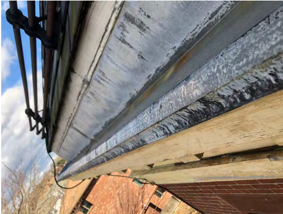
Cumberland Town Hall – Roofing, Flashing, Gutters, Leaders, Metal Trim and Roofing Elements North Elevation – Above Elevator Addition – Gutter built into Cornice Gutter too Shallow to Facilitate Lengthy Distance to Downspout
