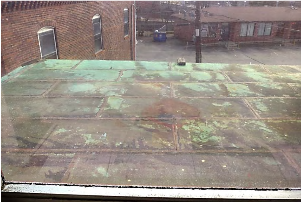
Cumberland Town Hall – Roofing, Flashing, Gutters, Leaders, Metal Trim and Roofing Elements Roof Above Southeast Entrance Porch Metal Roof in Good Condition Overall; Metal Lifting at Corner
