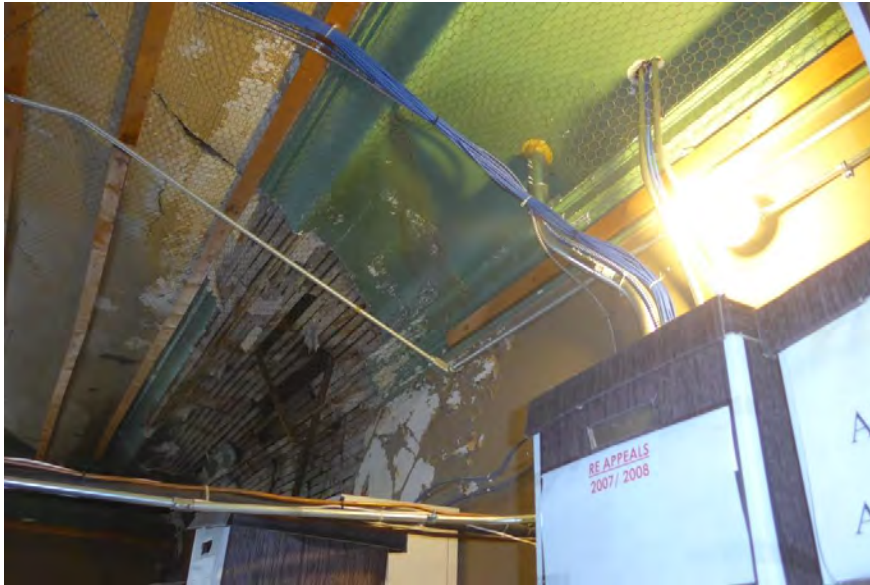
Cumberland Town Hall – Interior – Historic Finishes and Details – Plaster Walls and Ceilings Third Floor – Original Upper Assembly Hall Damaged Plaster Trim from Building Alterations; Unrepaired Damage to Plaster Walls, Ceiling, and Trim from Previous Leaks
