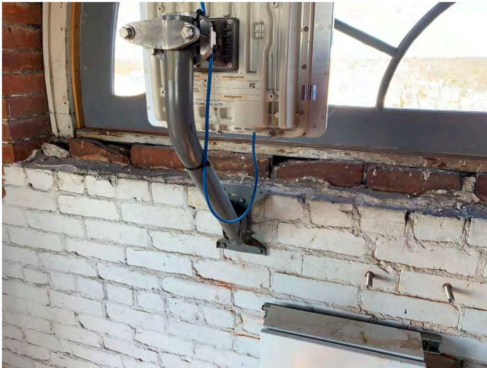
Cumberland Town Hall – Interior – Historic Finishes and Elements Tower Damaged Masonry
