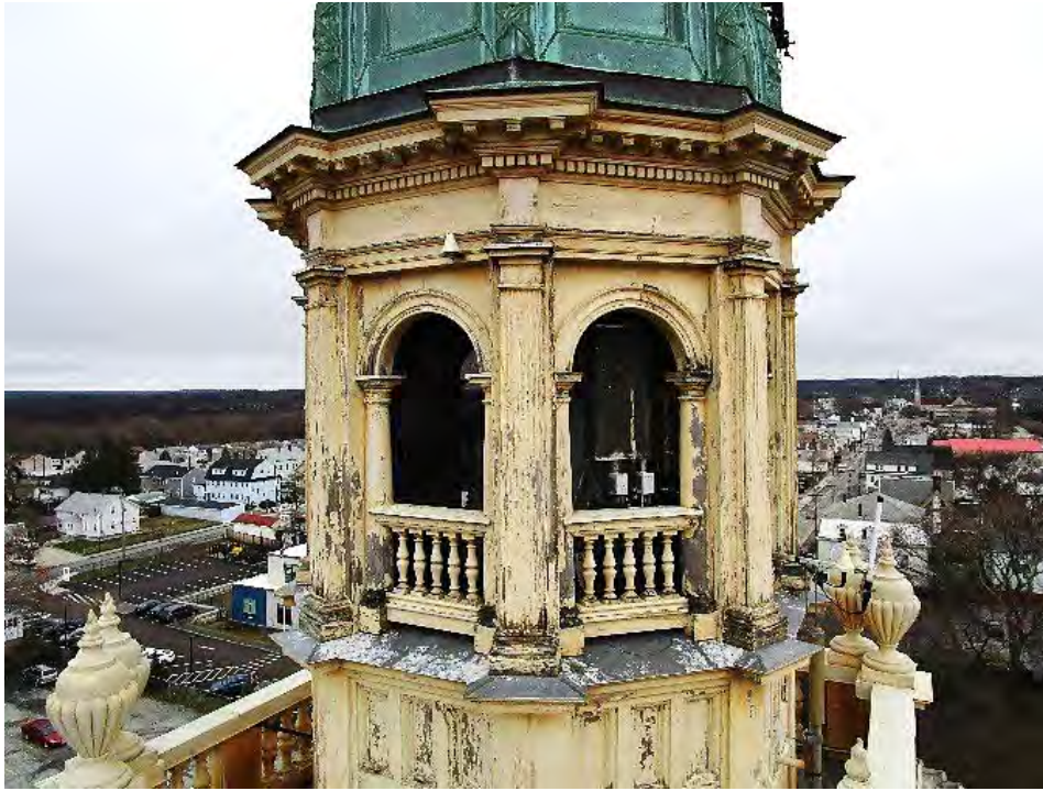
Cumberland Town Hall – Exterior – Wood Elements Tower – Cupola at Bell Level Flaking and Deteriorated Paint – Some Deteriorated Wood Source: Town of Cumberland
