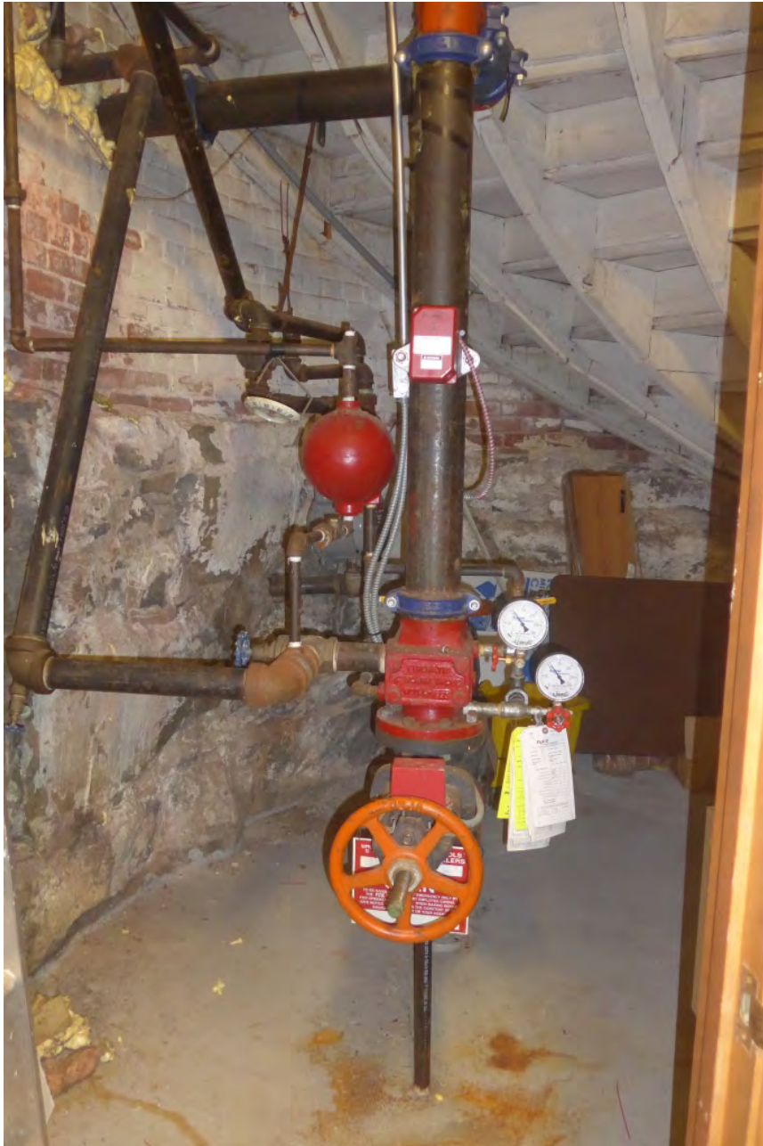
Cumberland Town Hall - Code Compliance Conditions - First Floor Basement – Under Main Stair Sprinkler System Pump
