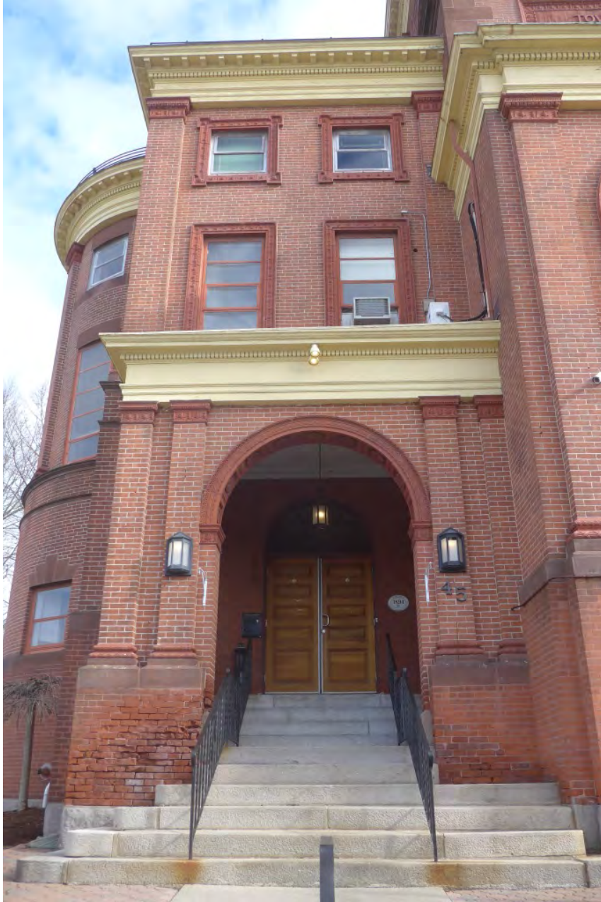
Cumberland Town Hall – Exterior - Masonry West Elevation – North Pavilion - Entrance - Overall Open Joints, Eroded Brickwork
