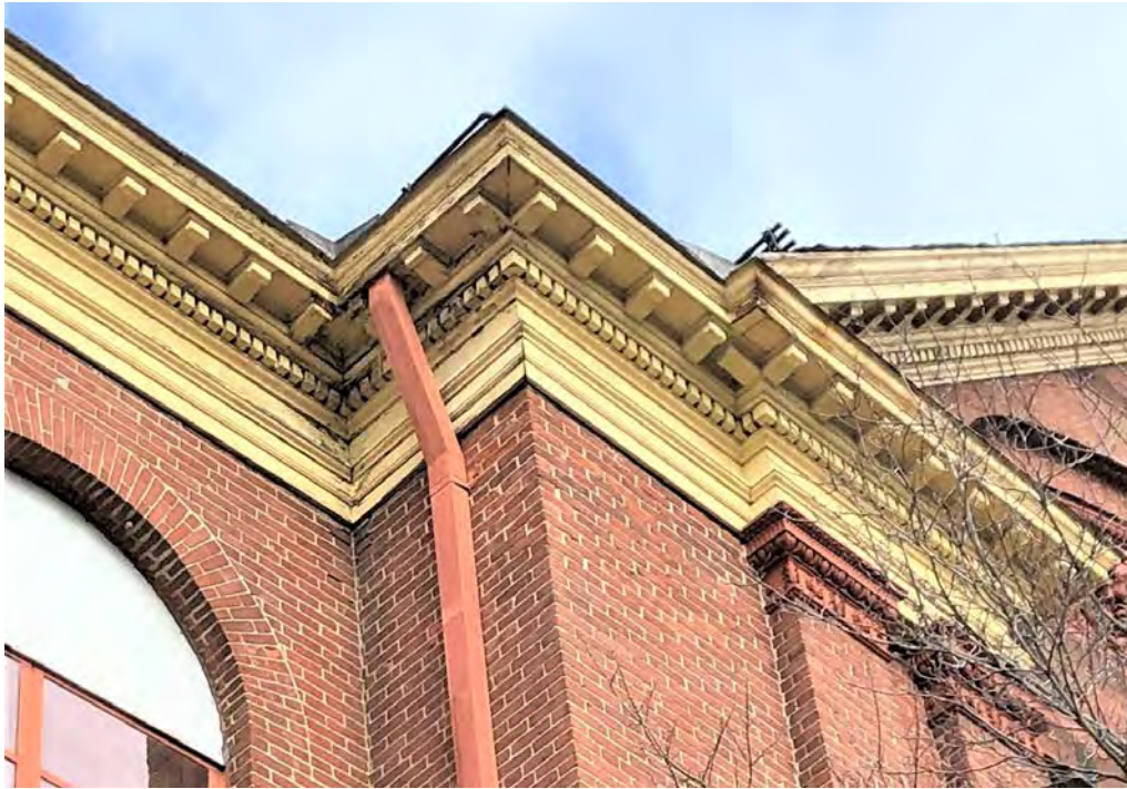
Cumberland Town Hall – Exterior – Wood Elements South Elevation – Return Between West and Central Pavilion - Cornice Worn/Peeling Paint; Deteriorated Wood Elements
