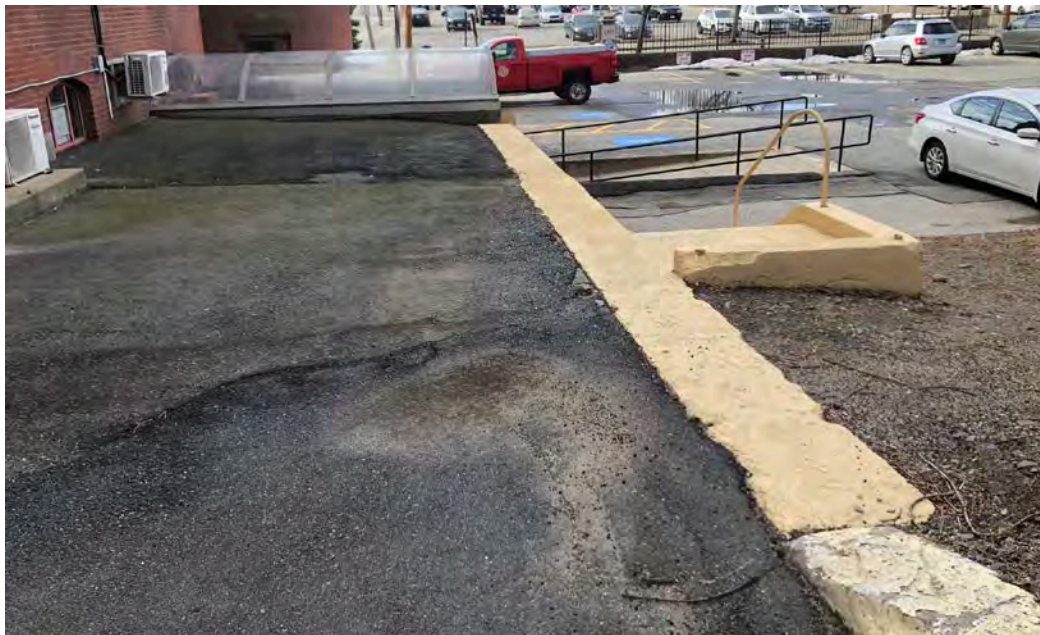
Cumberland Town Hall - Code Compliance Conditions North Raised Area No Railing along Raised Asphalt Area; Missing Railing at Stair
