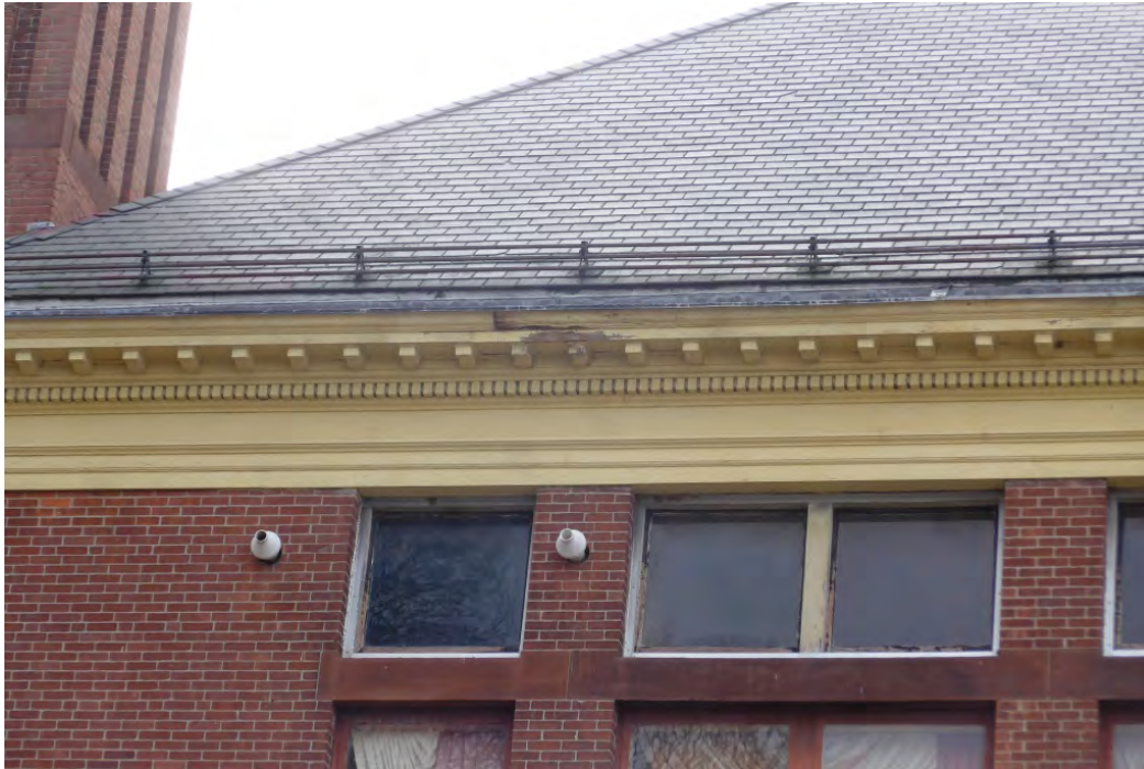
Cumberland Town Hall – Exterior – Wood Elements North Elevation – Central Pavilion - Cornice Worn/Peeling Paint; Deteriorated Wood Elements
