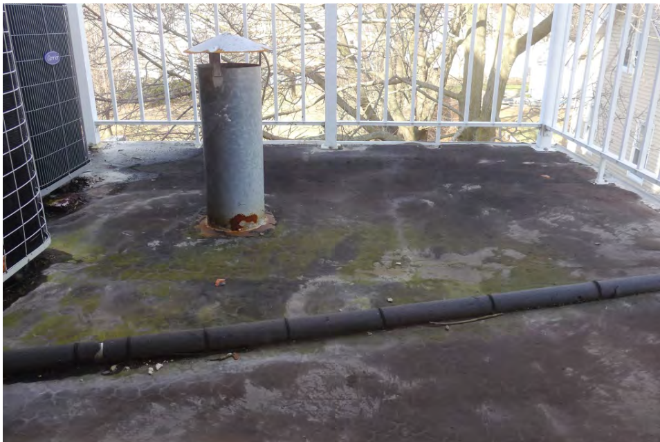
Cumberland Town Hall – Roofing, Flashing, Gutters, Leaders, Metal Trim and Roofing Elements Roof Above Elevator Addition Rubber Membrane Roof Stained and in Poor Condition; Rusting Metal Vent
