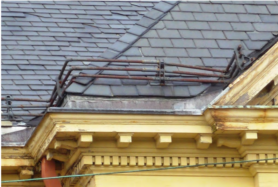
Cumberland Town Hall – Roofing, Flashing, Gutters, Leaders, Metal Trim and Roofing Elements South Elevation – West Corner of Central Pavilion Damaged Snow Guard Piping; Cracked Slates
