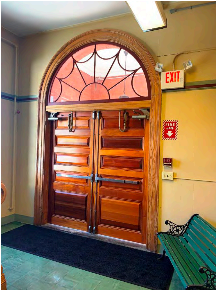
Cumberland Town Hall - Code Compliance Conditions First Floor – East Entrance/Stair Hall at Southeast Entrance Emergency Exit Panic Hardware, Signage, Emergency Lighting and Fire Pull Box
