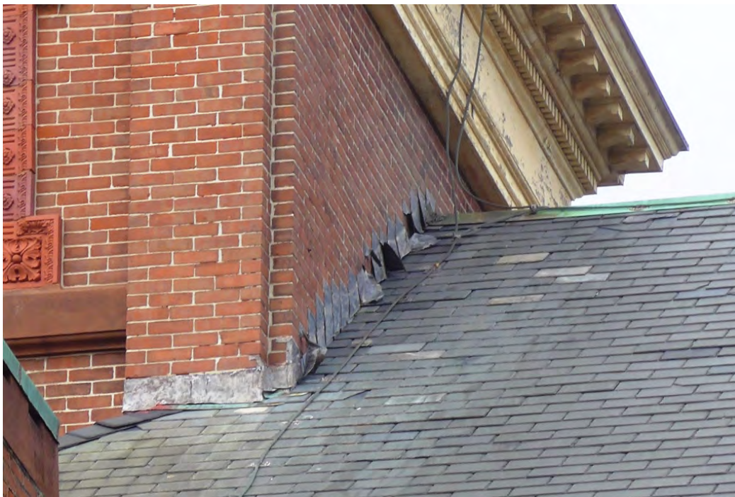
Cumberland Town Hall – Roofing, Flashing, Gutters, Leaders, Metal Trim and Roofing Elements Base of Tower at East Elevation Lifting and Damaged Step Flashing and Cracked Slates
