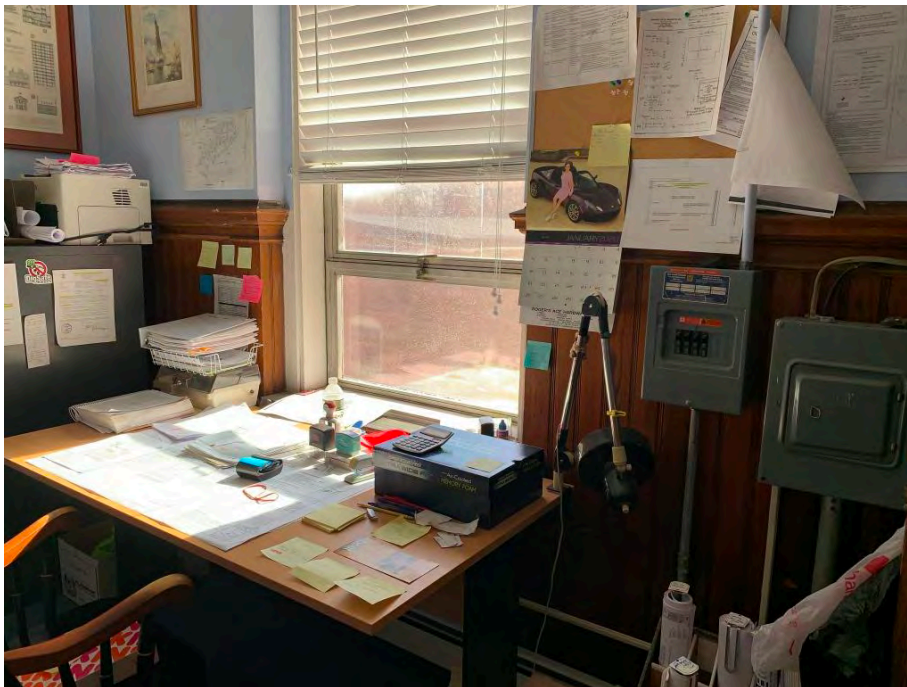
Cumberland Town Hall – Interior - Code Compliance
