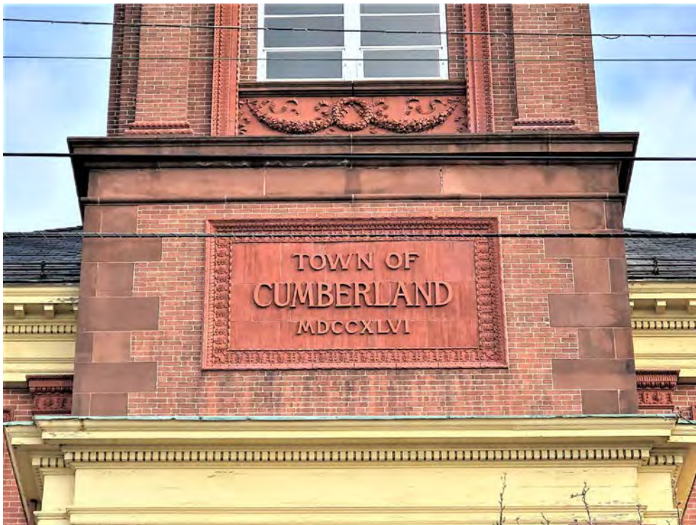
Cumberland Town Hall – Exterior – Masonry – Exterior Woodwork West Elevation – Central Pavilion - Tower Good Condition; Some Staining; Peeling Paint on Woodwork
