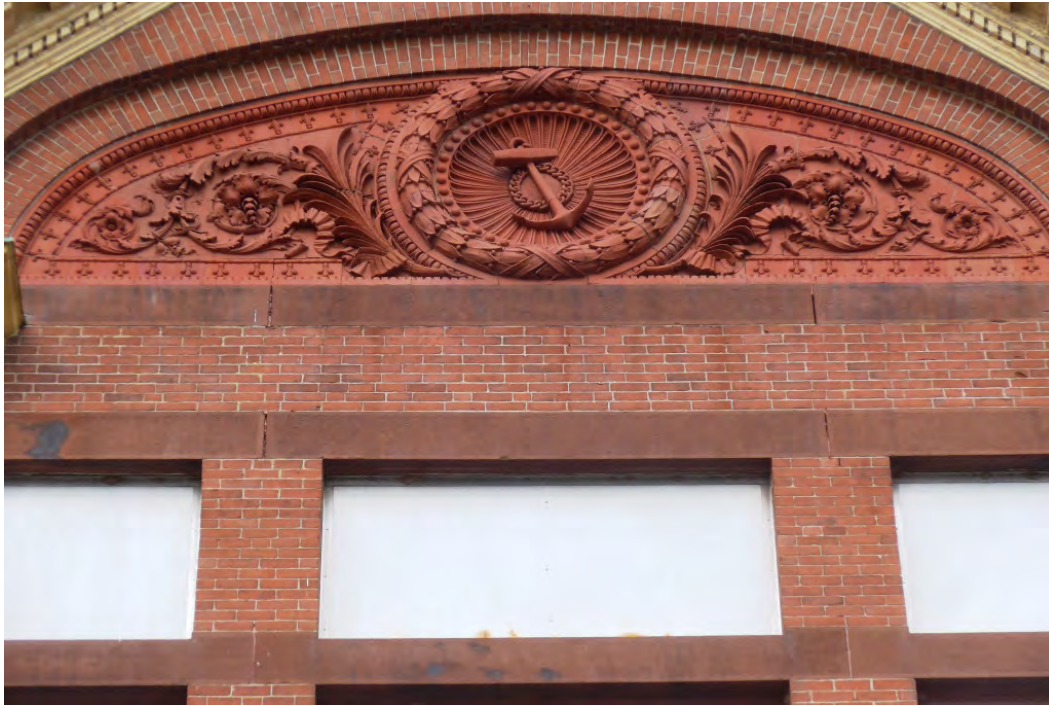
Cumberland Town Hall – Exterior - Masonry South Elevation – Central Pavilion – Third Floor (Currently Attic Level) Open Joints, Staining
