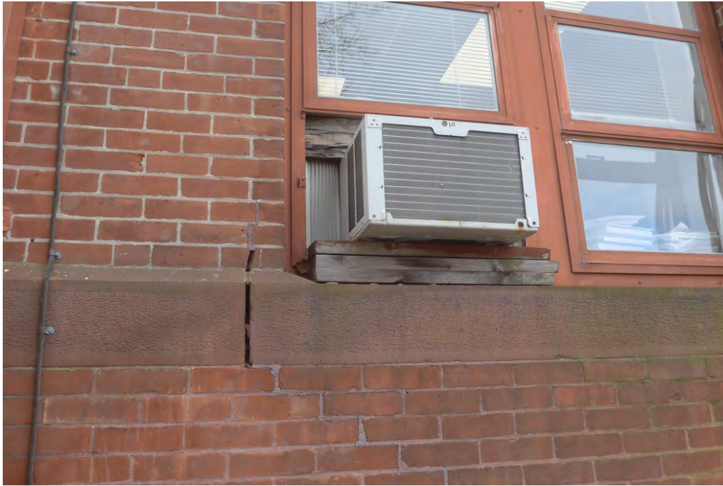
Cumberland Town Hall – Exterior - Masonry North Elevation – Central Pavilion – East Window Open Joints in Masonry
