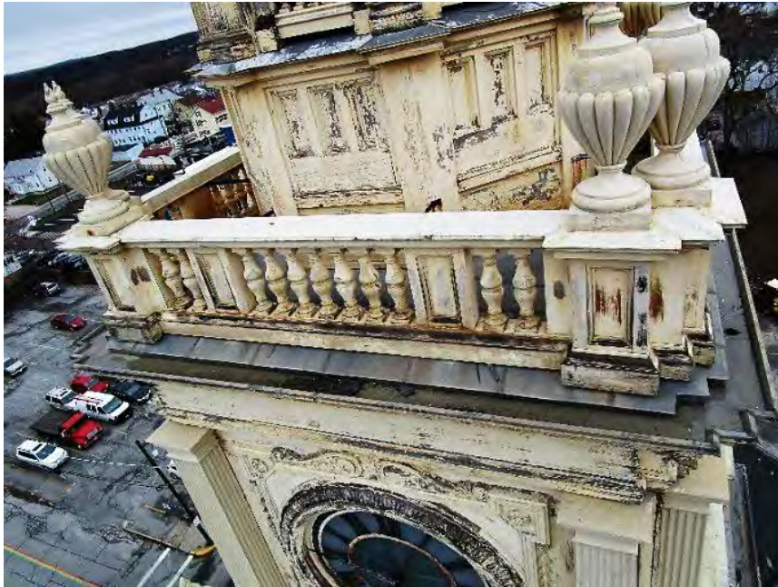
Cumberland Town Hall – Exterior – Wood Elements Tower – Base of Cupola and Upper Balustrade Flaking and Deteriorated Paint – Some Deteriorated Wood Source: Town of Cumberland
