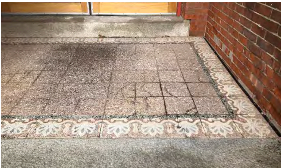
Cumberland Town Hall – Exterior - Masonry Southeast Corner – Entrance Porch Open Joints, Cracked & Deteriorated Pavers; Staining
