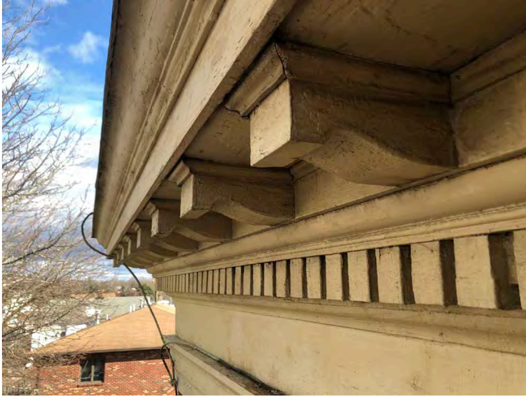
Cumberland Town Hall – Exterior – Wood Elements North Elevation – above Elevator Addition Worn Paint; Wood in Good Condition
