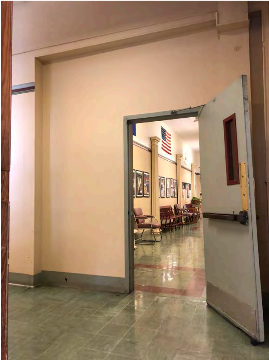
Cumberland Town Hall – Interior - Historic Finishes and Building Elements – Code Compliance
