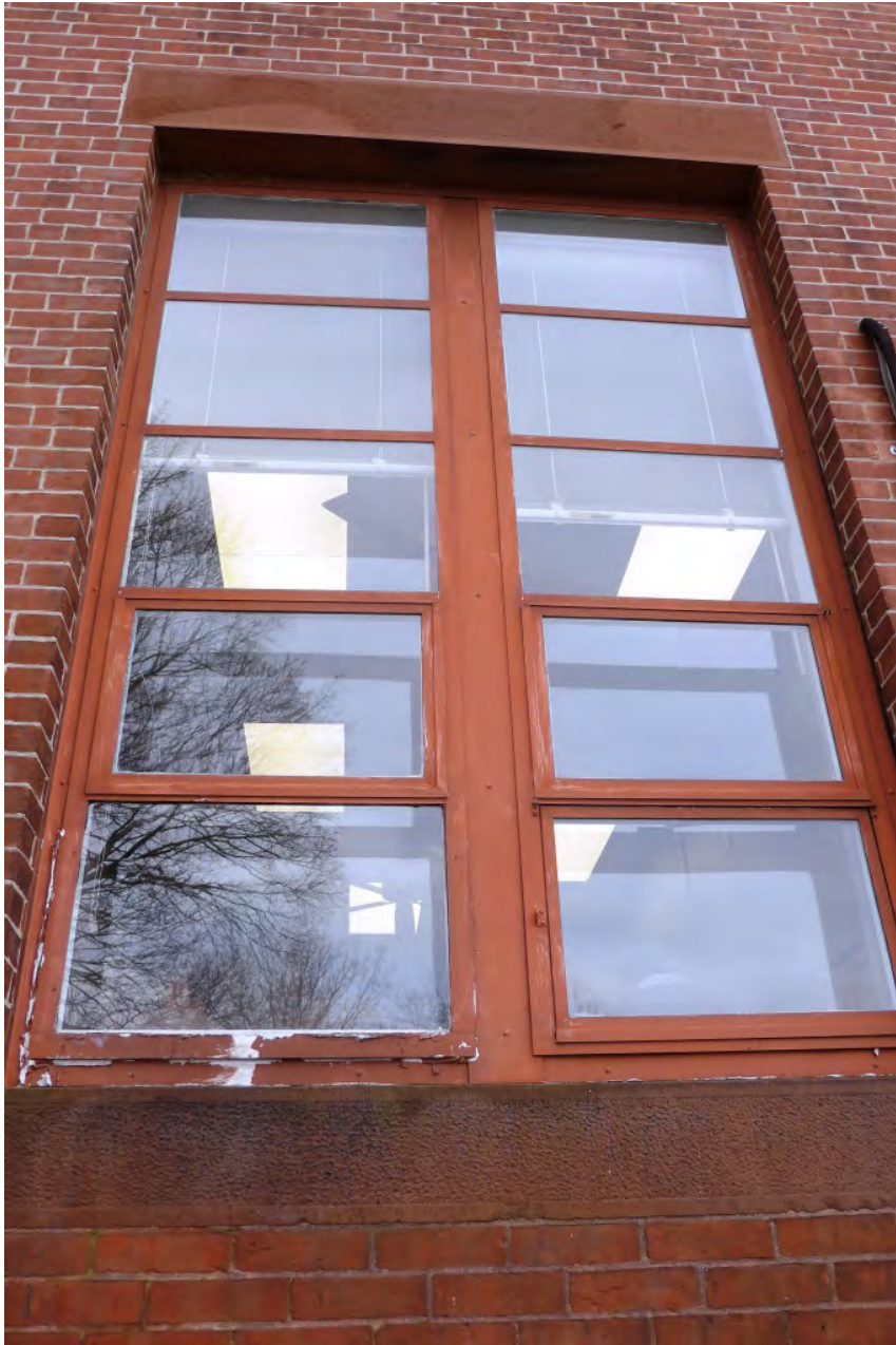
Cumberland Town Hall – Exterior - Windows, Doors and Hardware North Elevation – Central Pavilion - First Floor – Typical Replacement Window Historically Inappropriate Aluminum Hopper Replacement Window
