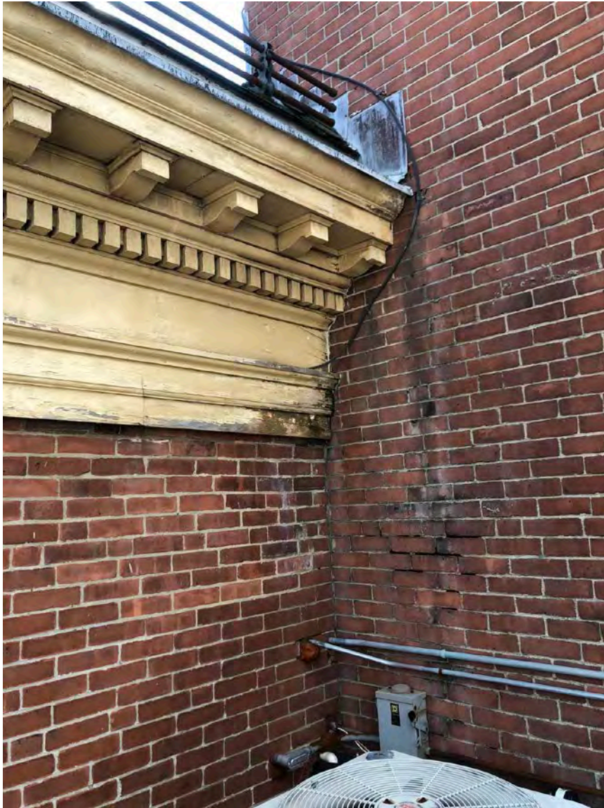
Cumberland Town Hall – Exterior - Masonry Inside Northeast Corner – Above Elevator Roof Open Joints, Eroded Brickwork, Staining, Worn and Peeling Paint – Due to Gutter Overflow
