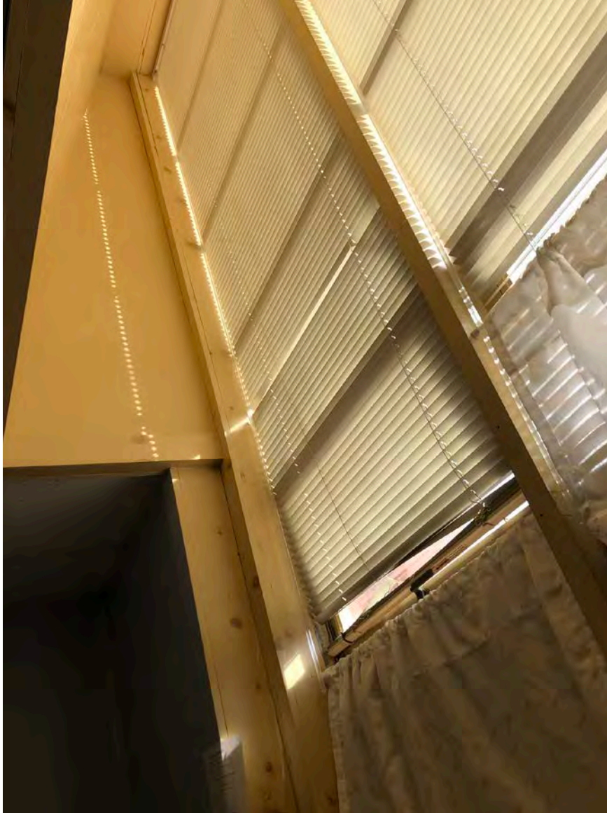
Cumberland Town Hall – Interior – Windows, Doors and Hardware Second Floor – Public Works Office Dropped Ceiling Bisects Original Windows; Inappropriate Replacement Windows; Transom Not Visible
