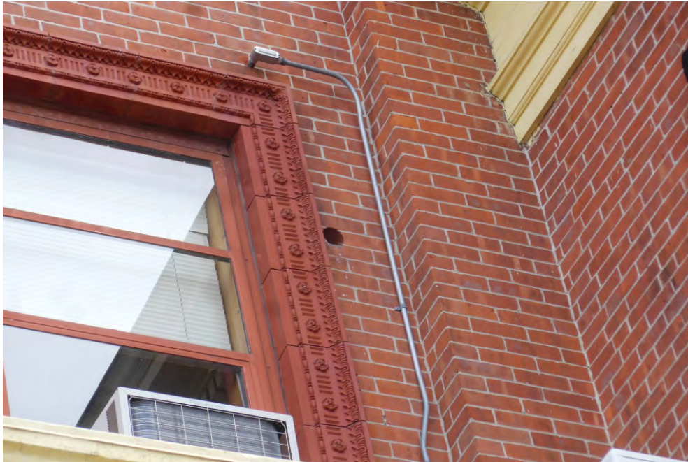
Cumberland Town Hall – Exterior - Masonry West Elevation – North Pavilion – South Window - Second Floor – Window above Entrance Open Joints, Eroded Brickwork
