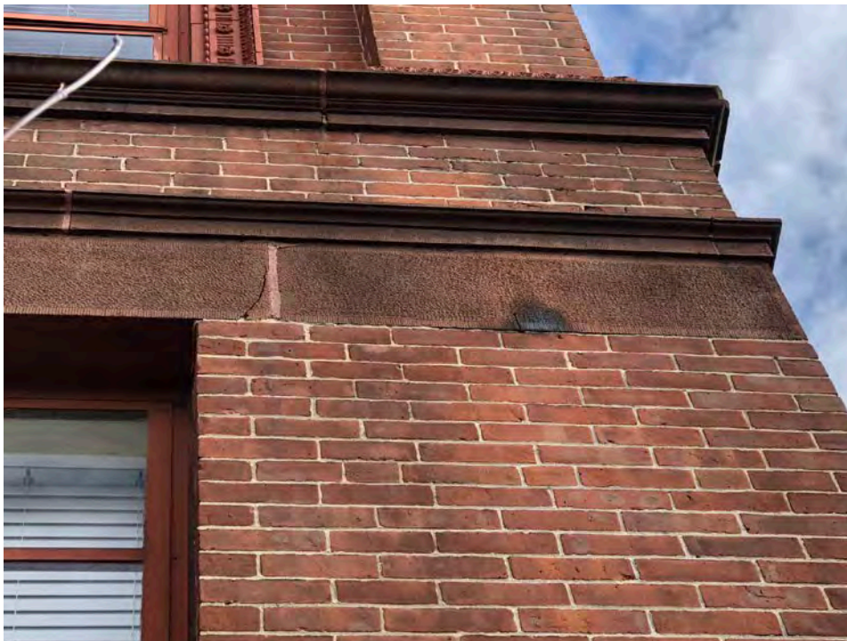
Cumberland Town Hall – Exterior - Masonry West Elevation – South Pavilion – South Corner - First Floor – South Corner Cracked Brownstone, Staining
