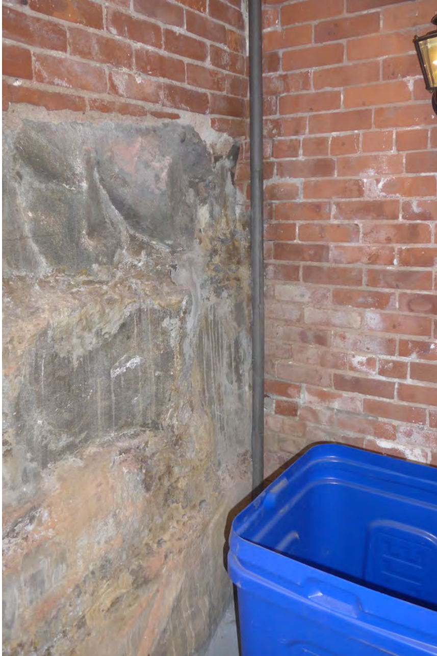
Cumberland Town Hall – Interior - Masonry Basement – Entrance Looking Toward Handicap Access Efflorescence Staining in Brick and Stone
