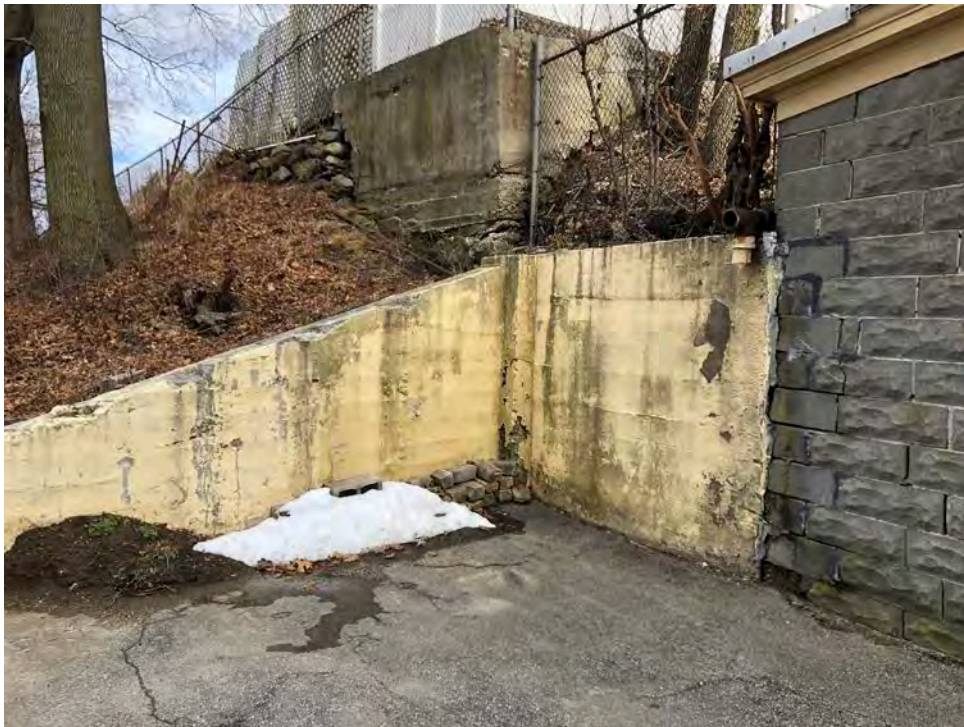
Cumberland Town Hall – Exterior – Retaining Walls, Steps, Landscaping, Asphalt Parking Area and Miscellaneous Landscaping Elements Northeast Corner - Retaining Wall and Wall of Garage Retaining Wall in Poor Condition, Step Cracks in Garage Wall
