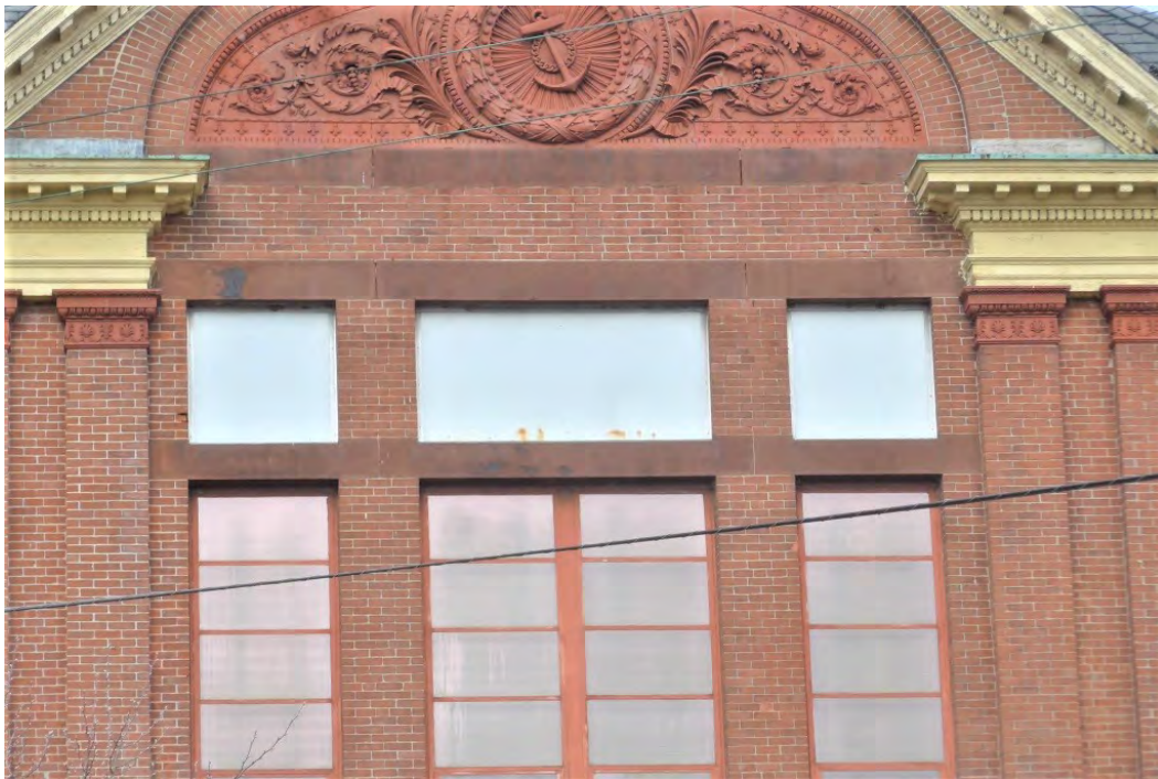
Cumberland Town Hall – Exterior - Masonry South Elevation – Central Pavilion Open Joints, Deteriorated/Missing Brickwork; Staining
