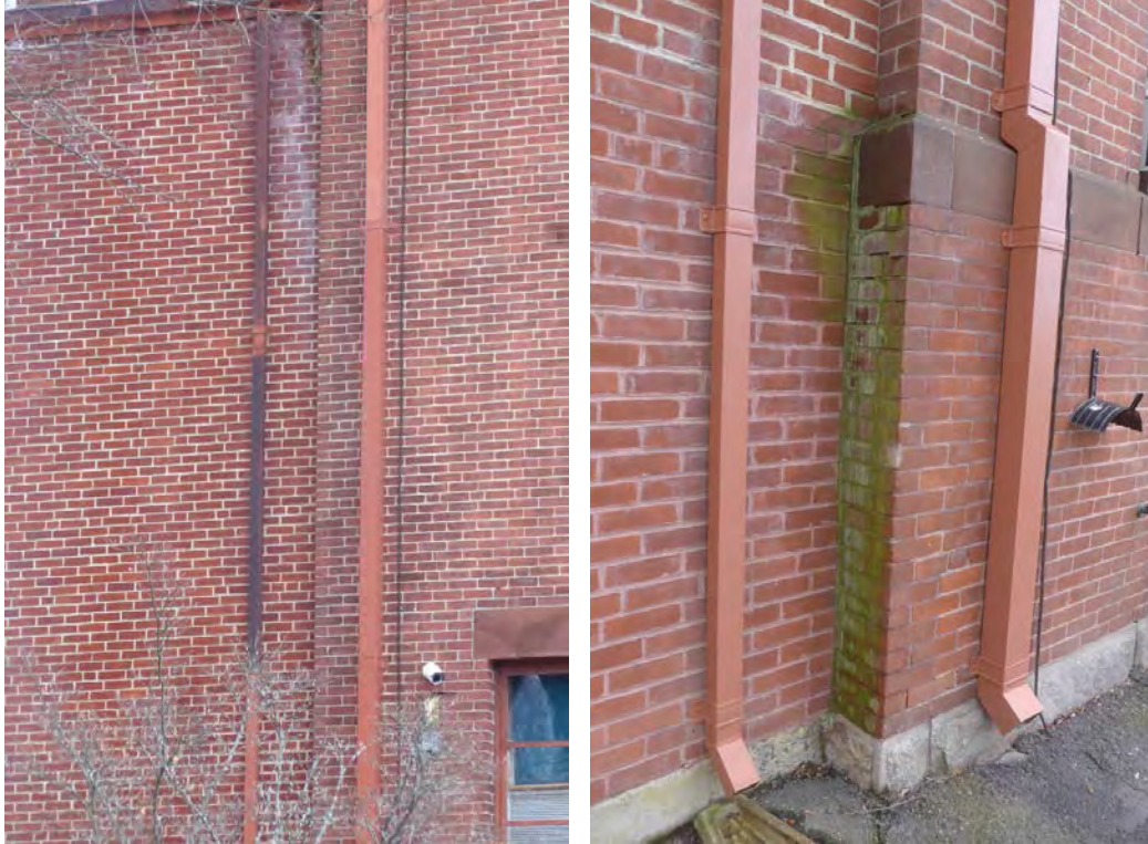
Cumberland Town Hall – Exterior - Masonry North Elevation – at Elevator Addition Efflorescence and Biological Staining
