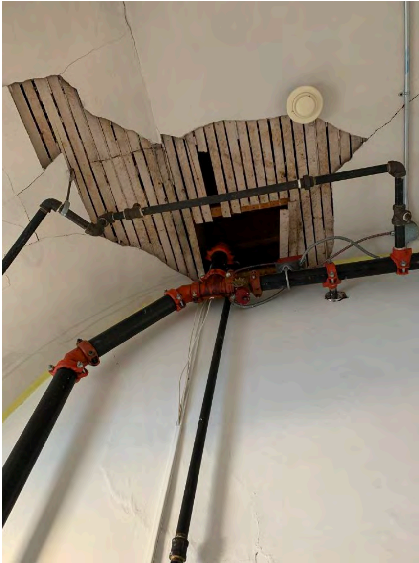
Cumberland Town Hall – Interior – Plaster Walls and Ceilings – Code Compliance Main Stair Cracked, Damaged and Missing Plaster on Walls and Ceiling; Unsealed Penetration
