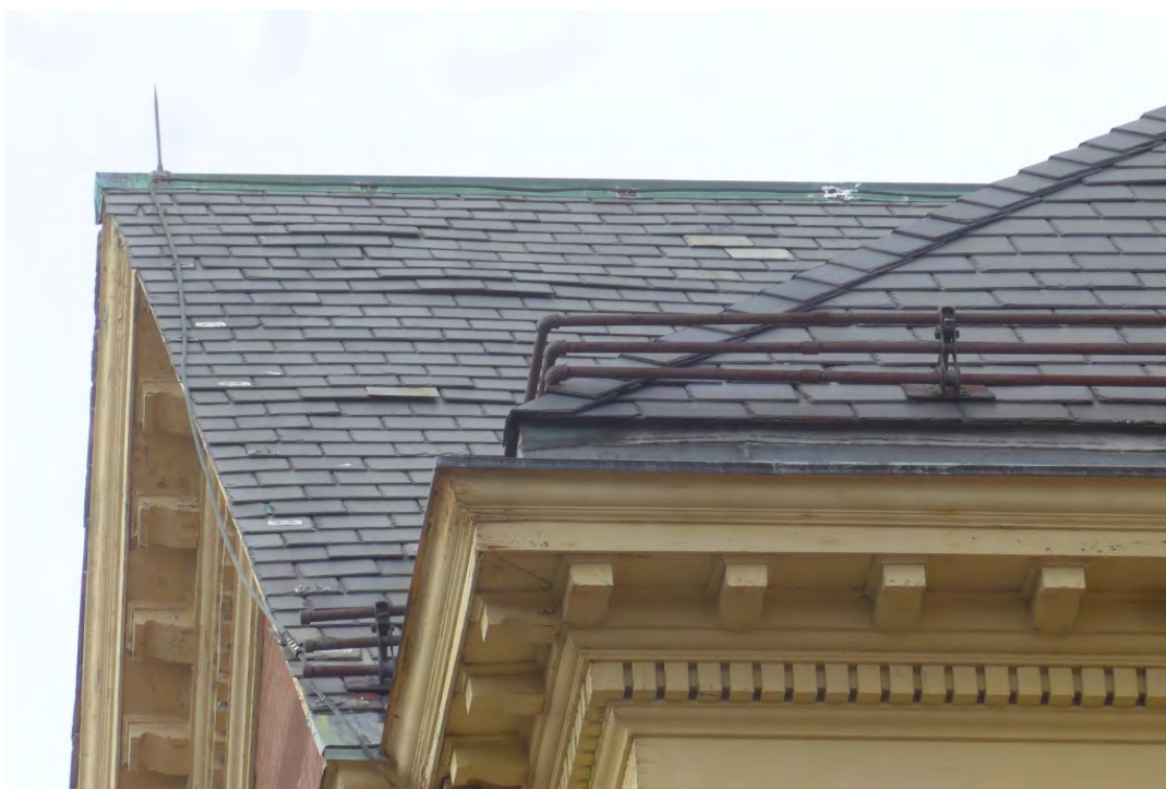
Cumberland Town Hall – Roofing, Flashing, Gutters, Leaders, Metal Trim and Roofing Elements East Slope over South, Central Pavilion - Detail Damaged, Lifted, Replacement Slates
