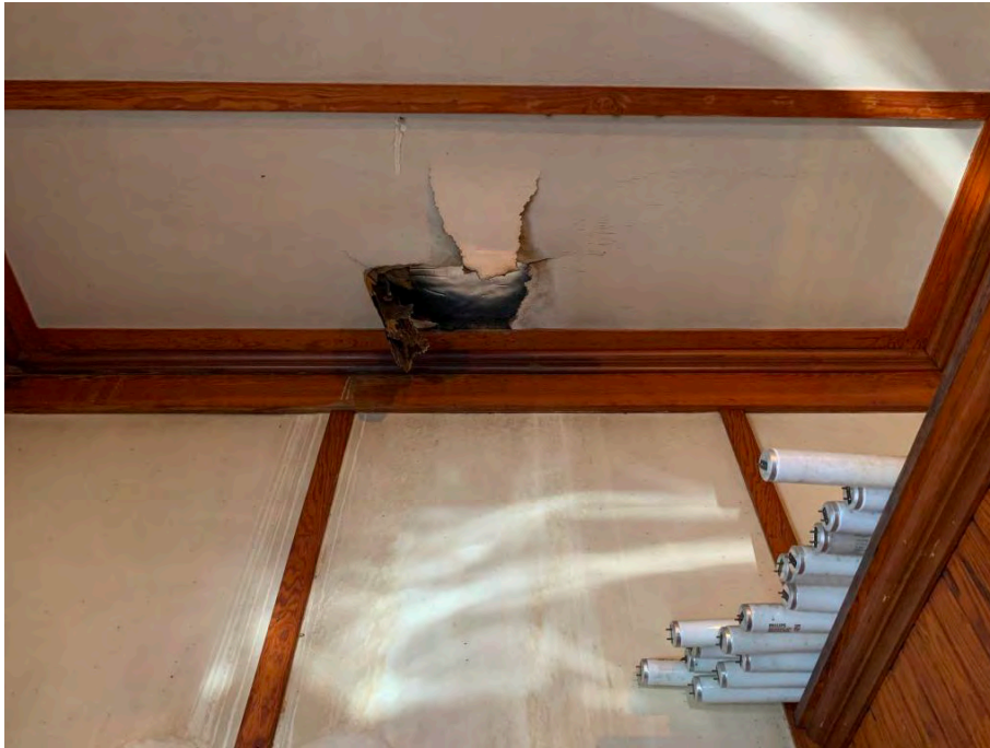
Cumberland Town Hall – Interior – Historic Finishes and Elements Third Floor – Southwest Corner Room 1930s-era Paneled Walls and Ceiling Damaged from Previous Leak
