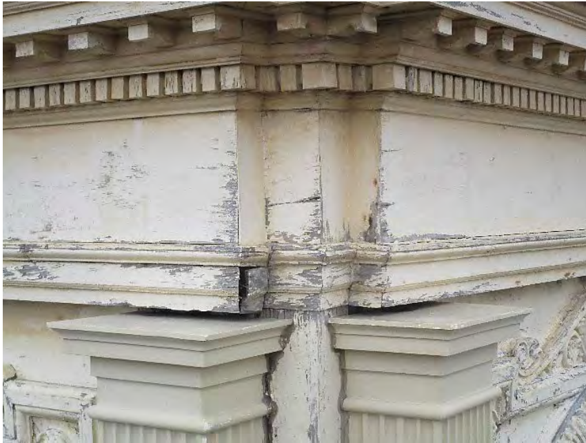
Cumberland Town Hall – Exterior – Wood Elements Tower – Clock Level (Sixth Floor) Flaking and Deteriorated Paint – Some Deteriorated Wood Source: Town of Cumberland
