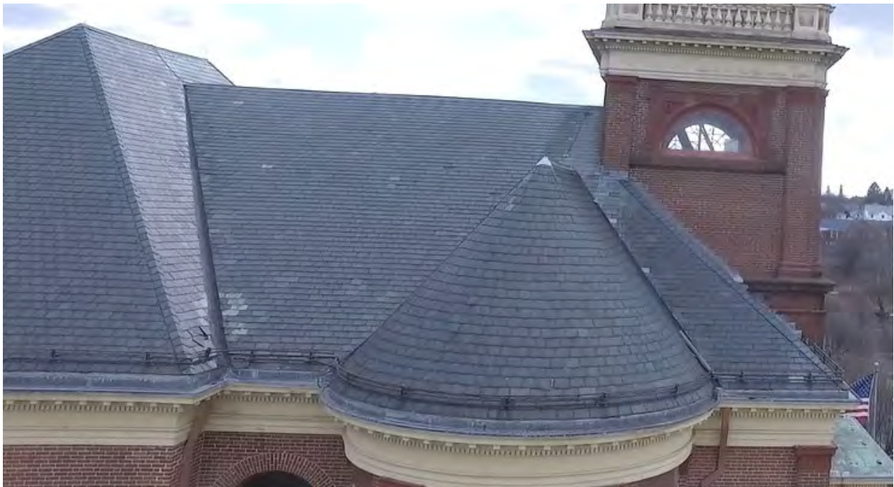
Cumberland Town Hall – Roofing, Flashing, Gutters, Leaders, Metal Trim and Roofing Elements View of North Slope, West End of Building Overall in Good Condition – Isolated Areas of Displaced, Damaged or Missing Slates
