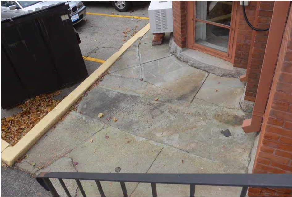
Cumberland Town Hall – Exterior – Landscaping Elements South Elevation – Concrete Pavement adjacent to Building Cracking and Settlement Overall in Good Condition; Some Cracking and Settlement of Concrete Pavement
