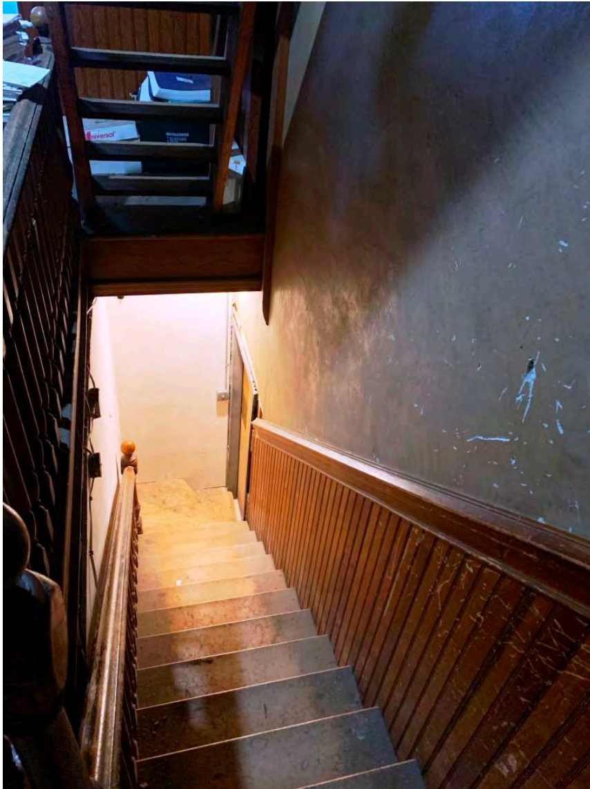
Cumberland Town Hall – Interior – Plaster Walls and Ceilings Third Floor – Base of Tower – Stair from Second to Third Floor Damaged Plaster and Wood Walls
