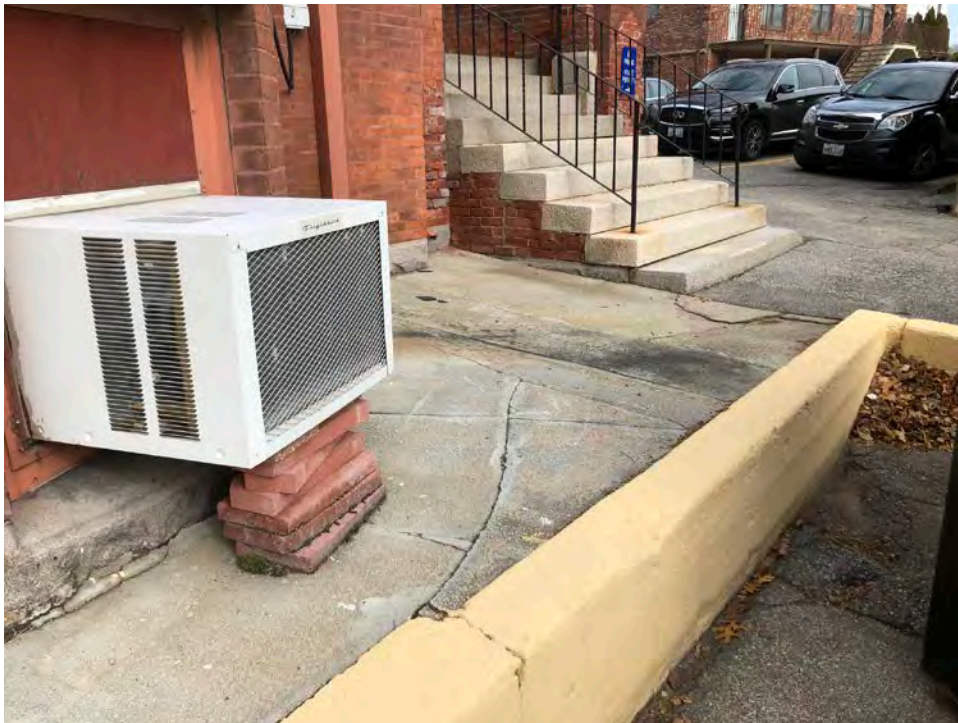
Cumberland Town Hall – Exterior – Landscaping Elements South Elevation – Concrete Pavement adjacent to Building Some Cracking and Settlement of Concrete Pavement; Pavers used to Support AC Unit
