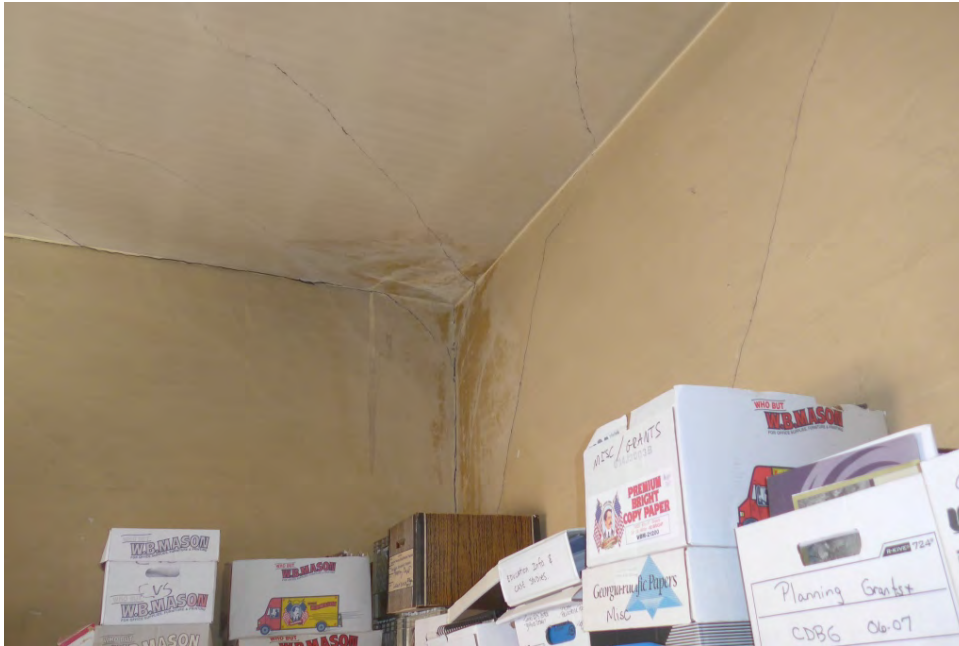
Cumberland Town Hall – Interior – Plaster Walls and Ceilings Third Floor – East Storage Area Damage from Previous Leak; Cracks in Plaster Walls and Ceiling
