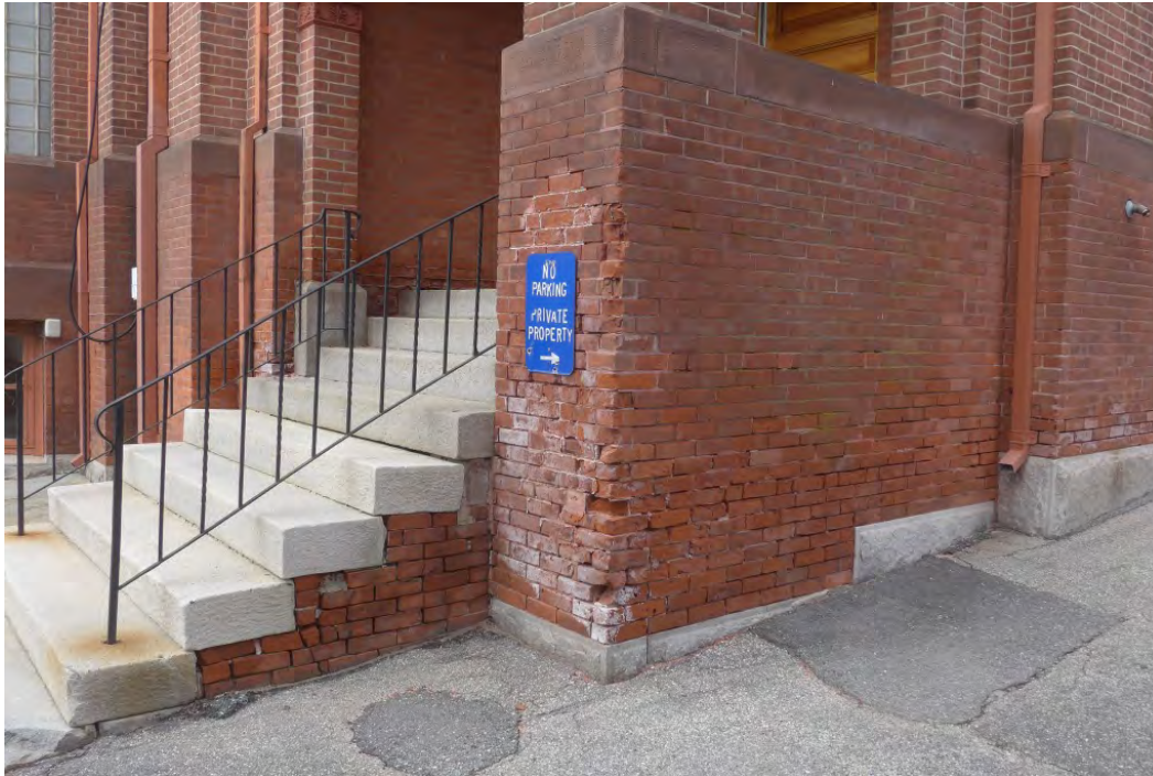
Cumberland Town Hall – Exterior - Masonry South and East Elevations - Southeast Corner – Entrance Open Joints, Deteriorated/Missing Brickwork; Staining
