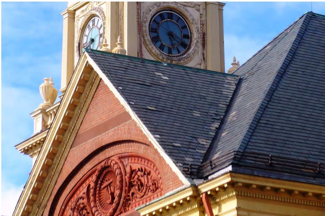
Cumberland Town Hall – Roofing, Flashing, Gutters, Leaders, Metal Trim and Roofing Elements East Slope over South, Central Pavilion Damaged, Lifted, Replacement Slates
