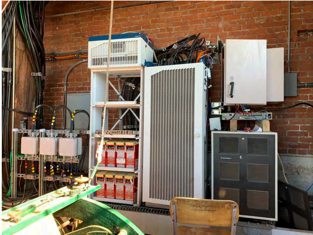
Cumberland Town Hall – Interior Tower – Fifth Floor Cell Service Equipment in Tower
