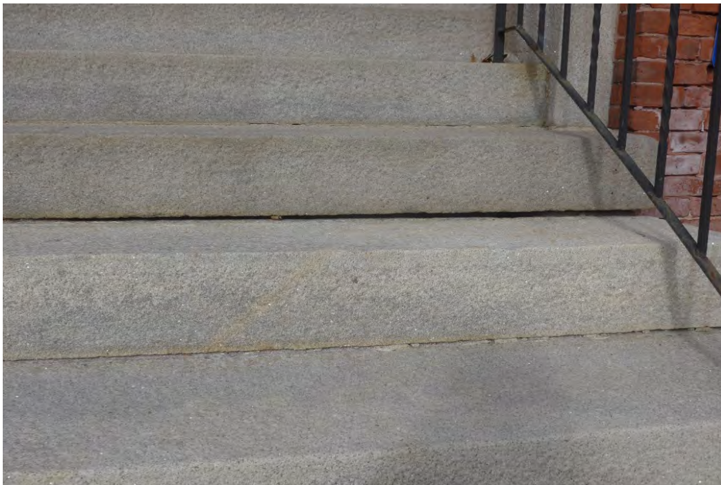
Cumberland Town Hall – Exterior - Masonry Southeast Corner – Entrance Open Joints at Granite Steps
