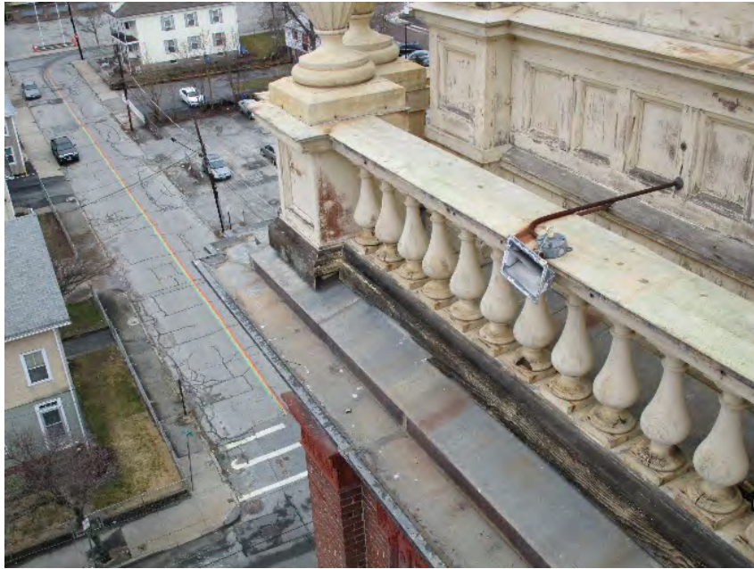
Cumberland Town Hall – Exterior – Wood Elements Tower – Lower Balustrade at Clock Level (Sixth Floor) Flaking and Deteriorated Paint , -Deteriorated Wood and Rusting Light Fixture Conduit Source: Town of Cumberland
