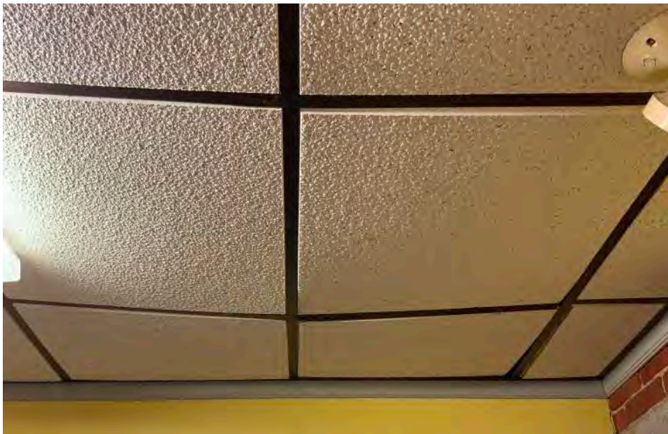
Cumberland Town Hall – Interior - Overall Basement – Employee Break Room Buckling of Dropped Acoustical Ceiling
