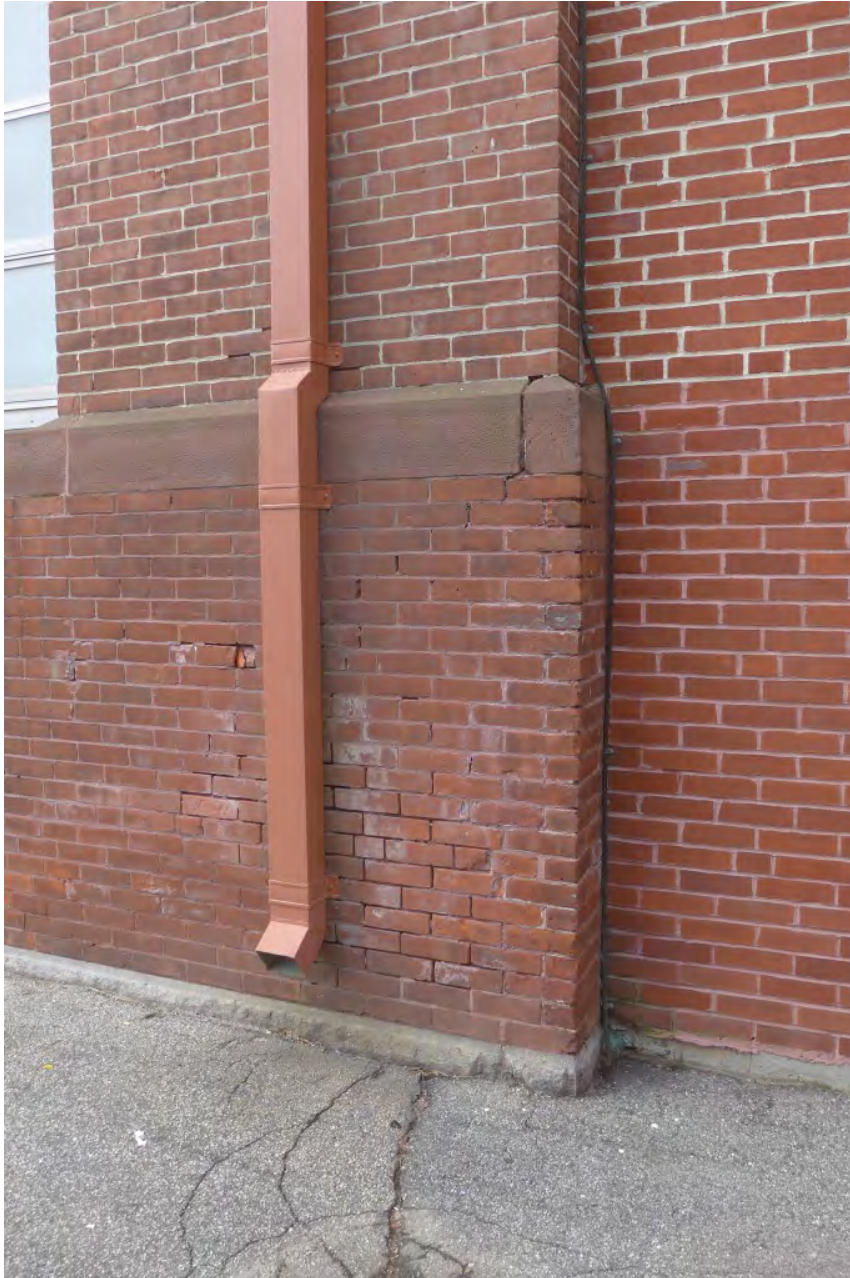
Cumberland Town Hall – Exterior - Masonry East Elevation – at Elevator Addition Open and Eroded Mortar Joints; Step Crack; Damaged Brickwork; Staining No Splashblock
