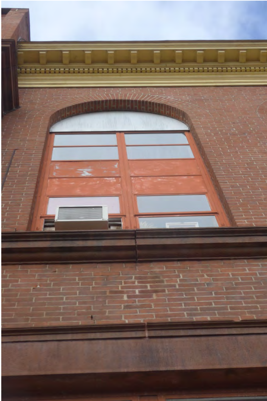
Cumberland Town Hall – Exterior - Windows, Doors and Hardware South Elevation – West Pavilion - Second Floor – Typical Replacement Window Historically Inappropriate Aluminum Hopper Replacement Window; Covering of Arched Transom
