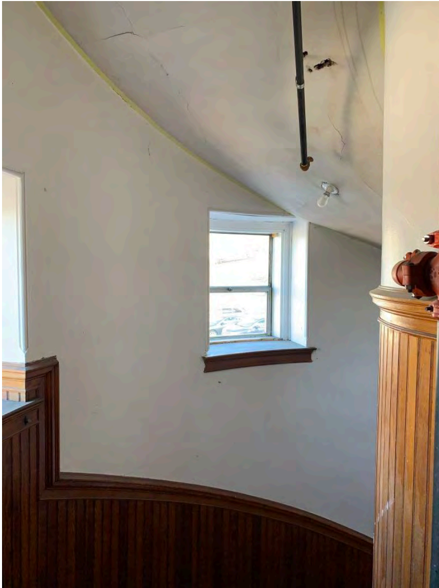
Cumberland Town Hall – Interior – Plaster Walls and Ceilings Main Stair Cracked, Damaged and Missing Plaster on Walls and Ceiling
