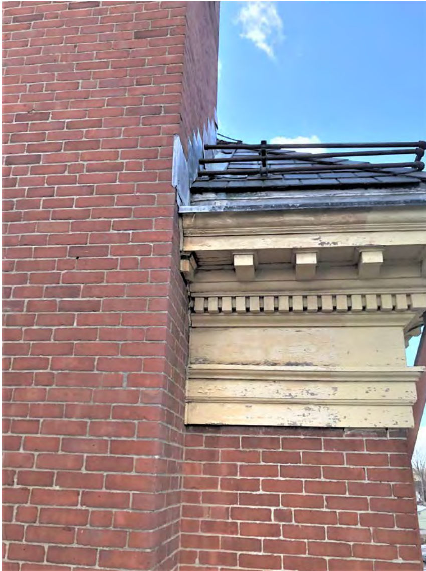
Cumberland Town Hall – Exterior – Wood Elements East Elevation – above Elevator Addition Worn/Peeling Paint; Deteriorated Wood Elements Bent Snow Guard Piping
