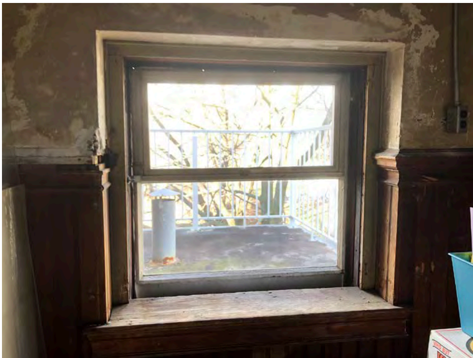
Cumberland Town Hall – Interior – Plaster Walls and Ceilings – Windows, Doors and Hardware Third Floor – East Storage Area Damage from Previous Leak
