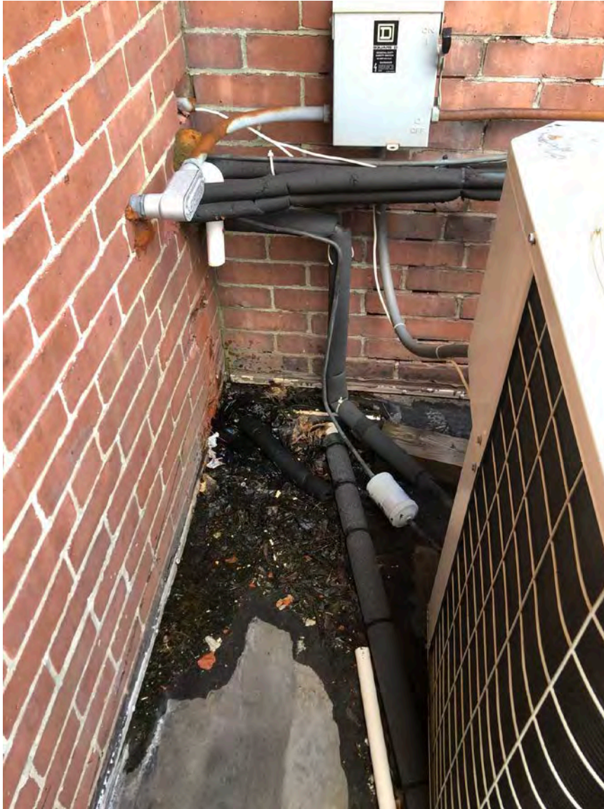
Cumberland Town Hall – Roofing, Flashing, Gutters, Leaders, Metal Trim and Roofing Elements Roof Above Elevator Addition Rubber Membrane Roof; Ponding and Debris in Corner; Open Joints in Brickwork
