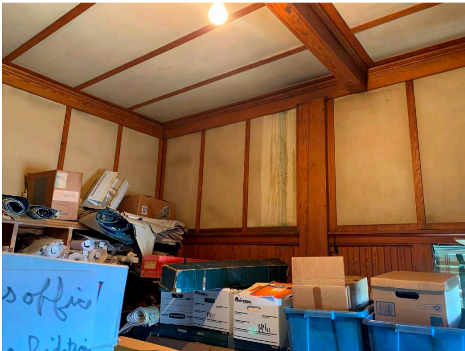
Cumberland Town Hall – Interior – Historic Finishes and Elements - Storage Third Floor – Southwest Corner Room 1930s-era Paneled Walls and Ceiling Damaged from Previous Leak Excessive Storage Creating Substantial Load
