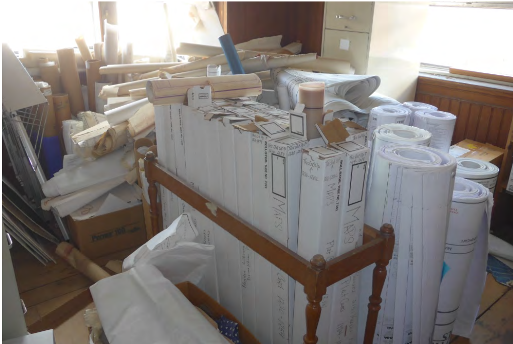
Cumberland Town Hall – Interior – Plaster Walls and Ceilings - Storage Third Floor – East Storage Area Excessive Storage Creating Substantial Load
