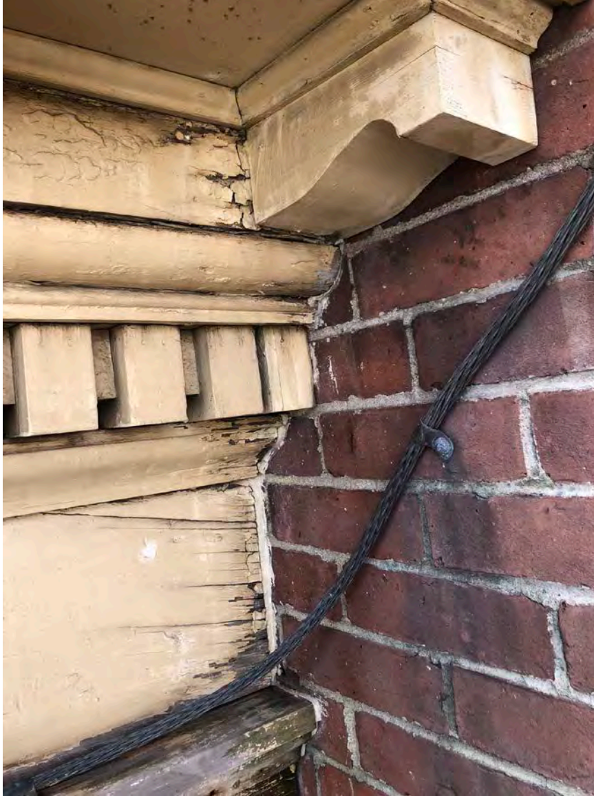
Cumberland Town Hall – Exterior – Wood Elements North Elevation – Inside Northeast Corner - above Elevator Addition Worn/Peeling Paint; Deteriorated Wood Elements
