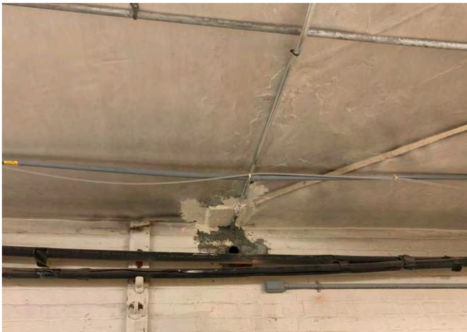
Cumberland Town Hall – Interior - Overall Basement – Vault under West Entrance Stair Moisture Issues at Upper Portion of Walls and Ceiling – Unsealed Penetration
