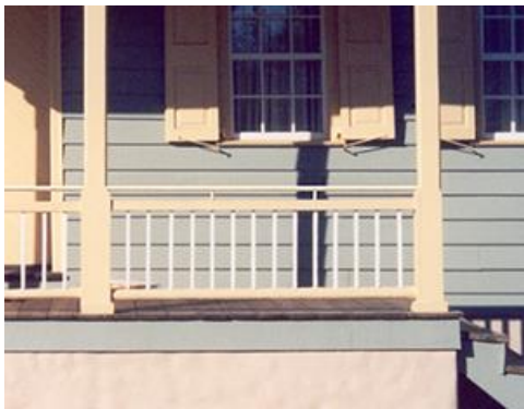
Figure 22 The use of a secondary railing which has been added to a historic rail baluster for additional safety.
