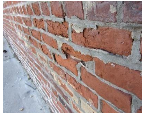
Figure 14 Historic masonry that has been repointed with Portland cement which has led to degradation.
