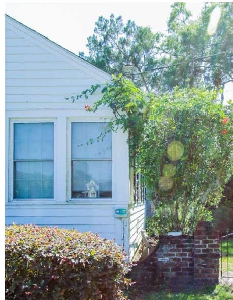
Figure 18 Vegetation adjacent to a historic building that could become a detriment to the building.
