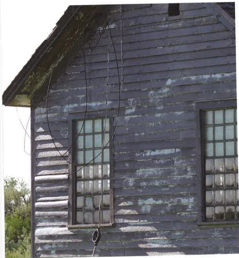
Photograph 13: Evidence of electrification at the Mont Township School.
