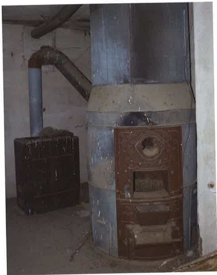
Photograph 12: Grey School basement furnace system. Coal storage located through door beside stairs.
