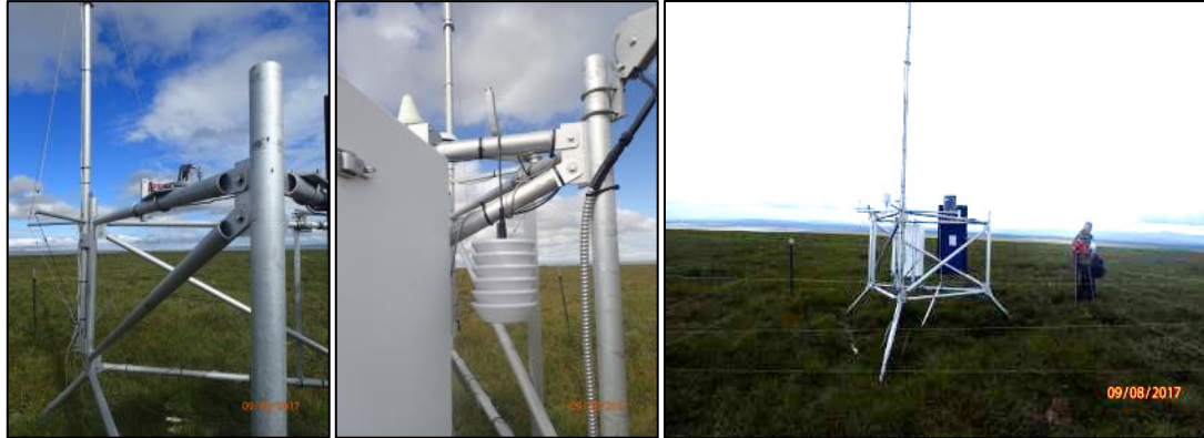
Figure 19. Hoodoo Hills fire RAWS station, August 9, 2017 showing the damaged RG-TB (left) and AT-RH sensors (middle). The right photo shows the site after repairs and maintenance.
