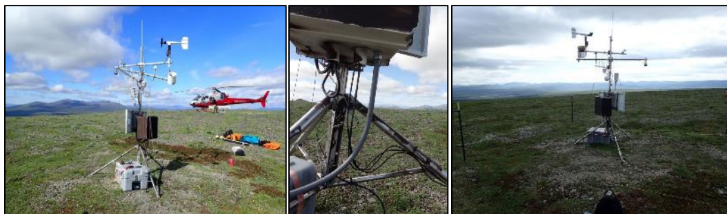
Figure 13. Sisiak climate station July 21, 2018. Upon arrival at the site the long crossarm was out of level, the tipping bucket funnel was missing (left). The soil temperature cables have been pulled on, but not damaged (middle). The station was repaired, and an electric fence was installed (right).
