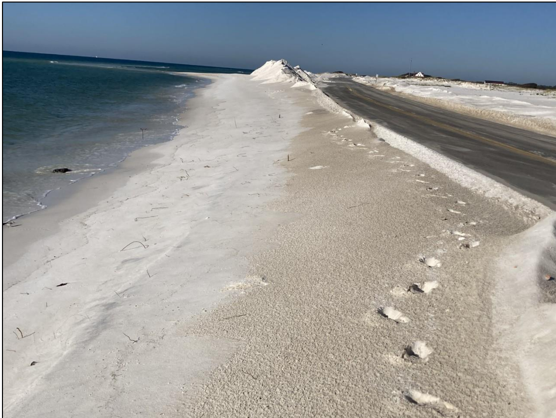
Figure 10. Fort Pickens road after Hurricane Sally removed over 100 feet of Gulf facing shoreline. This is the most egregious section at GUIS regarding shoreline erosion threatening infrastructure.
