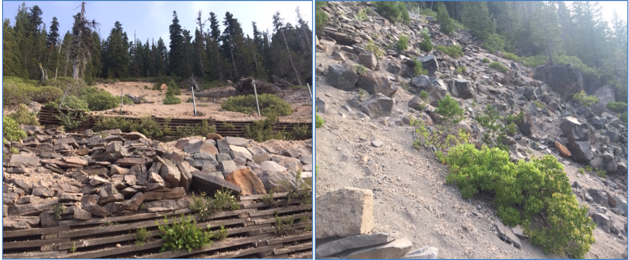
Figure 2. Failing cribbing and rock retaining wall (left); unstable, rocky pumice soils (right) on the Cleetwood Cove trail. Photos by Carrie Wyler.
