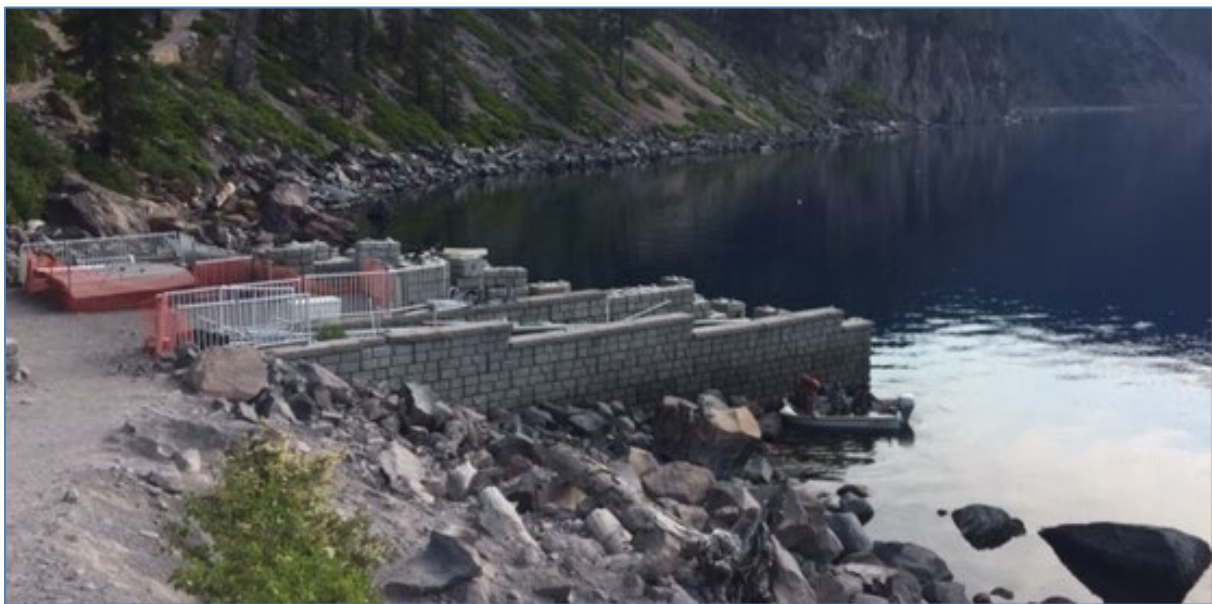
Figure 3. View of Crater Lake's shoreline and failed dock and bulkhead. Photo by Carrie Wyler.
