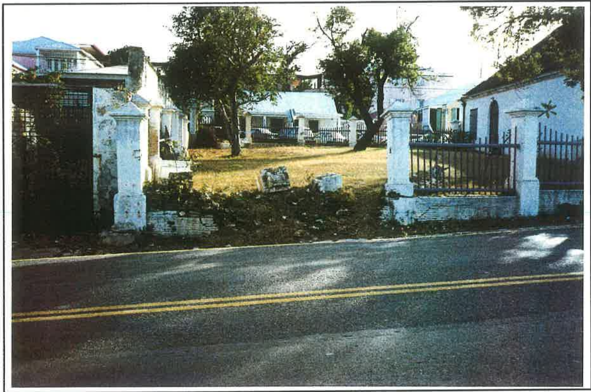
Steeple Building Fence showing Hurricane Hugo damage
