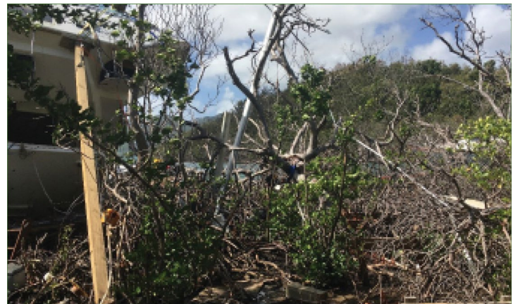
Figure 5. Hurricane damage at Saint John VIIS SET site. Severe wind damage caused debris deposits, mangrove die-off, and missing or damaged platform boards. This site had a capsized 30 foot boat in it.
