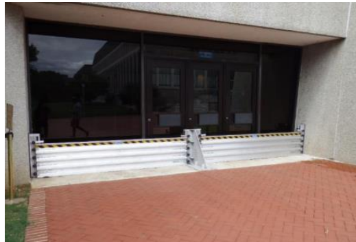
Figure 23: Flood barriers outside Rickover Hall at USNA
