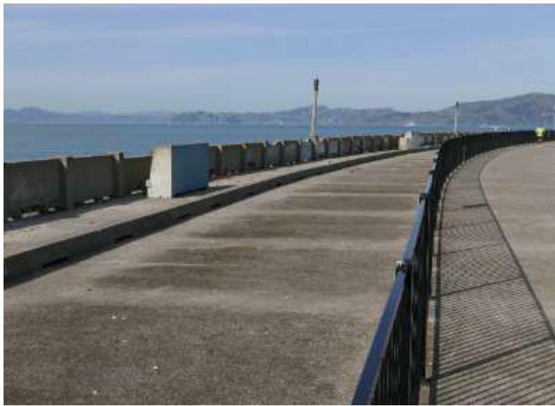
Figure C8: Half of the pier blocked from pedestrian use due to failed concrete hand railing (MIDN Myers, 2020)
