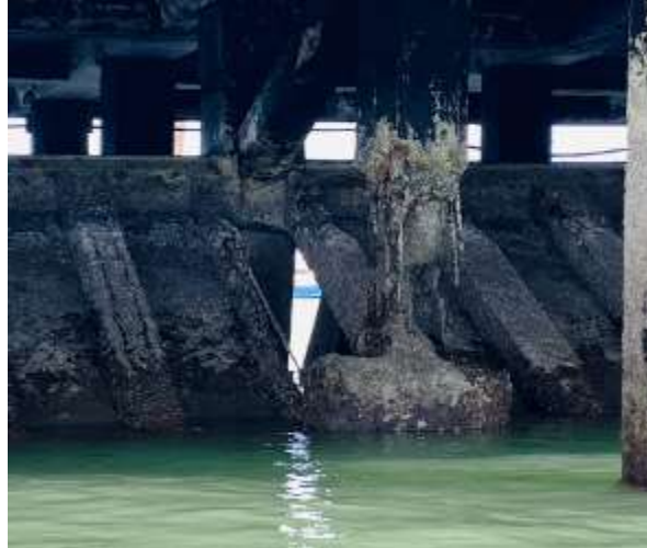
Figure C3: Spalling wave baffle and eroded piling (MIDN Ostrowski and Prince, 2020)
