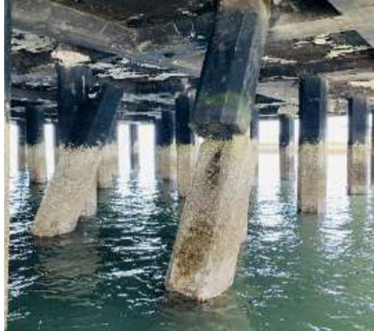
Figure C1: Broken piles from shear failure (MIDN Ostrowski and Prince, 2020)
