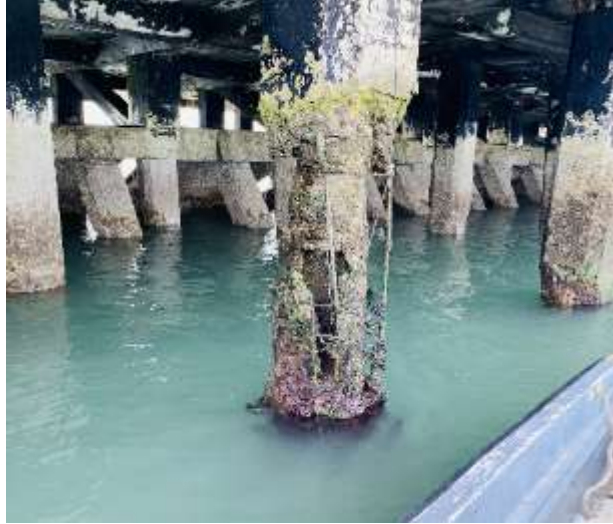
Figure C5: Spalled Pile with rebar and inner timber exposed (MIDN Ostrowski and Prince, 2020)
