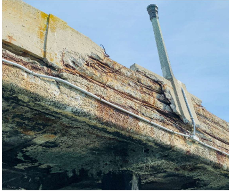
Figure 4: Spalling due to rebar corrosion (MIDN Connor Prince, Site Visit, 2020)
