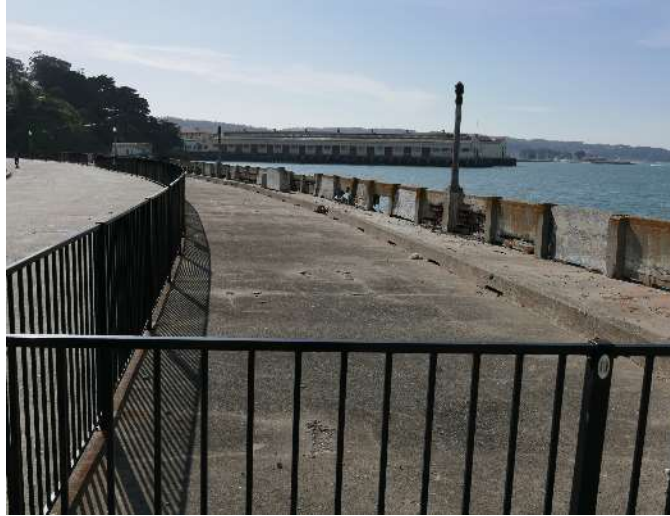
Figure C11: Restricted Area of the pier due to failed hand railing (MIDN Myers, 2020)
