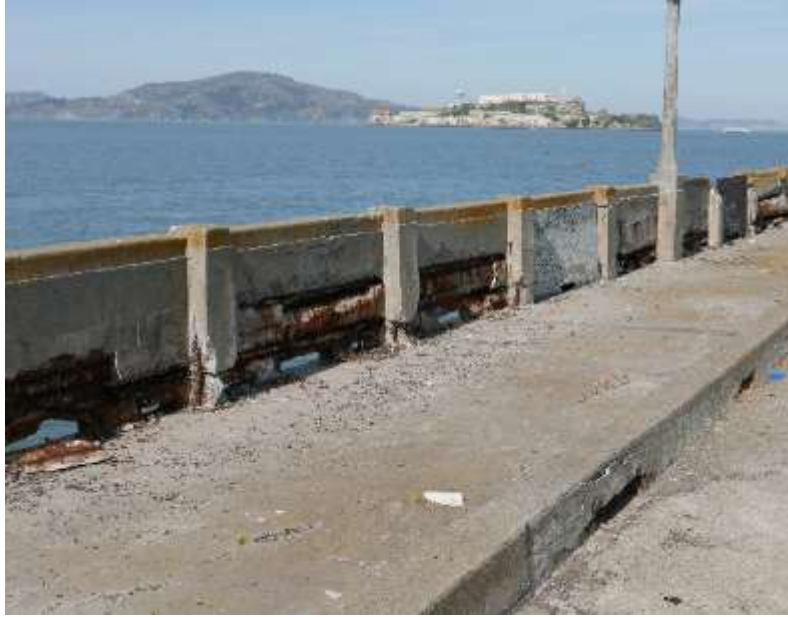
Figure C7: Spalling concrete handrail from the deck of the pier (MIDN Myers, 2020)
