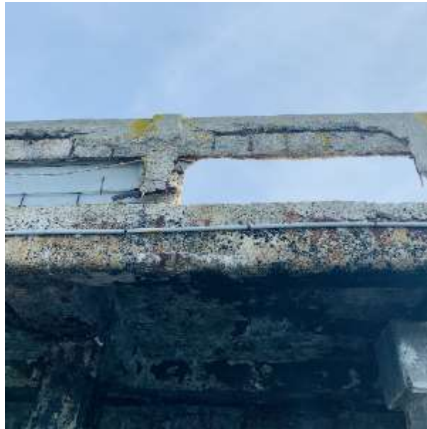
Figure C6: Spalled hand railing with steel rebar exposed (MIDN Ostrowski and Prince, 2020)
