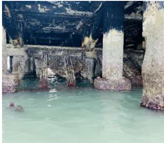
Figure C4: Broken wave baffle (MIDN Ostrowski and Prince, 2020)
