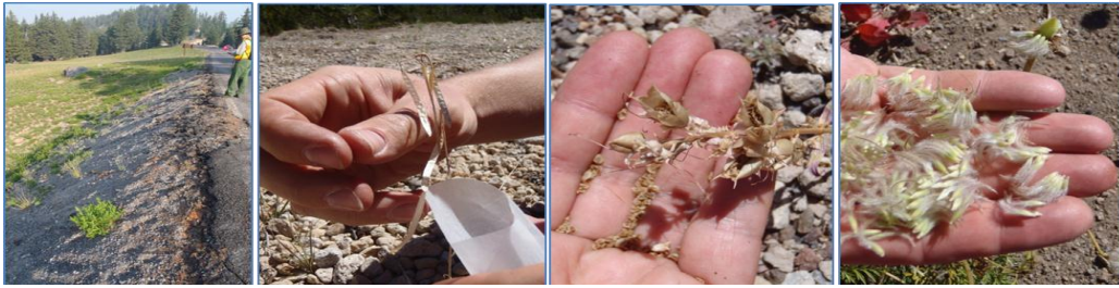
Crumbling pavement edge on West Rim Drive (left); collecting seed for revegetation of areas to be disturbed by the Rim Drive Rehabilitation project (center left, center right, right). Photos by Kathryn Williams.
