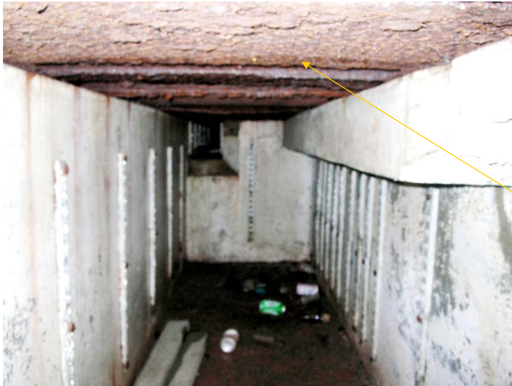
Floor Trench (T-Y)
