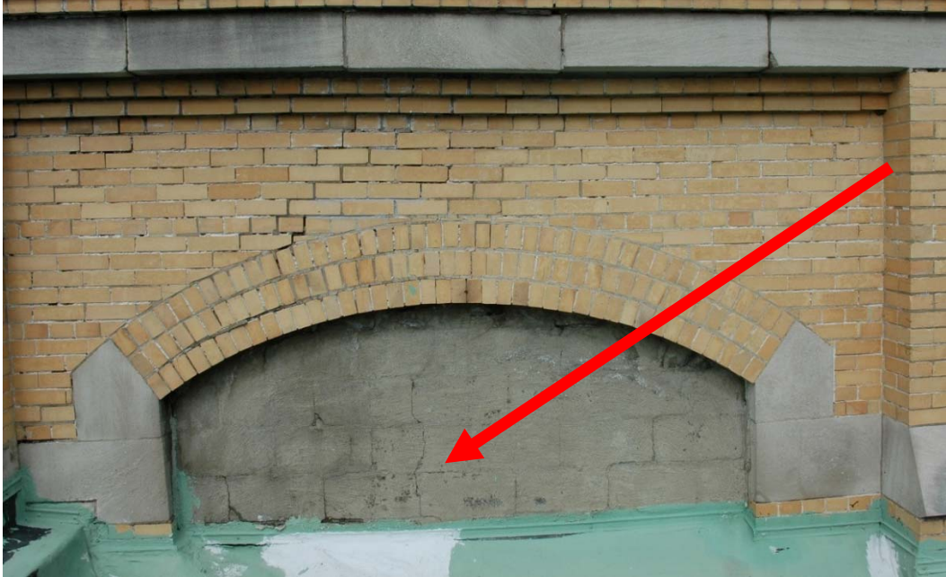
Figure 17: Moisture has penetrated the CMU infill and has caused cracks in the joints. This is the south infill of the 1910 building above the extension.
