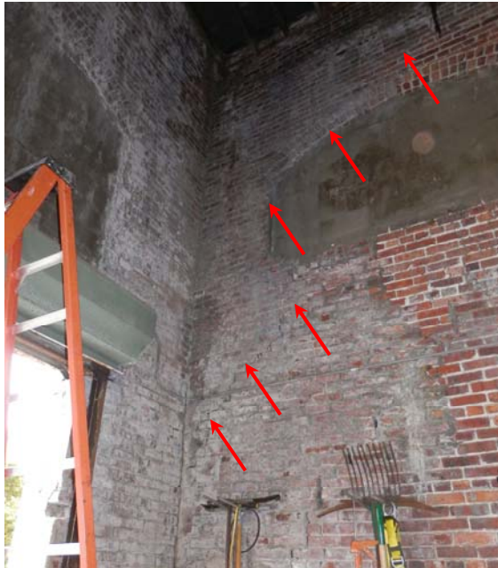
Image 13 – Crack in east wall at northeast corner of the original building.
