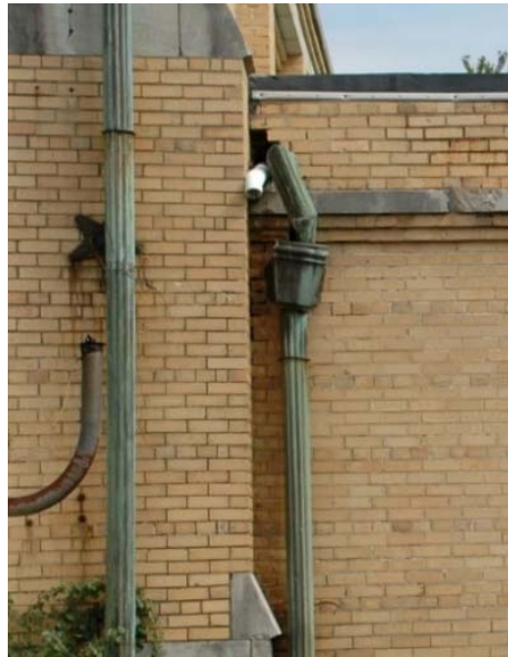
Figure 21: Typical downspout in need of replacement, located on the east end of the south elevation of the 1910 building.
