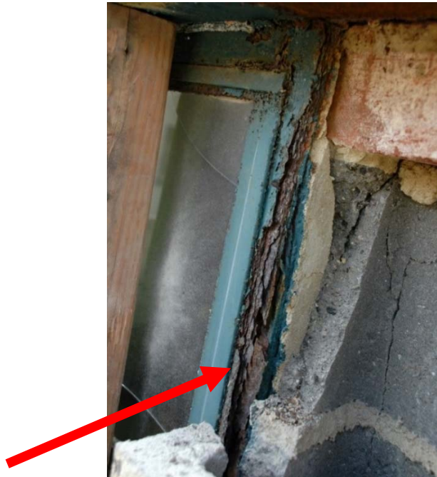
Figure 23: Delaminating steel of a typical window due to moisture. This window is located on the west end of the north elevation of the 1913 addition.
