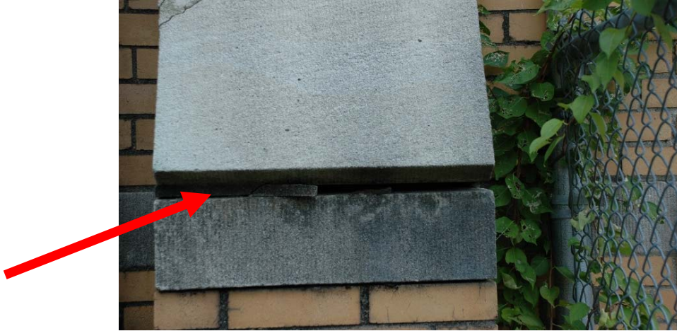
Figure 14: Mortar is missing between two pieces of limestone. This photograph shows the east pier of the south elevation of the 1913 addition.
