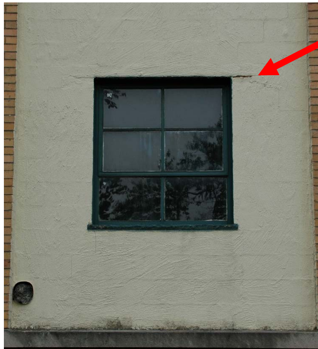
Figure 18: This deteriorating steel window, located in the south opening of the north elevation, has expanded and caused cracks in the CMU infill.
