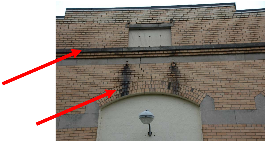
Figure 24: The top arrow shows atmospheric stains and the bottom arrow shows rust stains. This shows the center bay of the west elevation of the 1913 addition.
