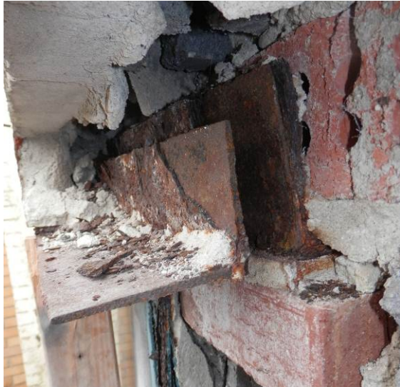
Image 8 – Two angles supported window opening at probe location W-1 (see Image 16). Outer angle is turned on its long side.
