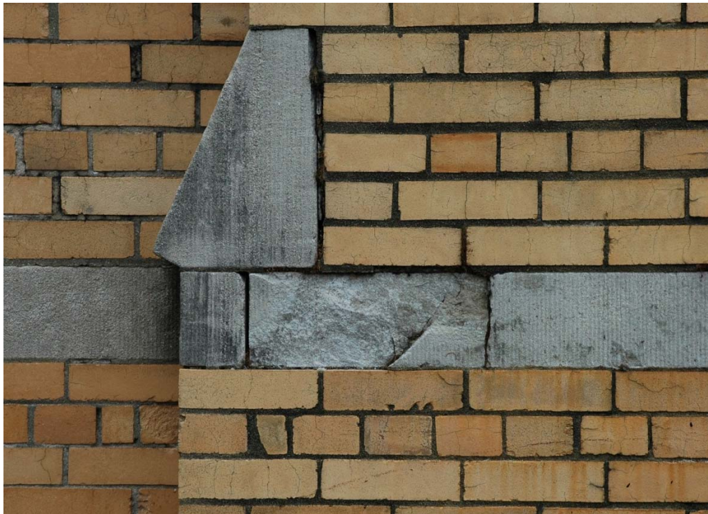
Figure 12: Much of the limestone is in fair to good condition with specific areas of damage. These damaged areas should be patched. This photograph shows the west end of the south elevation of the 1910 building.
