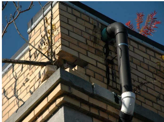
Figure 20: Water infiltration has resulted in openings in the mortar where vegetation is growing, damaging more bricks as a result. This is the east corner of the north elevation of the 1910 building.
