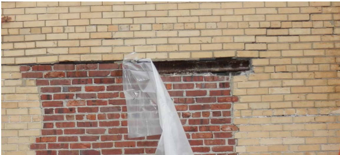
Image 10 – Probe location W-3 (see Image 16), showing masonry deterioration from rust-jacking.
