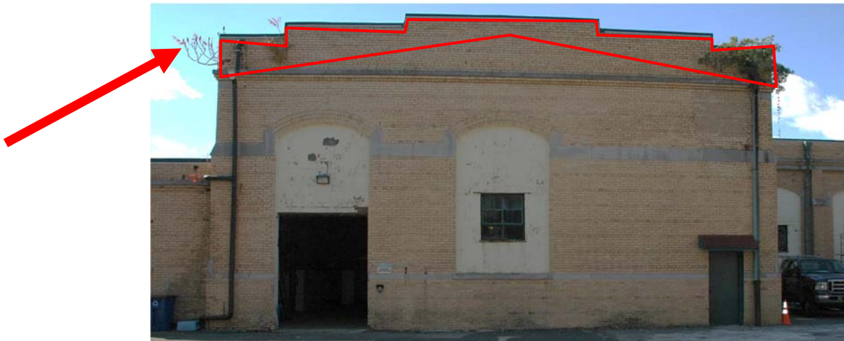
Figure 1: This photograph shows the north elevation of the 1910 building. The masonry parapet appears to be rotating, and is structurally unstable.
