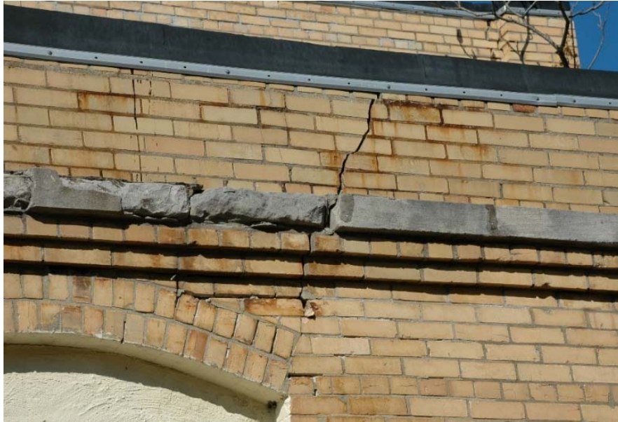
Figure 7: This photograph shows a crack in the masonry on the north side of the east elevation of the 1910 extension. The crack has resulted in broken bricks and a crack in the limestone belt course.
