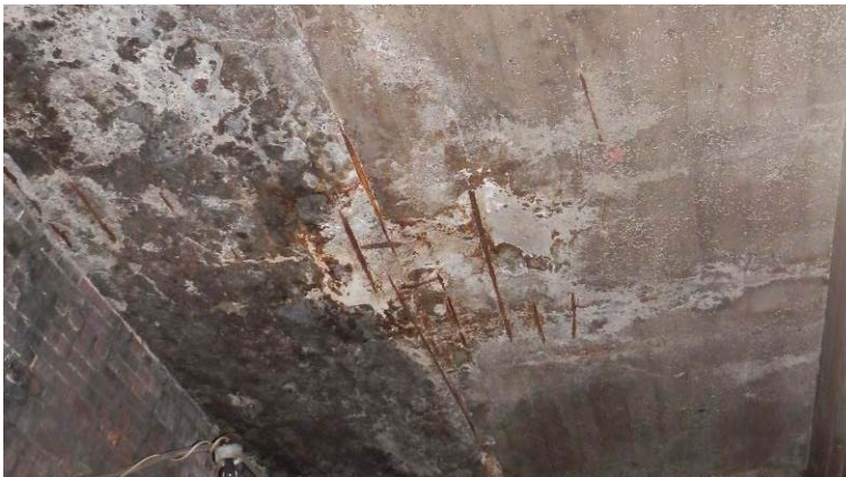
Image 15 – The underside of the concrete slab exhibits spalling and corroding reinforcing steel; shown location is just inside the east addition of the north portion of the original building.
