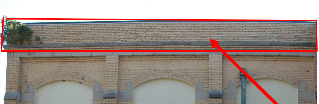
Figure 2: This photograph shows the west elevation of the 1910 building. The masonry parapet is in very poor condition and will need to be completely rebuilt from the large limestone band course up.
