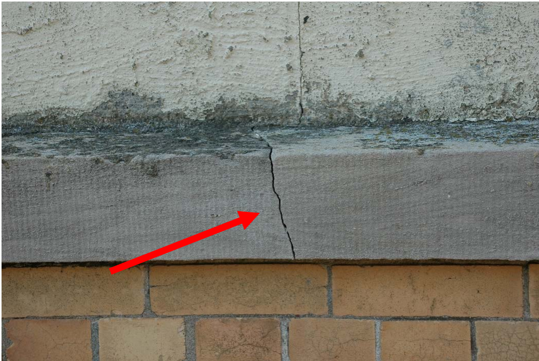
Figure 13: Typical limestone crack in a window sill that will need to be repaired. This sill is located on the west side of the north elevation of the 1910 extension.
