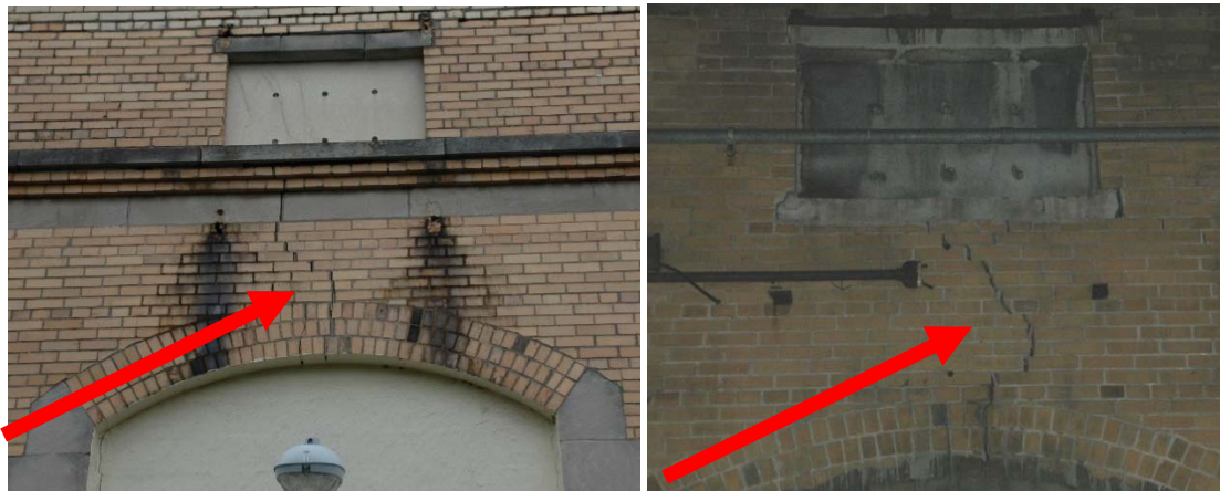
Figure 8: This photograph shows an exterior and interior crack in the bricks and mortar joint above the central door on the west elevation of the 1913 addition. This demonstrates the expansion and contraction of CMU vs. the expansion and contraction of brick.
