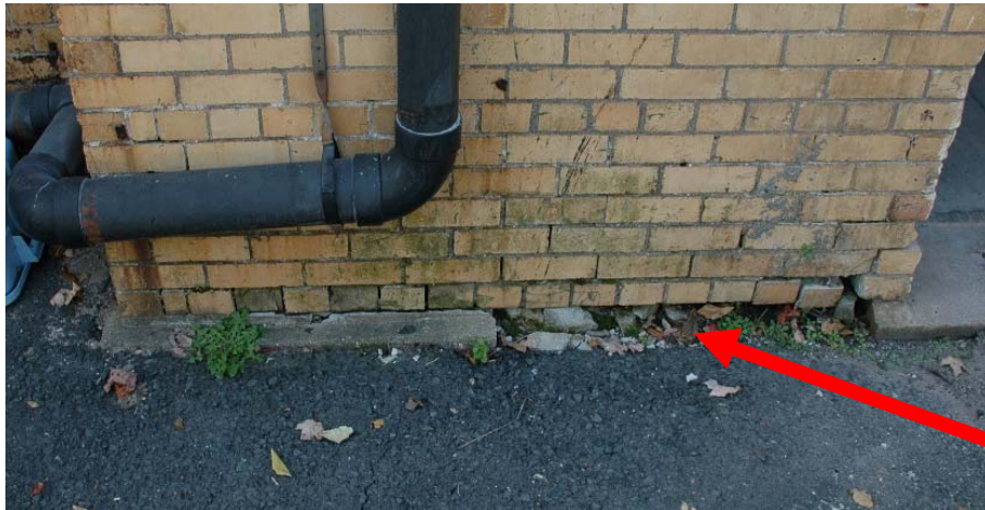
Figure 15: Parts of the limestone base are severely deteriorated. This photograph shows the east end of the north elevation.
