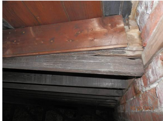
Image 14 – Split wood roof joist at sill with previous repairs as seen at probe location T-3 (see Image 16).
