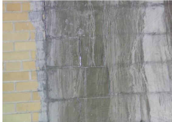
Image 12 – Crack through CMU infill on south wall of addition. Day light is visible through the crack.
