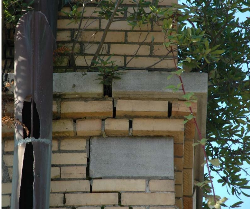
Figure 9: This photograph shows the west corner of the north elevation of the 1910 building. The limestone has shifted due to vegetation. The stone is in good condition but will need to be reset.
