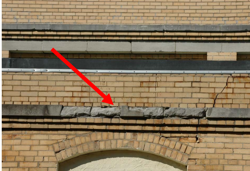
Figure 10: This photograph shows the limestone belt course on the north side of the east elevation of the 1910 building. This section of the belt course has severely deteriorated and will need to be replaced.
