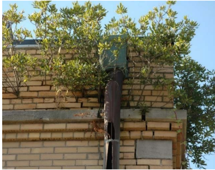
Figure 19: Infiltrating moisture has caused cracks and openings in the masonry, providing a place for vegetation. This photograph shows the west corner of the north elevation of the 1910 building.
