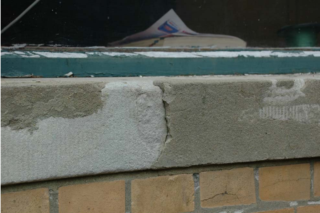
Figure 11: Some of the limestone is in fair to poor condition and has been previously patched, as seen here. Old failing patches will need to be removed and new patches installed. This photograph shows the south window of the east elevation of the 1910 extension.
