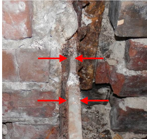
Image 7 – Section loss (top arrows) compared to intact section (bottom arrows) of bottom chord at probe location T-3 (see Image 16).
