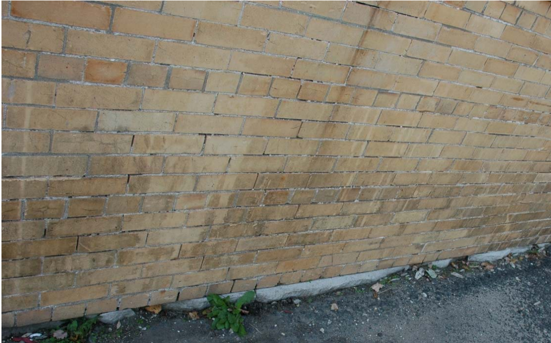
Figure 5: This photograph shows the west end of the north elevation of the 1910 building. The mortar in this area has deteriorated and will need to be repointed.
