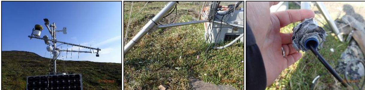
Figure 3. Killik Pass climate station July 15, 2021. Bear damage included crossarm orientation (left), sensors/cables (middle), and the battery cable (right).
