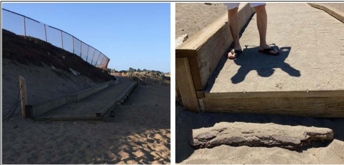
Figure 2 - Original 2018 (left) and Current 2020 (right) condition of the accessible ramp transition
