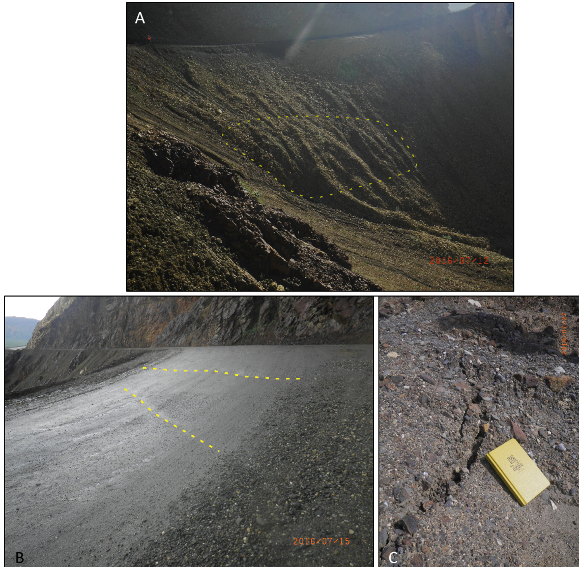
Figure 8. (A) Convex morphology downslope of the road. Numerous debris flow levees also visible. Person for scale (top left, wearing orange.) Photo taken looking northeast. (B) Northwestern road cracks. The westernmost crack (above, in this view) is longer, more prominent, and was visible more often during field work in July 2016. Highlights added for clarity, but do not represent full extent of cracks. Photo taken looking southwest. Road is one lane wide, for scale. (C) Detail of crack immediately upslope of northwestern road crack. Offset magnitude and aperture varied based on road maintenance interval and precipitation amount.
