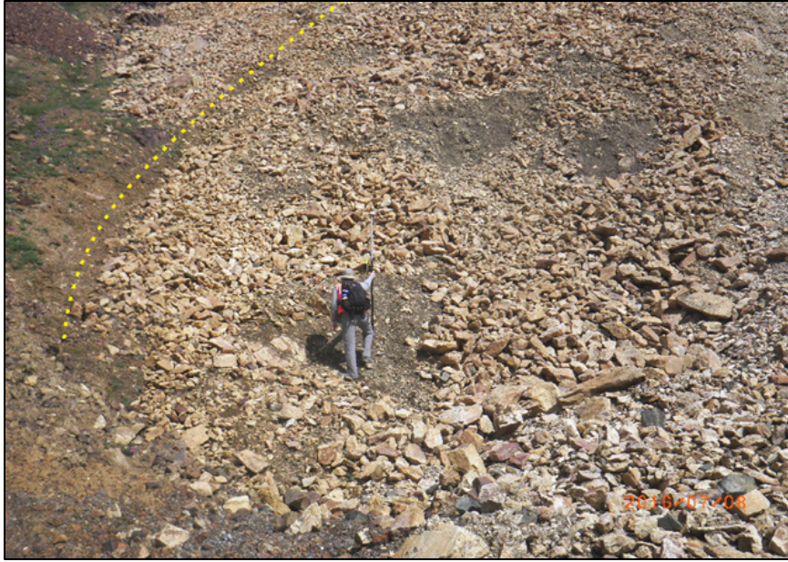
Figure 20. Northwestern boundary of failure area which divides the homogenous upper talus from the dissected slope below, and patches of slope which lack cobble- to boulder-sized clasts. Photo taken above the location of the northwestern road crack, looking north.
