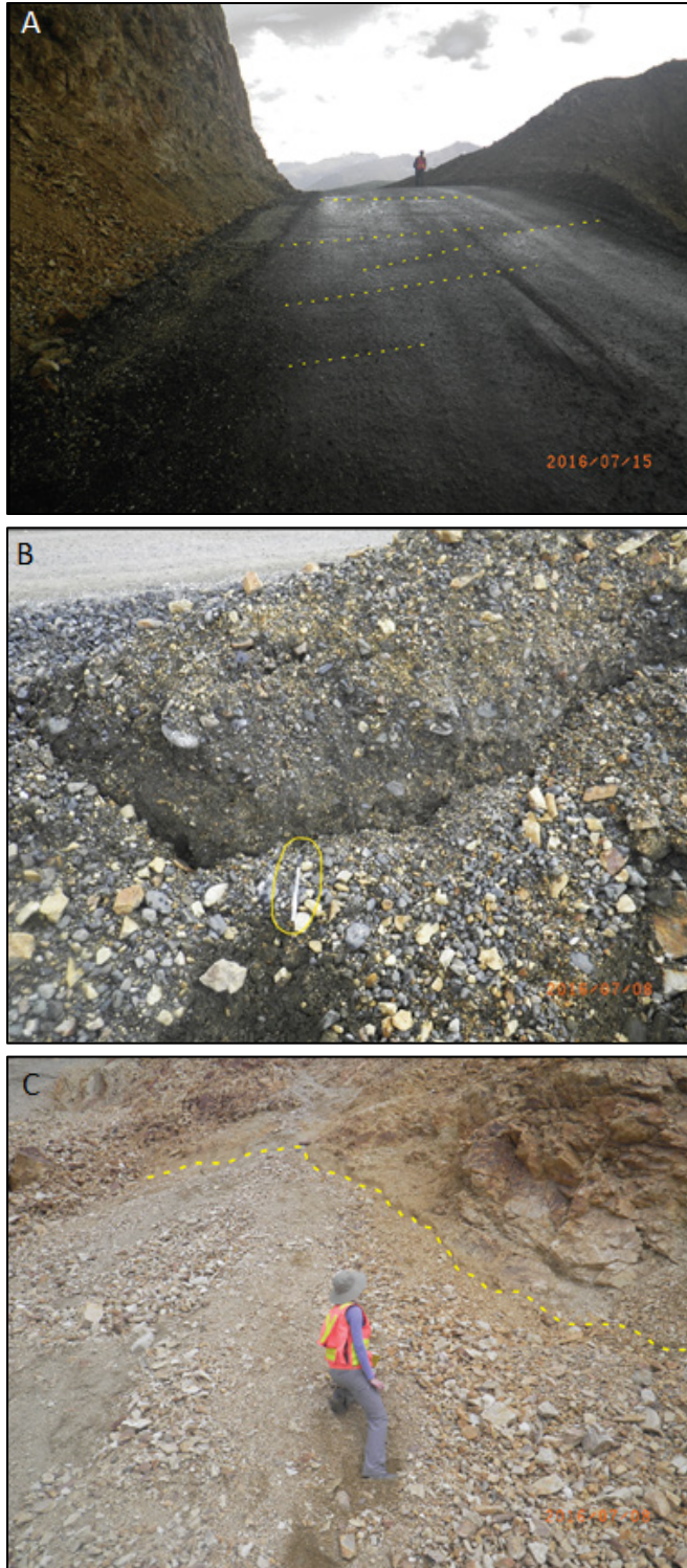
Figure 10. (A) Southeastern, en echelon road cracks. Highlights added for clarity. Photo taken looking southeast. (B) Detail of southeastern road crack where it continues below the road and turns easterly to propagate parallel to the road surface. Photo taken looking northeast. Pen for scale. (C) Outline of southeastern slide boundary upslope as defined by the crack between bedrock and colluvium. Crack is a continuation of southeastern road crack. Highlight added for clarity.
