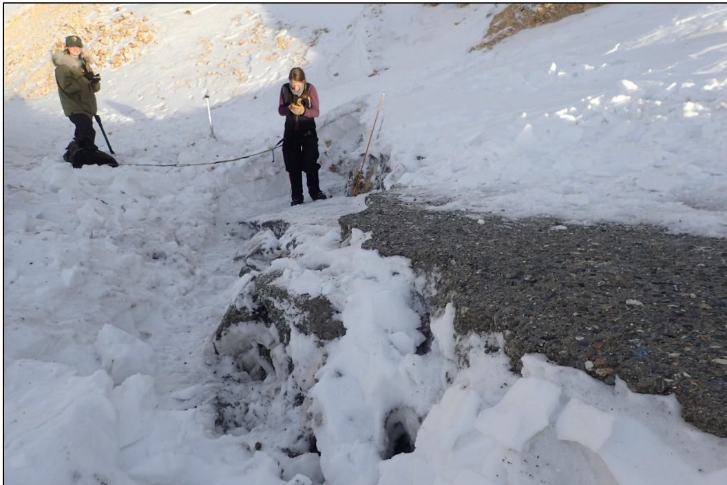
Figure 3. (TOP) Vertical offset along northwestern lateral scarp (i.e., road crack) in April 2004. (BOTTOM) Vertical offset along southeastern lateral scarp (i.e., road crack) in March 2018.
