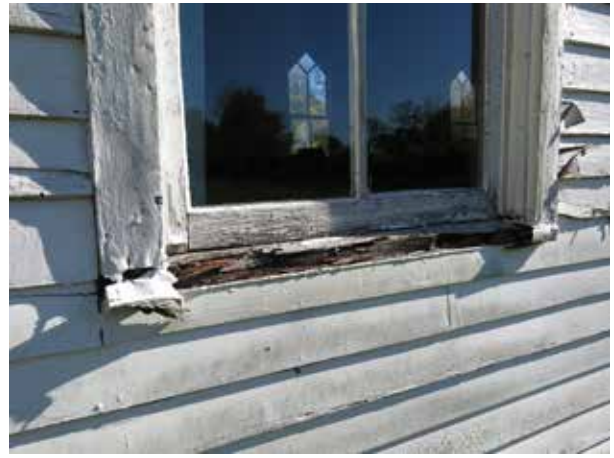
Figure 88. Extensive deterioration of sill and bottom sash 4 located at south elevation caused by lack of gutters and 5 downspouts to handle rainwater runoff from roof. (Source: 6 RATIO Architects, 2020) 7
