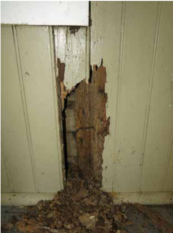
Figure 121. Detail of hole at north wall below east window as observed during site visit. This condition appears to be caused by insect damage and possibly by water infiltration. (Source: RATIO Architects, 2020)
