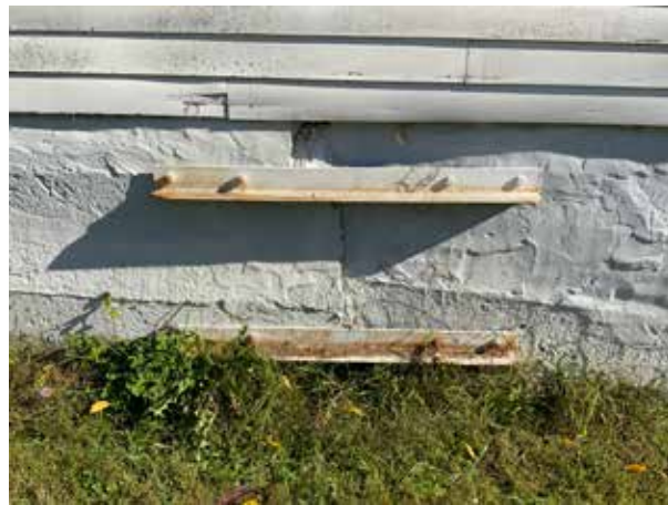
Figure 71. Angle irons in place at crack on south elevation. (Source: RATIO Architects, 2020)
