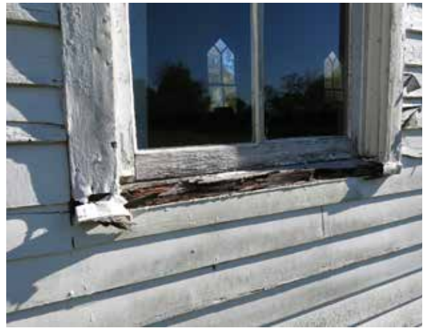
3 Figure 78. Detail of typical windowsill at south elevation. 4 Note extensive deterioration of sill and bottom sash caused 5 by lack of gutters and downspouts to handle rainwater 6 runoff from roof. (Source: RATIO Architects, 2020)
