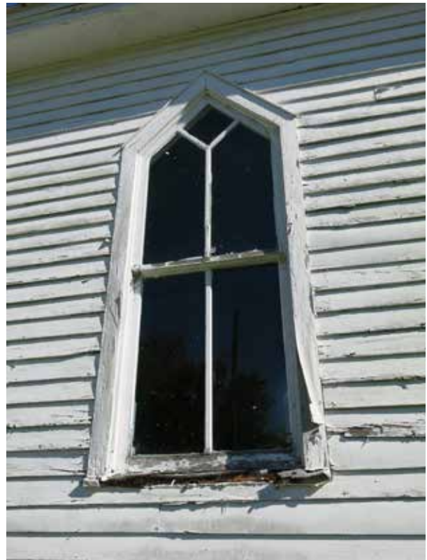
Figure 73. Typical "peak head" window at south elevation. Note typical deterioration of sill and bottom sash caused by lack of gutters and downspouts to handle rainwater runoff from roof. (Source: RATIO Architects, 2020)
