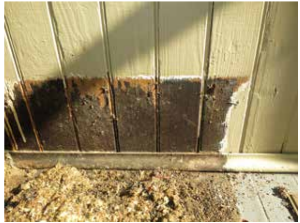
1 Figure 130. Detail of west face of dais after investigative 2 removal of south step. Note evidence of earlier finishes; The 3 debris is from a mouse nest that had been built inside the 4 step. (Source: RATIO Architects, 2020)
