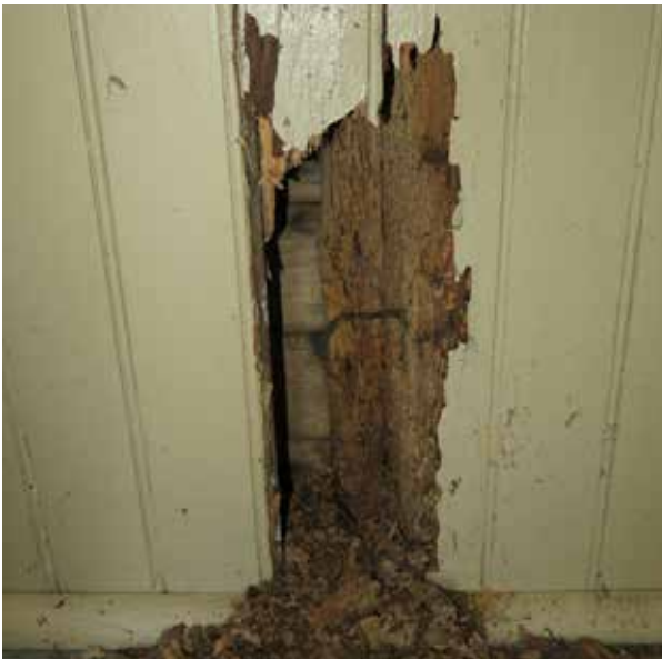
Figure 98. Detail of hole at north wall below east window as observed during site visit. This appears to be caused by insect damage and possibly by water infiltration. (Source: RATIO Architects, 2020)
