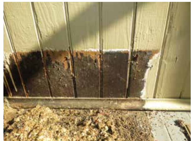
Figure 126. Detail of west face of dais after investigative removal of south step. Note evidence of earlier finishes. The debris is from a mouse nest that had been built inside the step. (Source: RATIO Architects, 2020)
