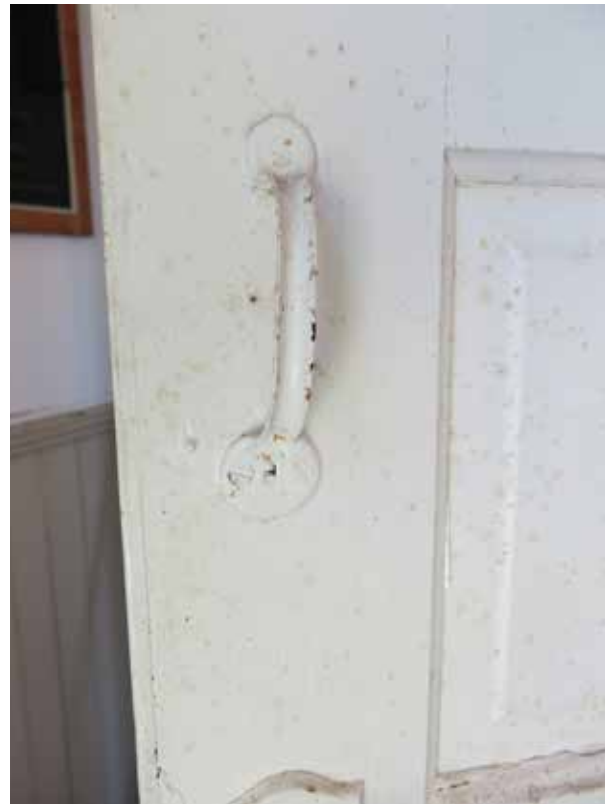
3 Figure 86. Detail of part of Suffolk latch installed upside- 4 down and used as a pull on vestibule door. (Source: RATIO 5 Architects, 2020)
