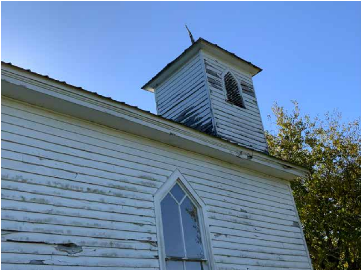
Figure 94. Detail of east and north elevations of cupola, showing paint deterioration. (Source: RATIO Architects, 2020)
