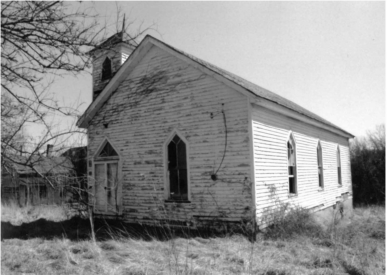
1 Figure 49. West façade and south elevation of Fee Memorial Church, ca. 1994-2000. This shows the deteriorated condition of 2 the church prior to the Jessamine County renovation. Note manse in distance at left. (Source: W. Stephen McBride) See Figure 3 47 for a similar view in 2020.
