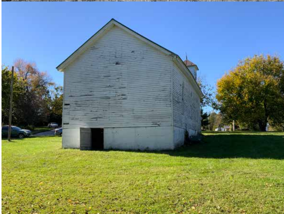
1 Figure 50. East and north elevations of Fee Memorial Church, ca. 1994-2000. This shows the deteriorated condition of the 2 church prior to the Jessamine County renovation. (Source: W. Stephen McBride) Similar view of the east and north elevations 3 in 2020. (Source: RATIO Architects)
