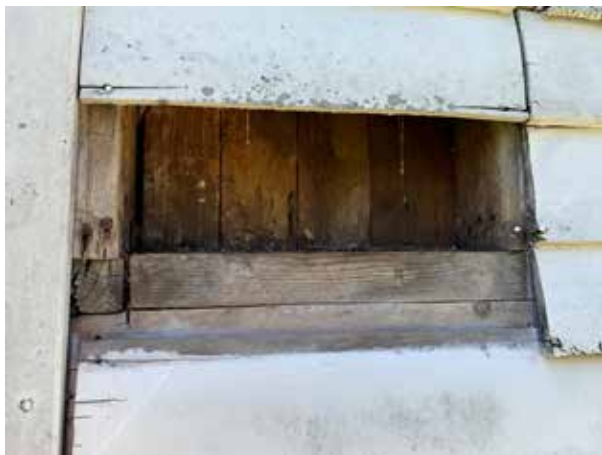
Figure 72. Detail of a missing section of siding at the south end of the east elevation, showing weatherboards nailed directly to studs with no sheathing. The back side of the interior wainscoting is visible between the studs. (Source: RATIO Architects, 2020)
