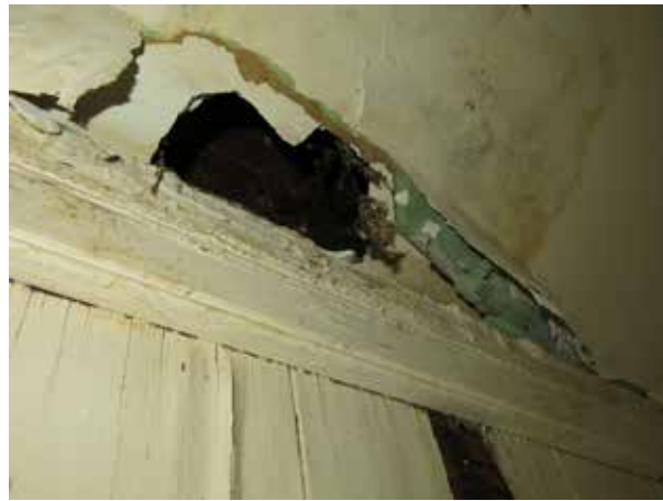
Figure 115. Detail of damage to lower edge of sloped ceiling along north wall; note fibrous paper with pale greenish-blue paint finish. (Source: RATIO Architects, 2020)
