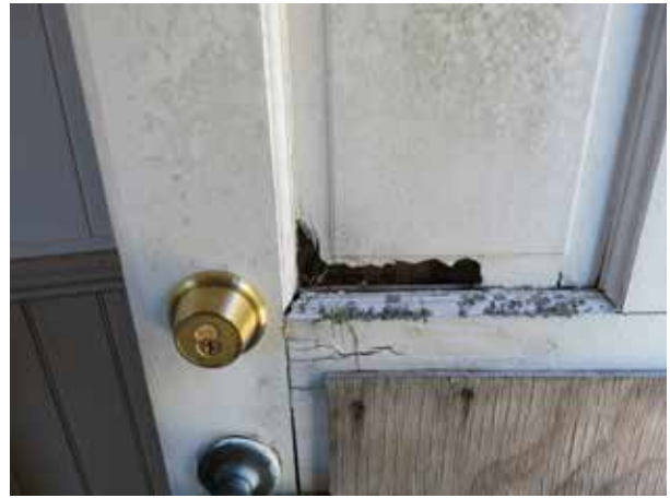
Figure 83. Typical deterioration at modern wood replacement doors. (Source: RATIO Architects, 2020)
