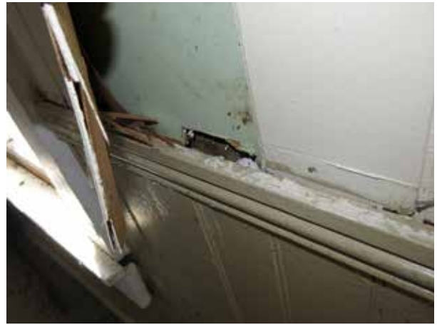
Figure 122. Detail of wall surface behind loose paneling at west wall of sanctuary; note pale greenish-blue paint over fibrous paper. (Source: RATIO Architects, 2020)
