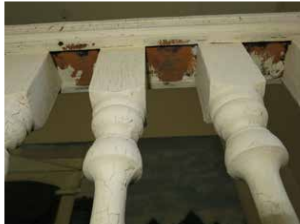
26 Figure 128. Detail of south section of dais balustrade 27 showing evidence of earlier finishes. (Source: RATIO 28 Architects, 2020)
