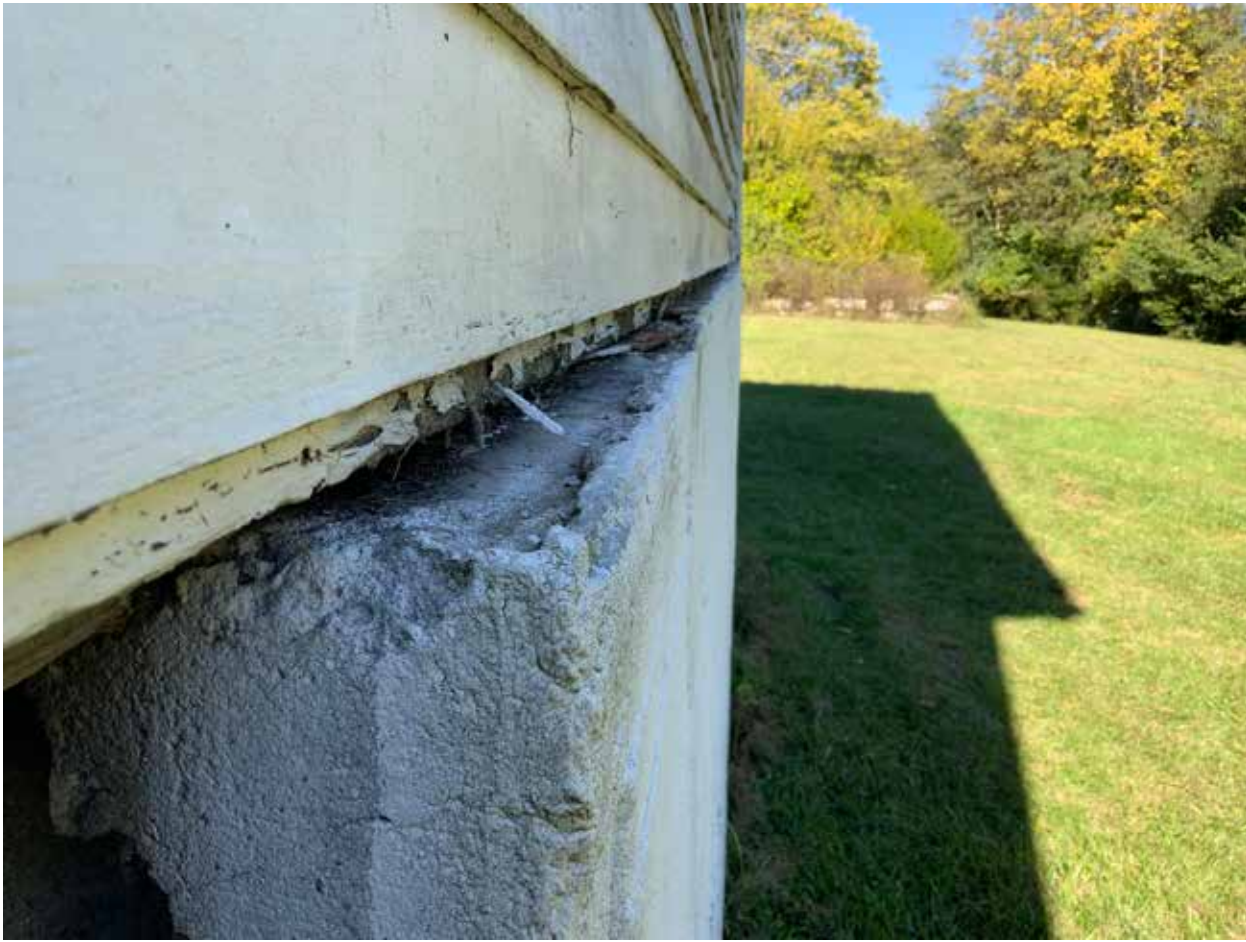
1 Figure 97. Detail of displacement at east face of foundation, facing north. (Source: RATIO Architects, 2020)
