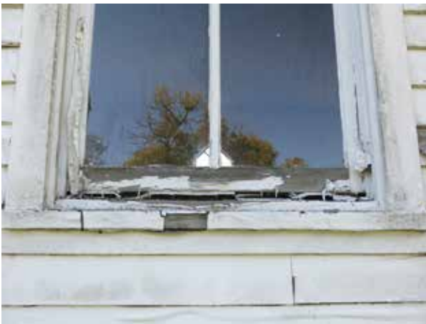
7 Figure 79. Detail of typical windowsill at north elevation. 8 Note typical deterioration of sill and bottom sash caused by 9 lack of gutters and downspouts to handle rainwater runoff 10 from roof. (Source: RATIO Architects, 2020)
