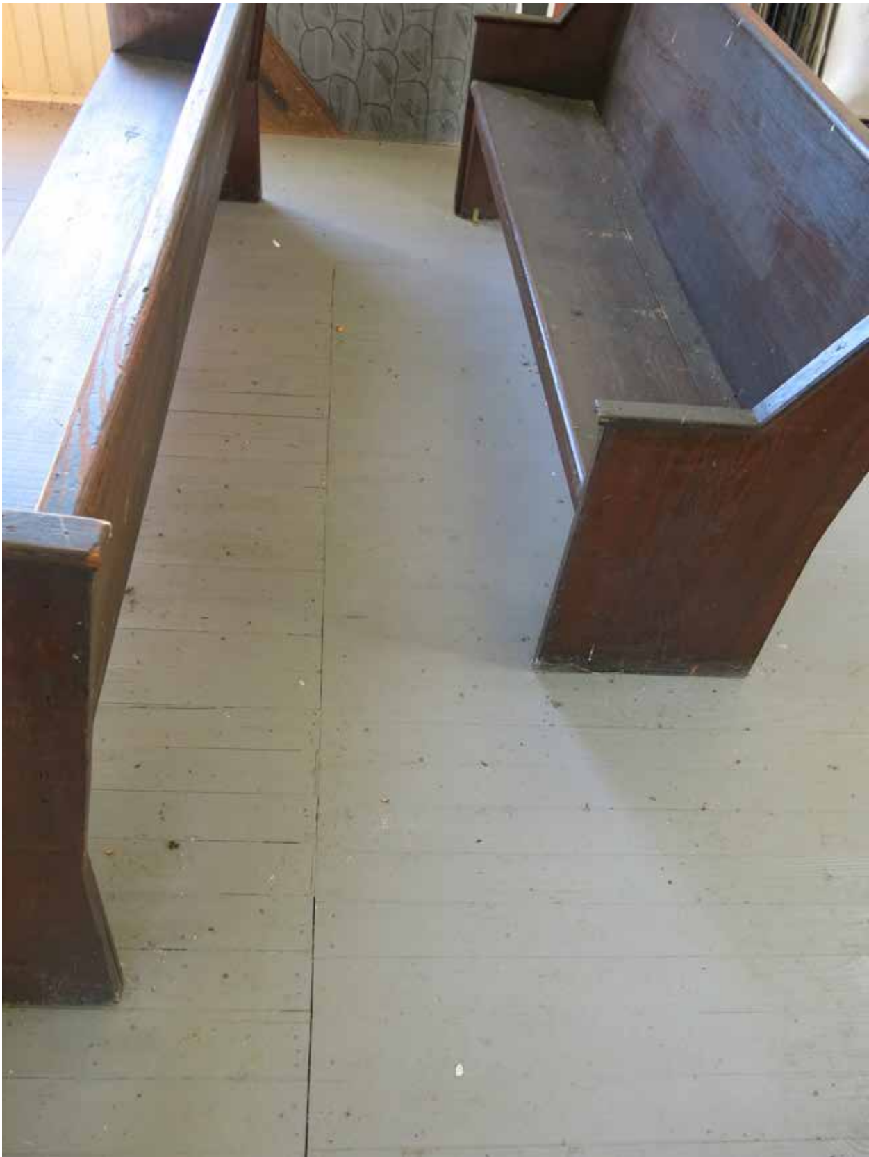
1 Figure 124. Seam at sanctuary floor, facing southeast. (Source: RATIO Architects, 2020)
