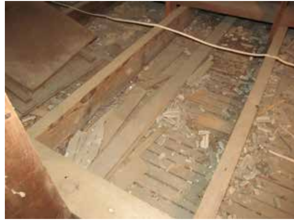
4 Figure 134. View of sanctuary ceiling south of vestibule, 5 facing southeast; note broken plaster keys and snakeskin at 6 left. (Source: RATIO Architects, 2020)
