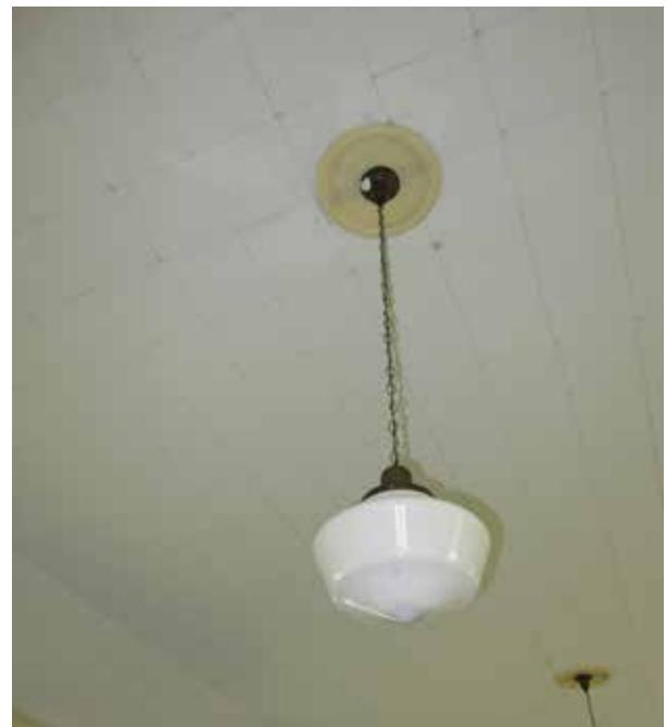
Figure 107. Typical "schoolhouse"-type electric pendant. (Source: RATIO Architects, 2020)
