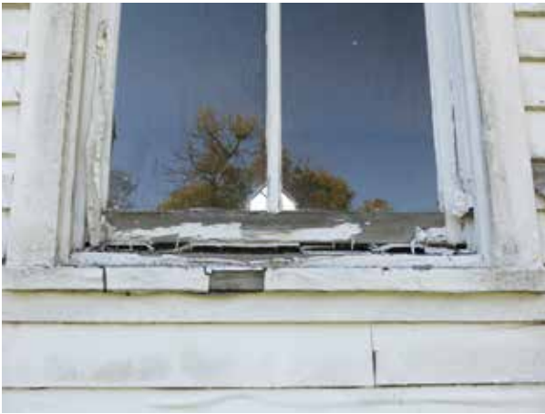
8 Figure 89. Typical deterioration of sill at north elevation 4 9 and bottom sash caused by lack of gutters and downspouts 5 10 to handle rainwater runoff from roof. (Source: RATIO 6 11 Architects, 2020) 7
