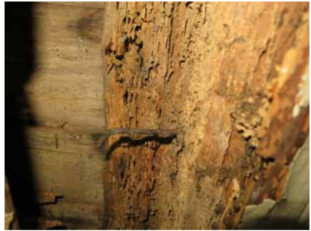
Figure 99. View inside hole at north wall showing deterioration of wall framing. Note wire nail now exposed. (Source: RATIO Architects, 2020)
