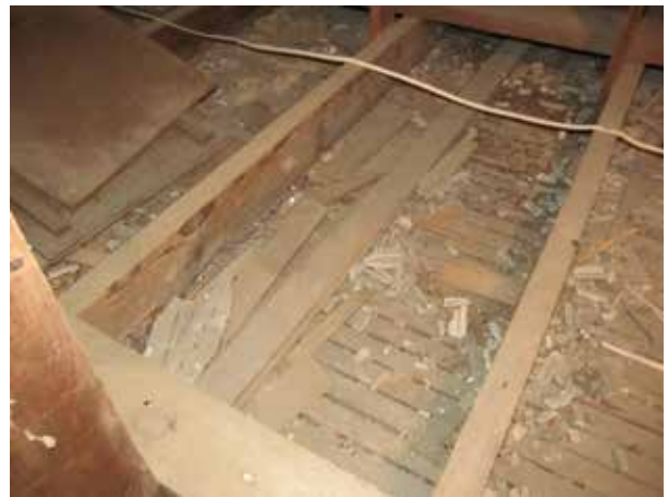
Figure 123. View of sanctuary ceiling south of vestibule, facing southeast; note broken plaster keys and snakeskin at left. (Source: RATIO Architects, 2020)
