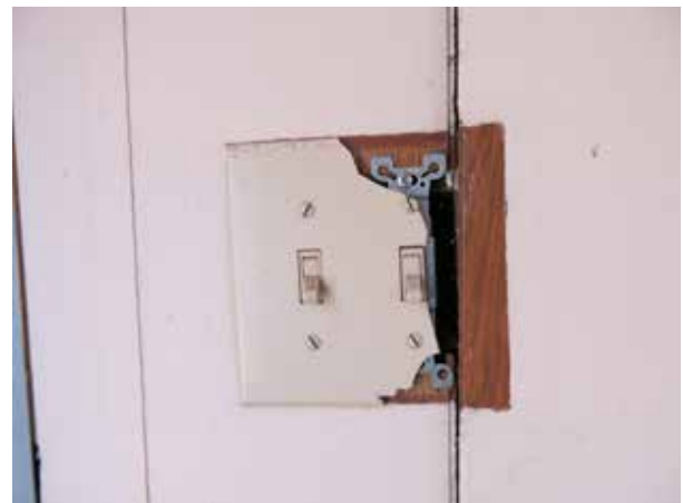
Figure 109. Detail of damaged light switch cover at north wall of vestibule showing stained finish of modern plywood paneling below ca. 2000-2005 paint finish. (Source: RATIO Architects, 2020)
