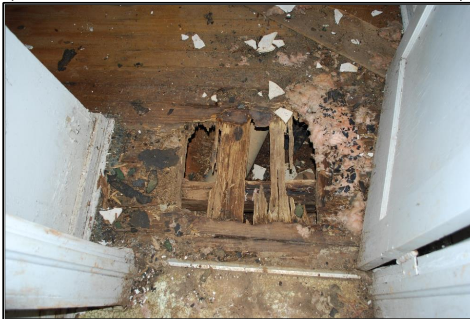
Figure 28. House interior: View of hole in floor of Room 105 showing floor joist and decaying original flooring. Photograph taken October 29, 2019, by Trent Spurlock.
