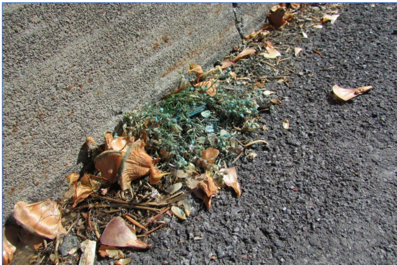
Figure 9. Red sand-spurrey growing out of the pavement in the Annie Creek Restaurant parking lot after being sprayed with a blue herbicide mixture. Photo by Alexandra von Bergman.
