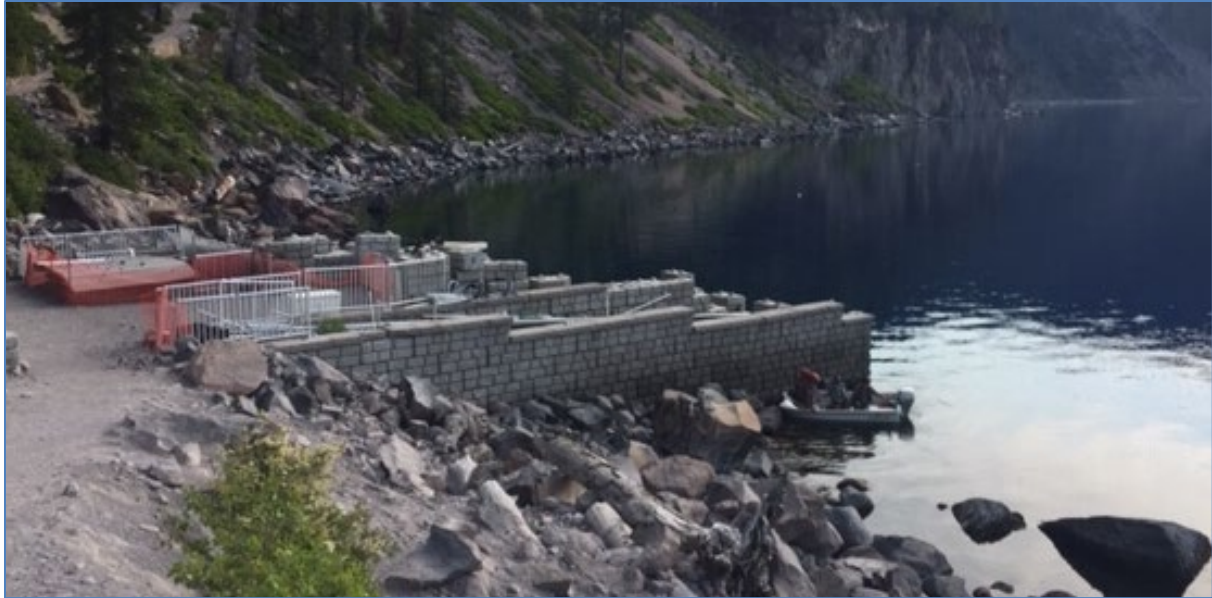
Figure 4. View of Crater Lake's shoreline with failed dock and bulkhead. Photo by Carrie Wyler.
