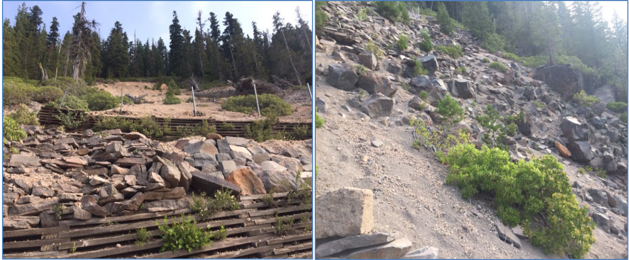
Figure 2. Deteriorated cribbing and rock retaining wall (left); unstable, rocky pumice soils (right) on the Cleetwood Cove trail. Photos by Carrie Wyler.
