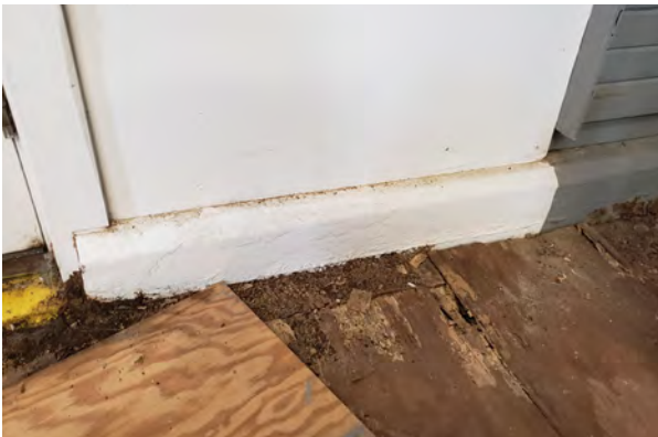
Figure 2.148. Plywood flooring in Room 103. Note termite and water damage.
