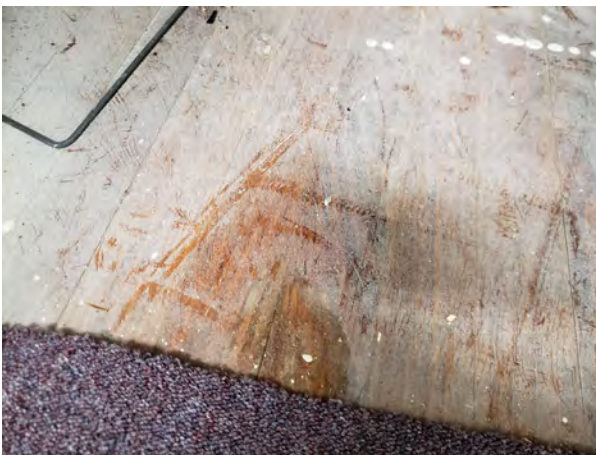
Figure 2.99. Wood flooring in closet of Room 204. Note paint overspray.
