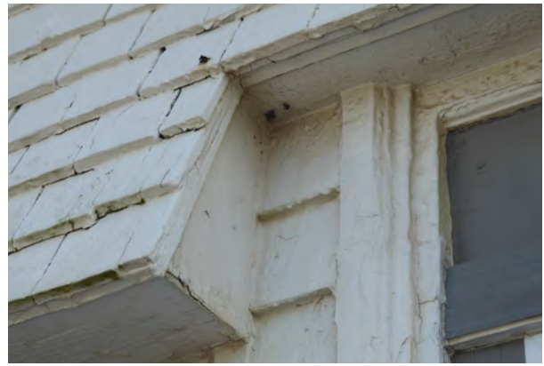
Figure 2.20. Flare in siding at north elevation boat doorways. This detail is expected to have been moved from the south elevation.
