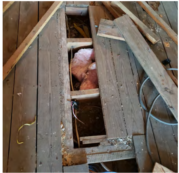
Figure 2.114. Partially exposed opening where chimney extended through floor. Newer blocking now spans the opening.
