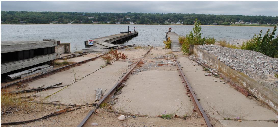
The Launchway to the west of the study area is in poor condition (source: Mundus Bishop, 2019)
