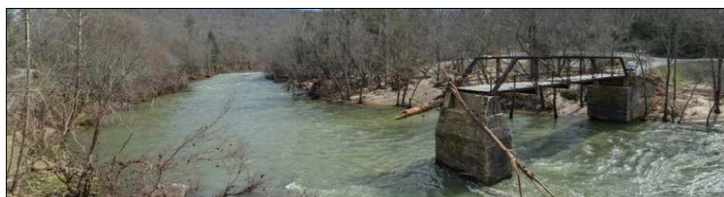
Burnt Mill Bridge on Clear Fork damaged from the March 2021 flooding. NPS photo / APHN staff.
