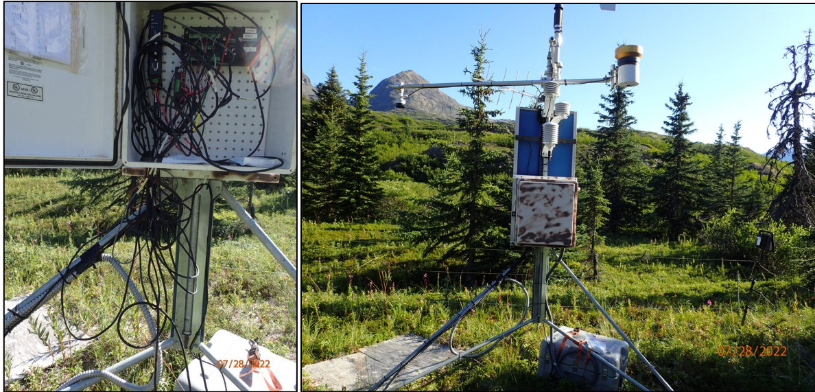
Figure 10. Tebay climate station, July 28, 2022. Site had been damaged (left). Station after site maintenance was completed (right).
