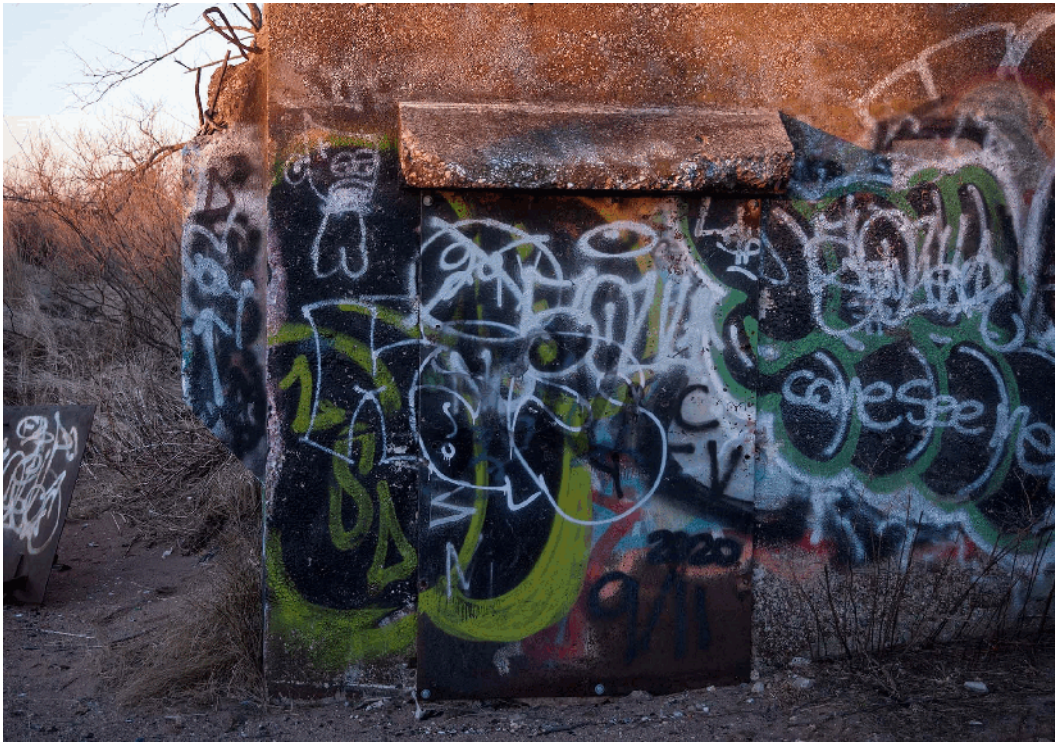
Figure 37 Miller Field Fire Control Tower, Detail of Northeast Façade Entrance and Damaged Ventilation Inlet, Facing Southwest (Attenborough 2022).
