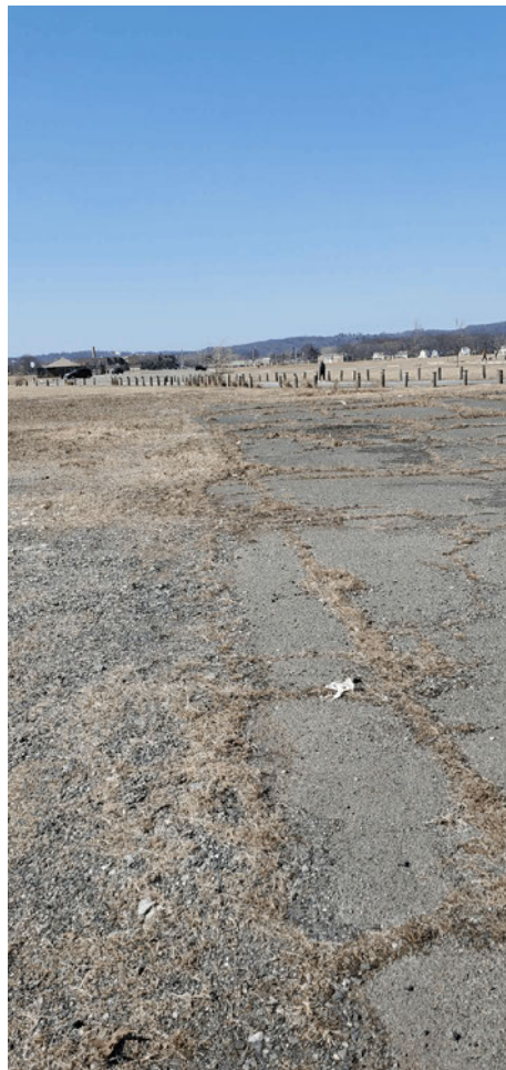
Figure 6 View of the portion of the Miller Field shovel test area between the Concrete Apron and Cedar Grove Avenue showing the decaying paving, facing northwest (Image 130802: March 2, 2022).
