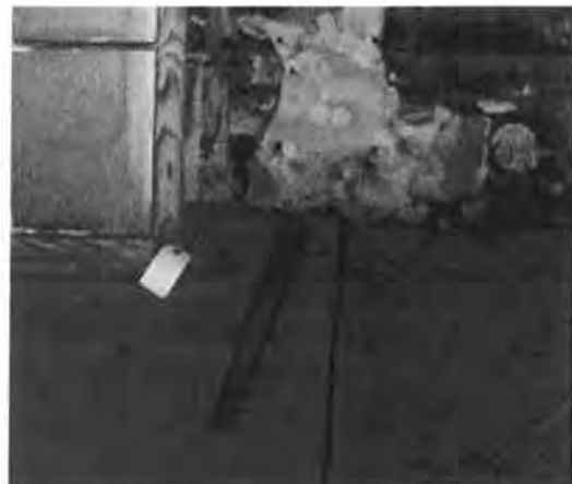
Flooring joint, Room 103
