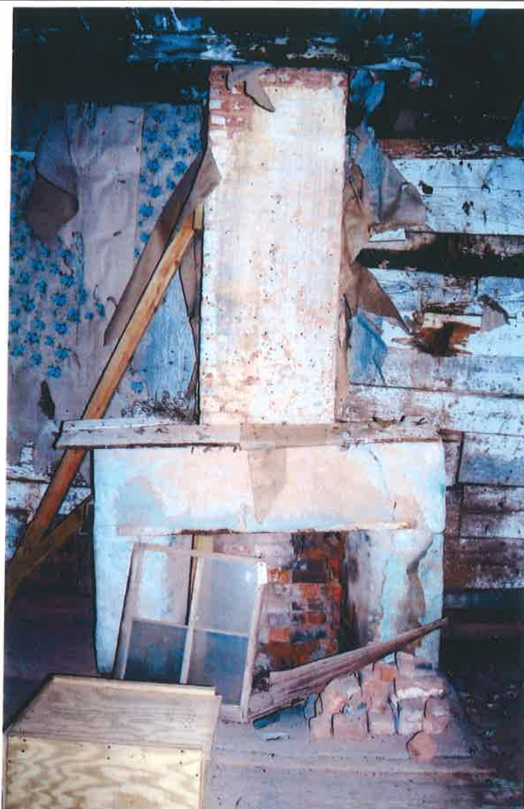
Image 87: Oakland Plantation. South Tenant Cabin, Room 102, 2002. The chimney has bousillage plaster on it while the mantle is made of hard cement with modern blue paint.
