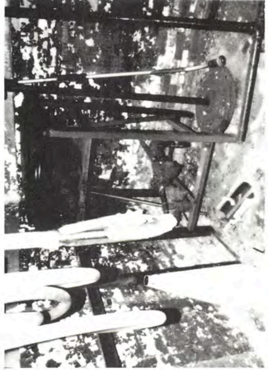
Photo 3-48 View of insulation material, probably asbestos, on pipes.
