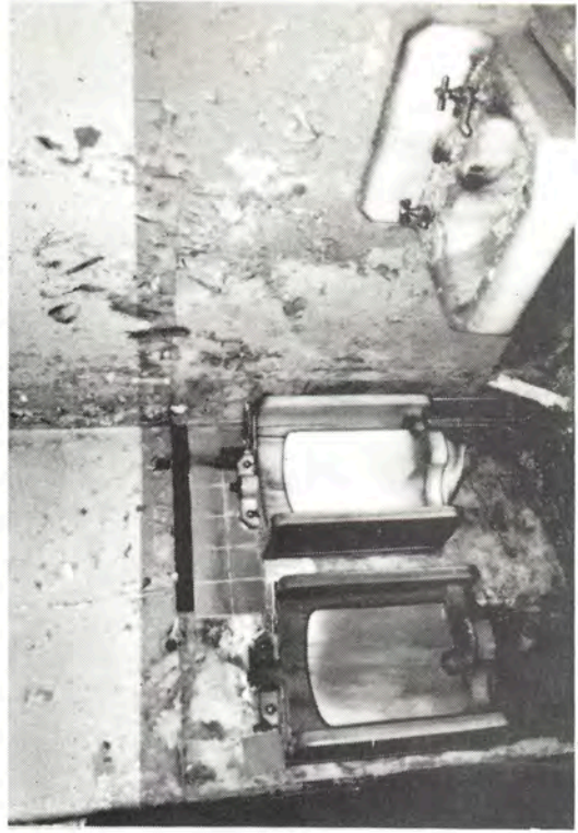
Photo 3-56 Typical view of the deteriorated condition of the existing plumbing fixtures
