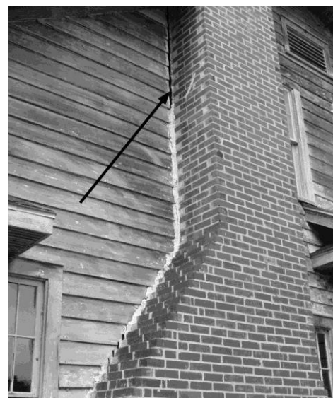
Figure 9 View of chimney; arrow indicates gap between masonry and the wall of the house. (NPS-SERO-CRS, 2002)
