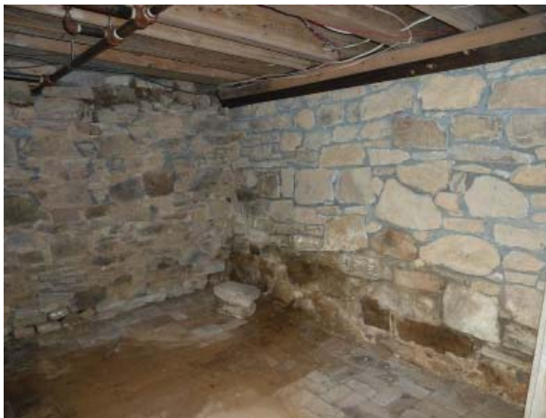
Figure 96. Southwest oblique of Room 001 showing moisture problem on west wall.
