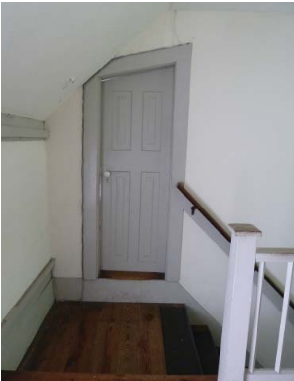
Figure 127. The doorway off of the Upper Stair Hall (Room 202) connecting to the Central Bedroom (Room 203). Note the door is hung upside down.
