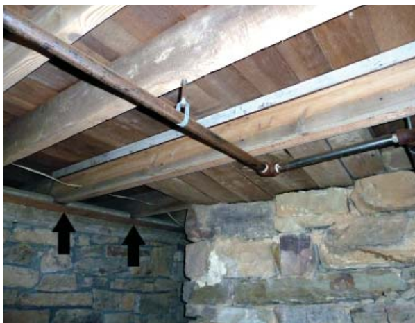
Figure 69. First-floor joists extend beyond the west foundation wall in Rooms 001 and 002.
