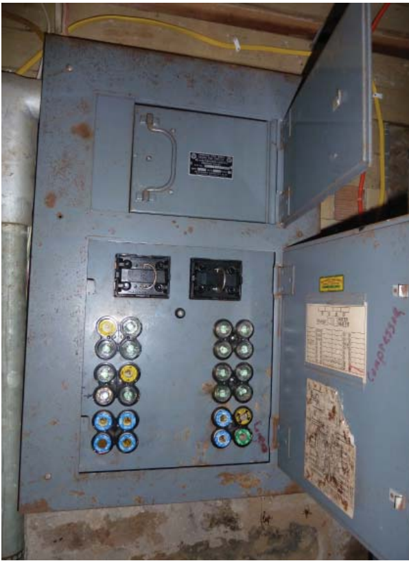
Figure 74. Electrical panel in the Utility Room (Room 003B).
