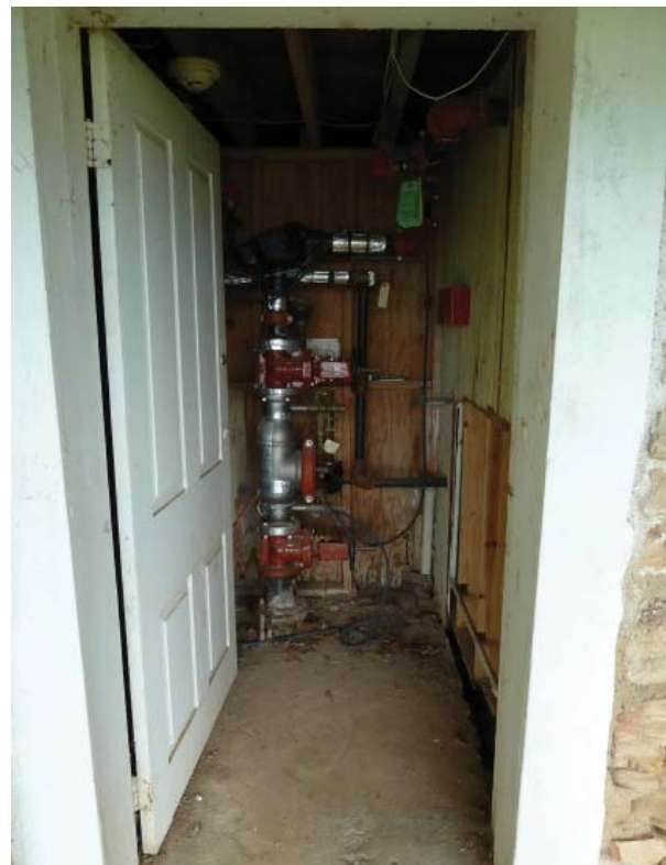
Figure 104. View of west wall of Utility Room (Room 003B) and the pump for the fire suppression system.
