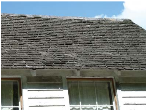
Figure 77. Failing shingles of the main roof.
