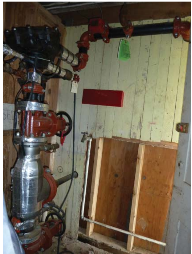
Figure 76. Water pump for the fire suppression system in the Utility Room (Room 003B).
