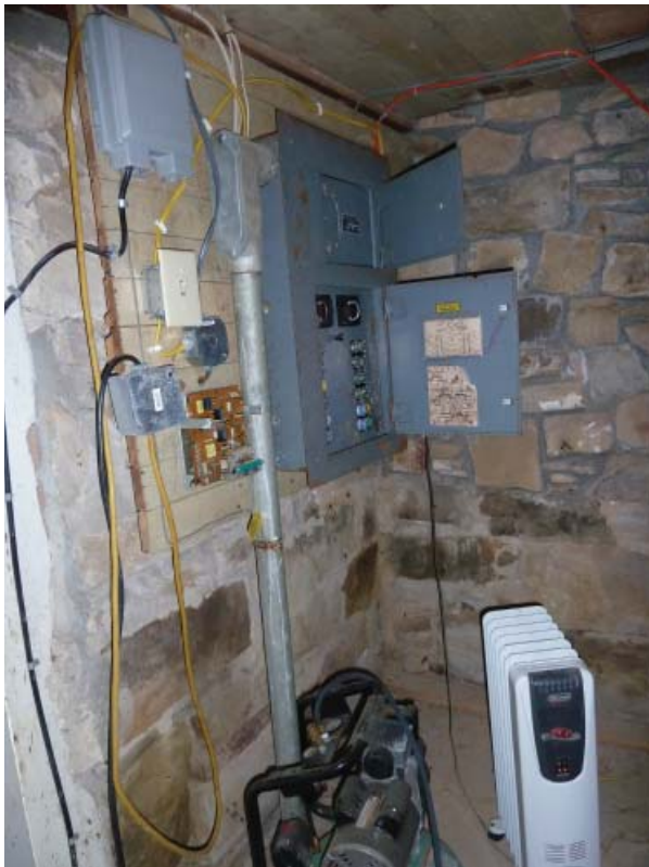
Figure 105. Electrical panel of Utility Room (Room 003B).
