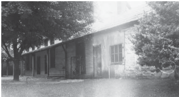
Figure 31. Photograph accompanying 6/18/1946 Quarters Report showing the poor condition of the house. (CHCH Acc 212, Folder 38)
