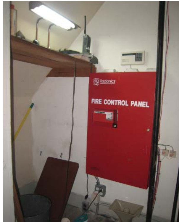
Figure 118. The fire control panel and security panel on the north wall of the stair closet of the Central Parlor (Room 103).
