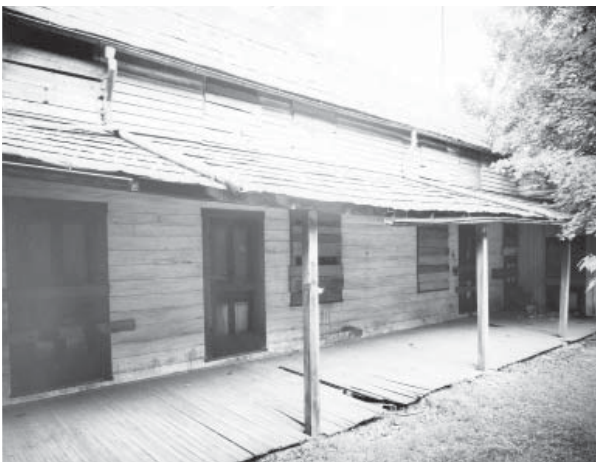
Figure 36. Pre-restoration photograph taken in 1956 showing west elevation of the connector. Doors and windows are boarded over. Porch and gutter system in poor condition. (CHCH Collection)
