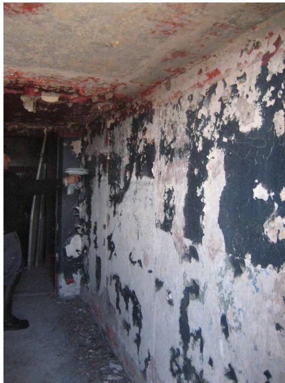
Fire-control Bunker B: Peeling blue paint on interior concrete walls.
