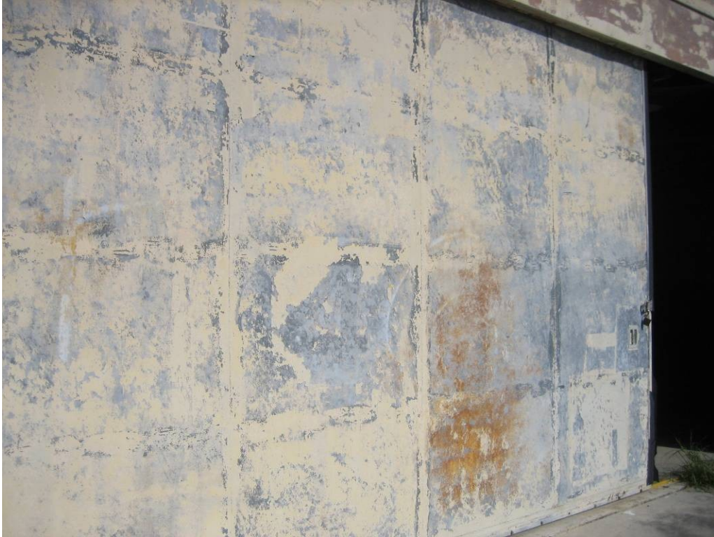
Missile Barn B: Peeling pink (beige) paint on exterior metal barn doors.
