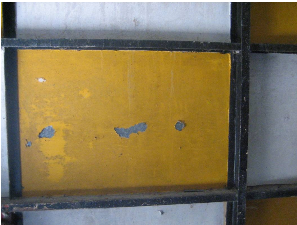
Missile Barn A: Chalking yellow paint on interior of barn door.
