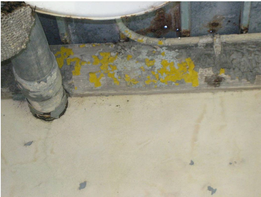
Sign/Generator Building 190A: Peeling yellow paint on wood header above bathroom door.
