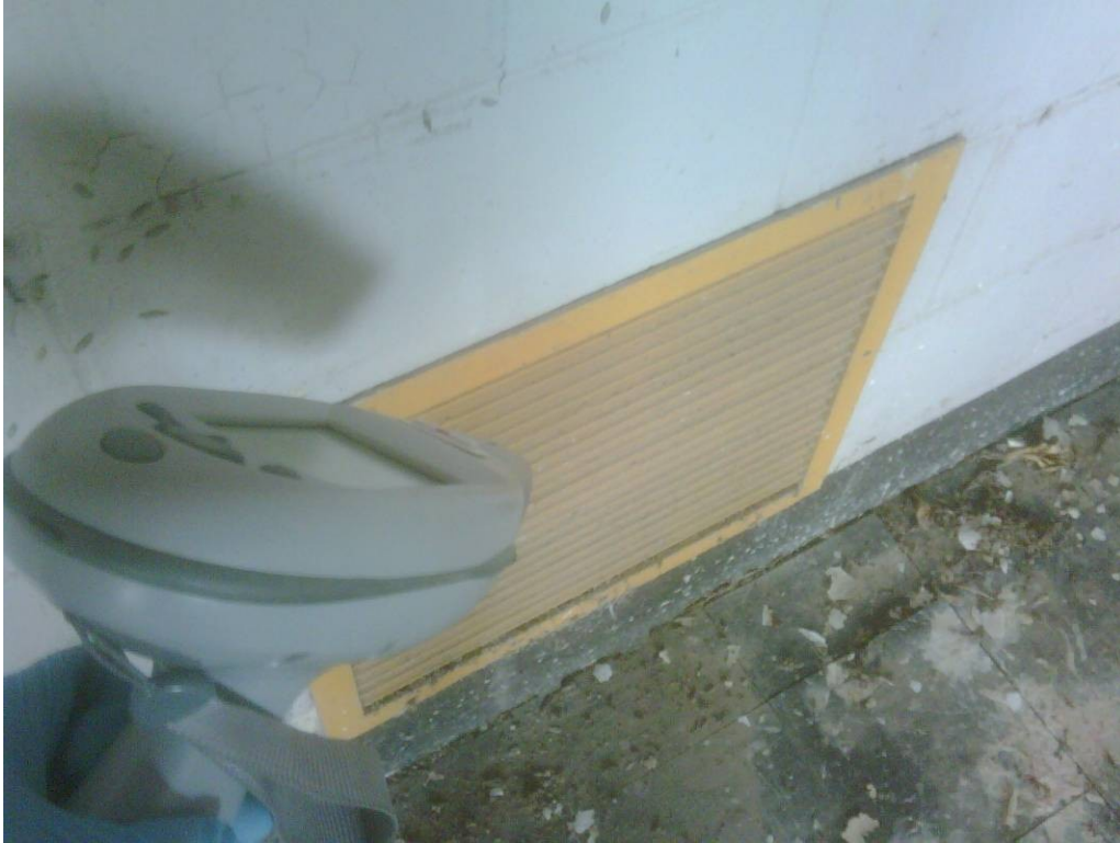
Missile Assembly Building: Peeling yellow paint on air conditioning vent.
