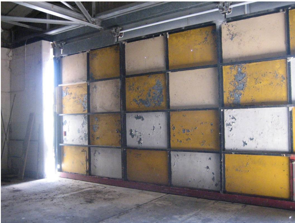
Missile Barn A: Chalking yellow and white paint on interior of barn door.
