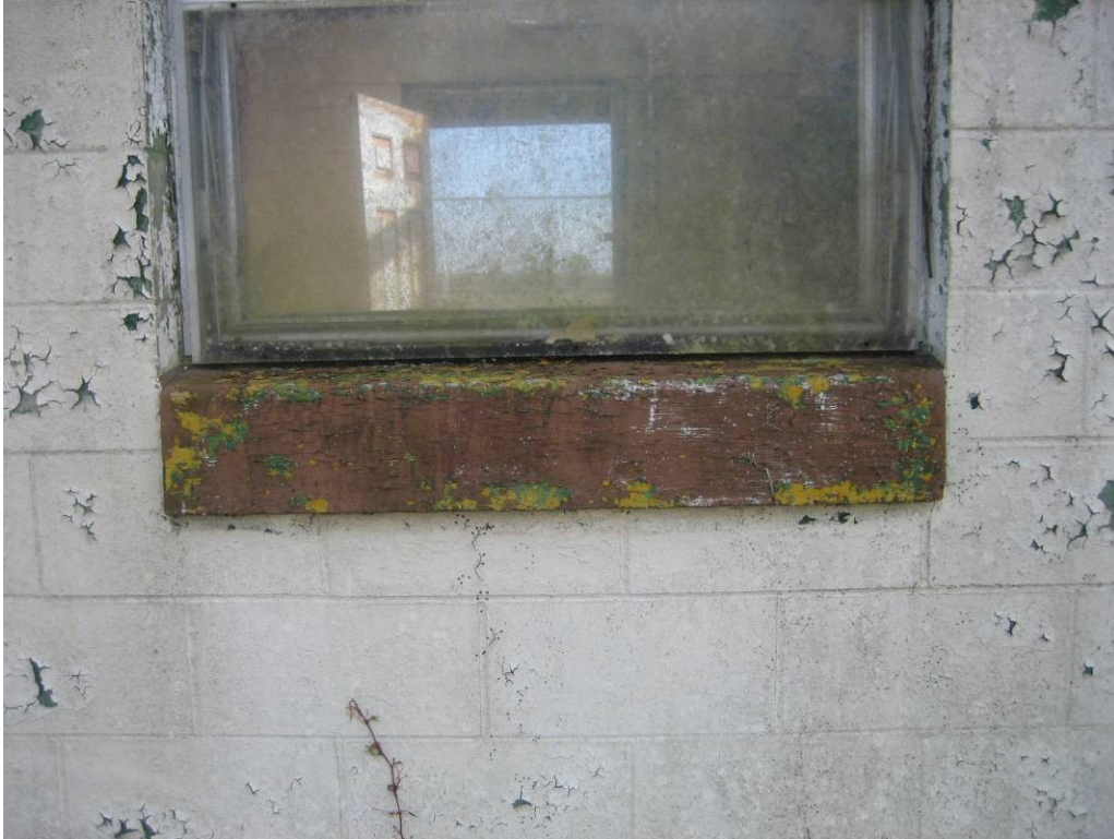
Kennel Building: Peeling brown (yellow) paint on exterior window sill.
