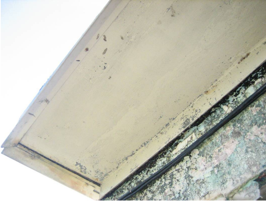
Sign/Generator Building 190A: Cracked beige paint on metal eve soffit.
