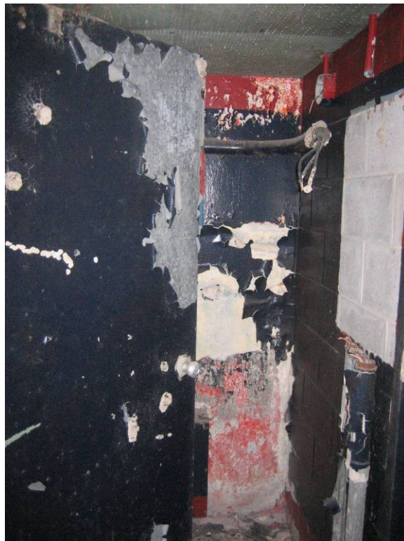
Fire-control Bunker B: Peeling gray paint on interior metal door.
