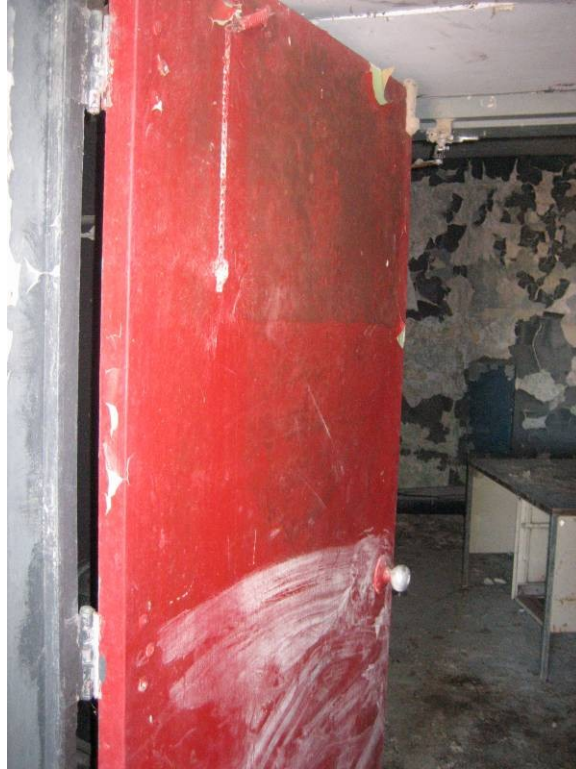
Fire-control Bunker A: Cracked red paint on interior metal door.
