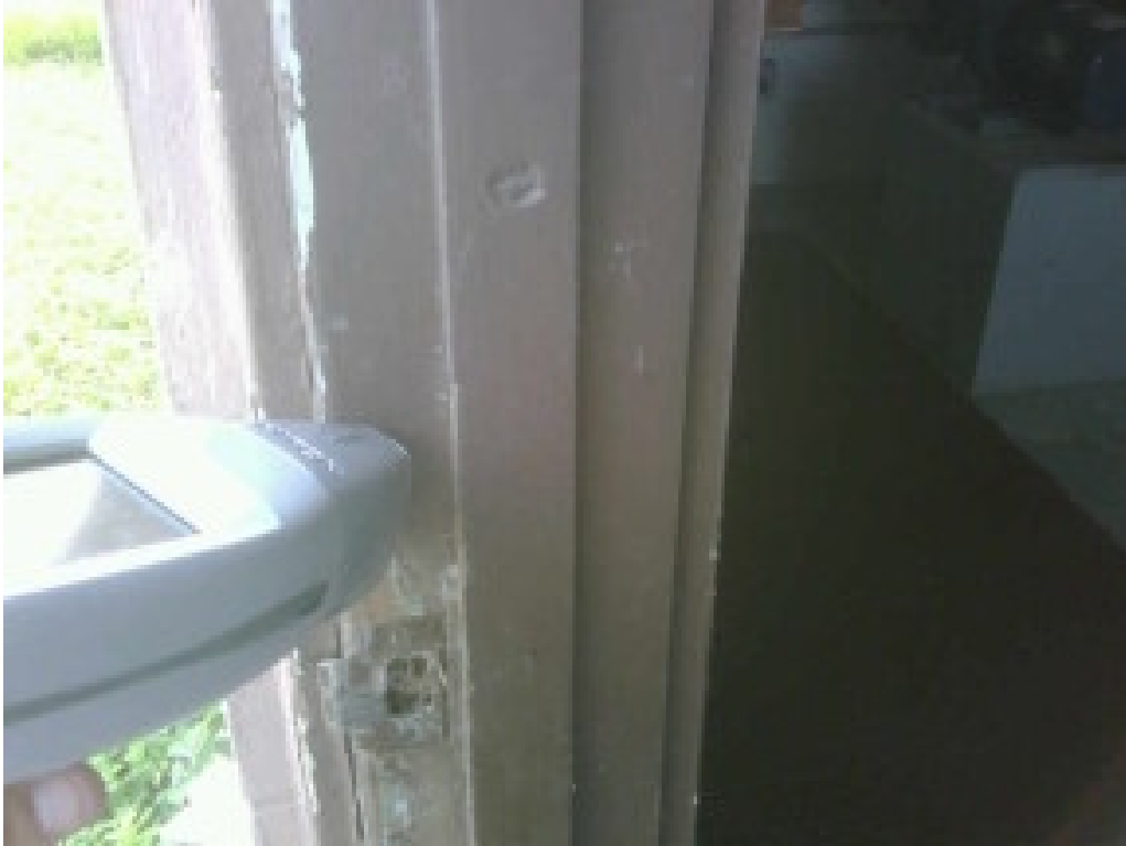
Water Pump House: Brown paint on wood door jamb.
