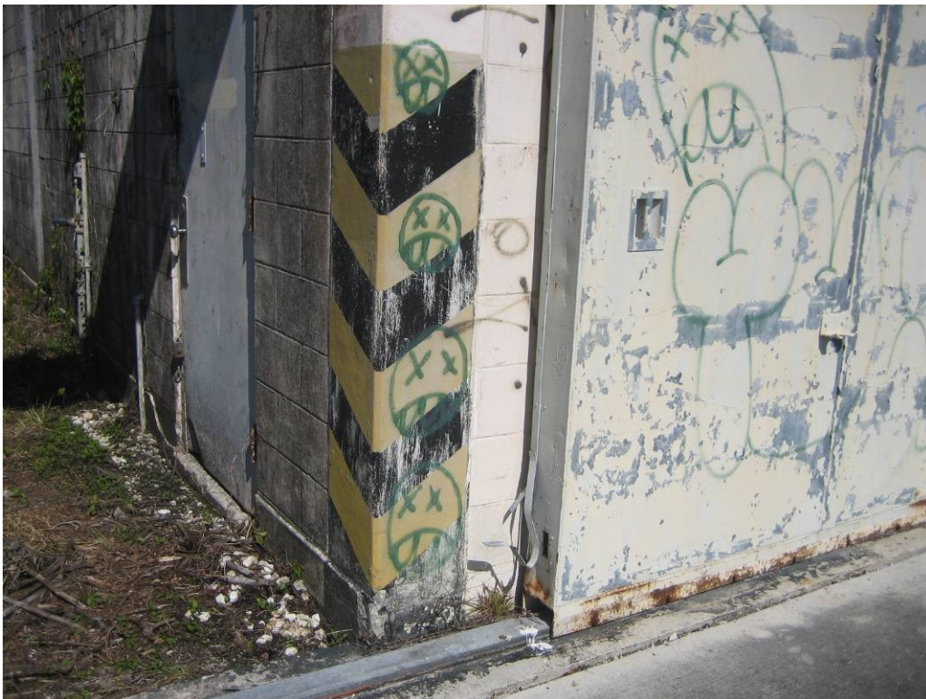
Missile Barn A: Peeling yellow paint on concrete block.
