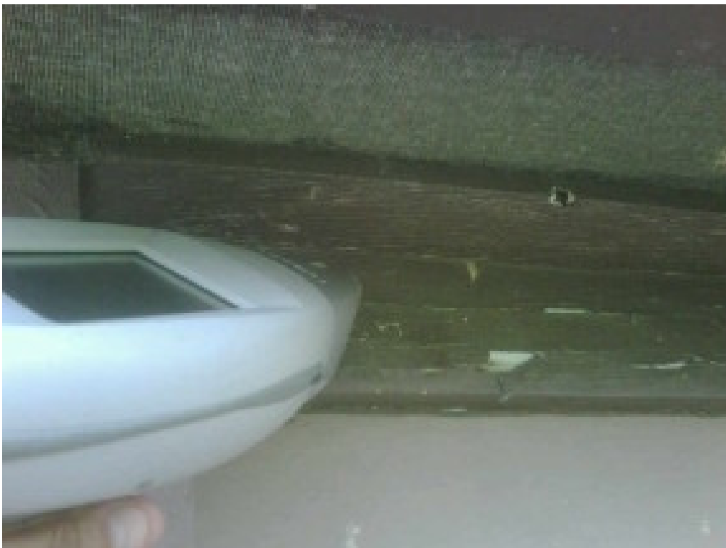
Water Pump House: Brown paint on wood header.
