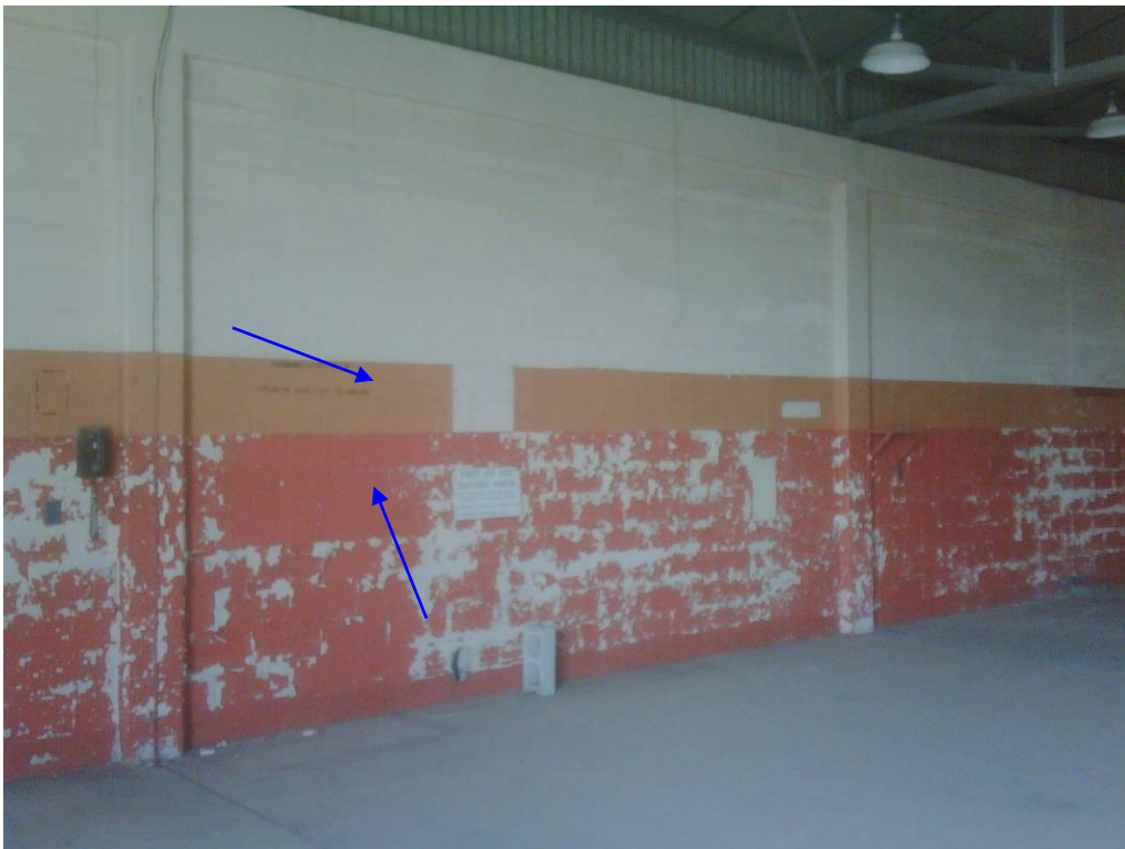
Missile Barn C: Peeling red and orange paint on concrete block wall.
