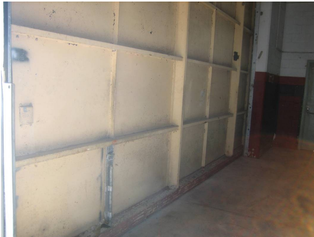
Missile Barn B: Peeling pink paint on interior of barn door.
