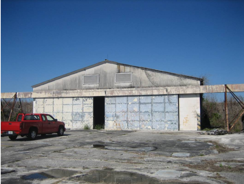
Missile Barn A: Peeling pink paint on exterior metal barn doors.
