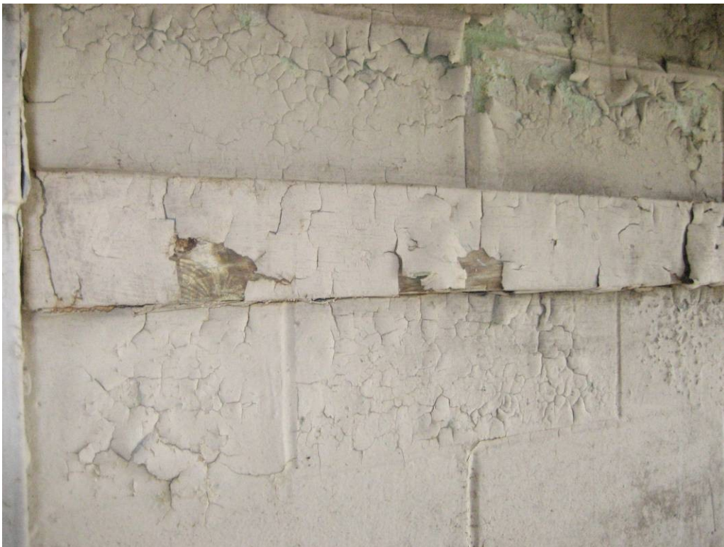
190B Building: Cracked/peeling beige paint on interior concrete block walls.
