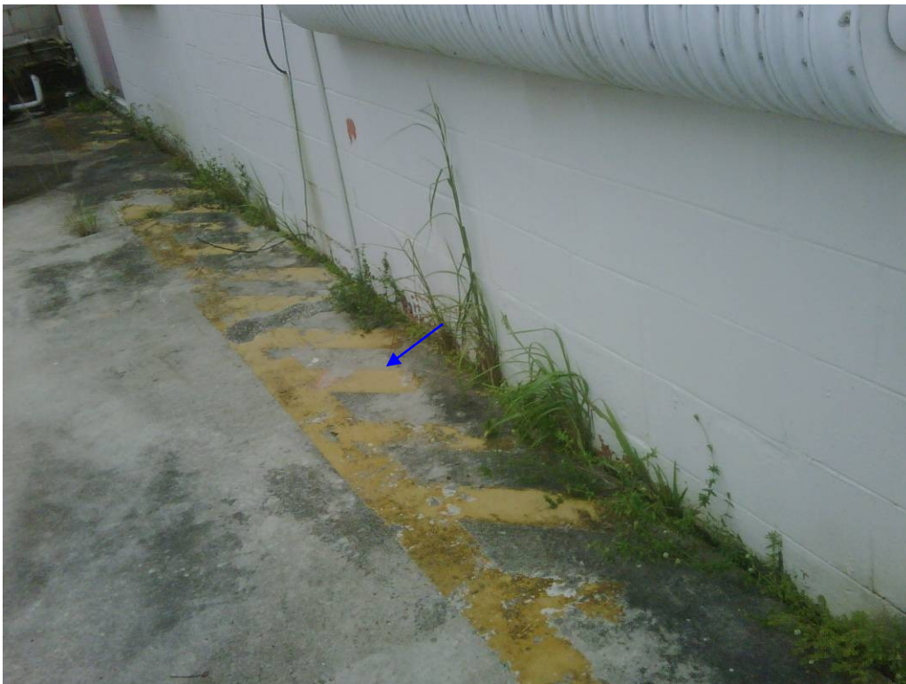
Administration Building: Yellow caution paint on sidewalk.
