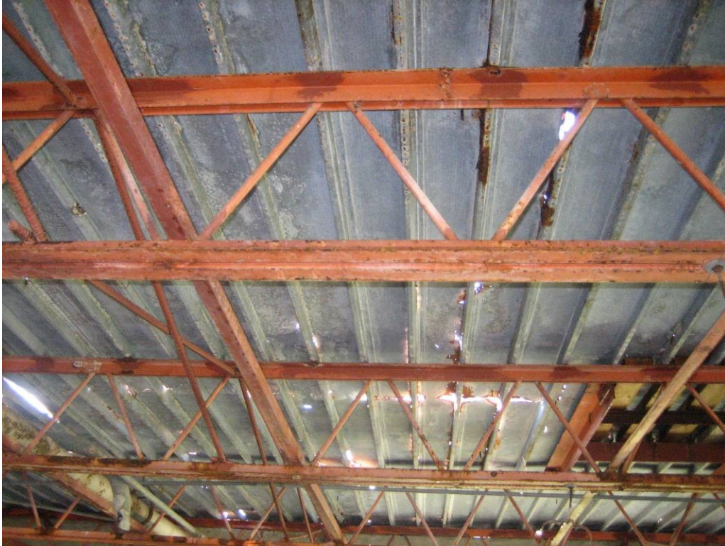
Sign/Generator Building 190A: Red paint on interior metal support beams.
