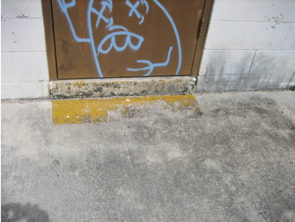
Missile Assembly Building: Peeling yellow paint on exterior concrete slab.
