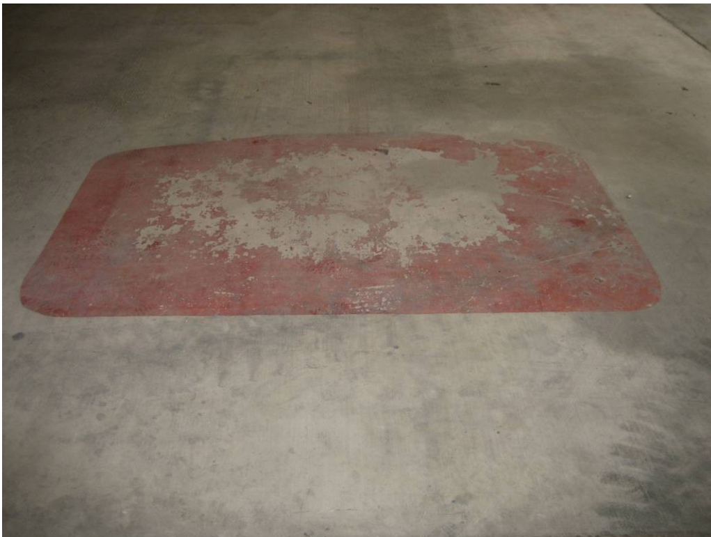
Missile Barn B: Red paint on concrete floor.
