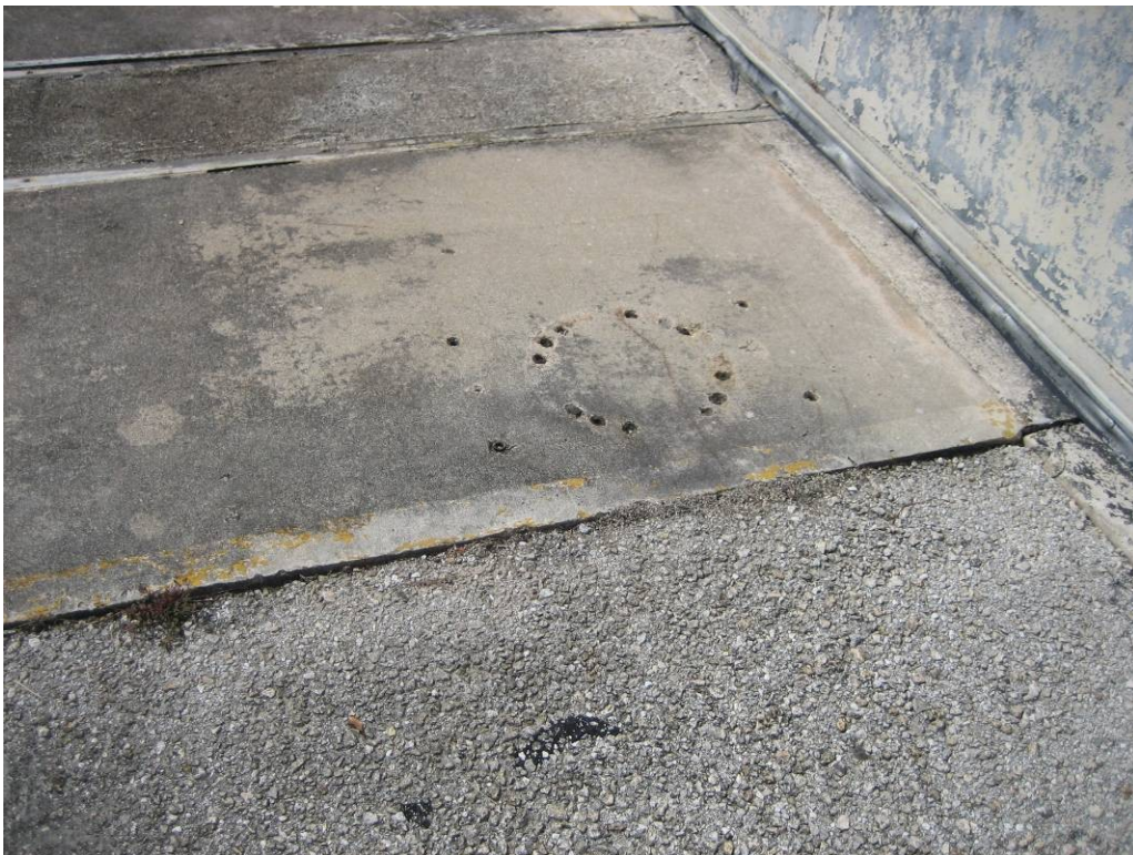
Missile Barn C: Chalking yellow paint on concrete slab.
