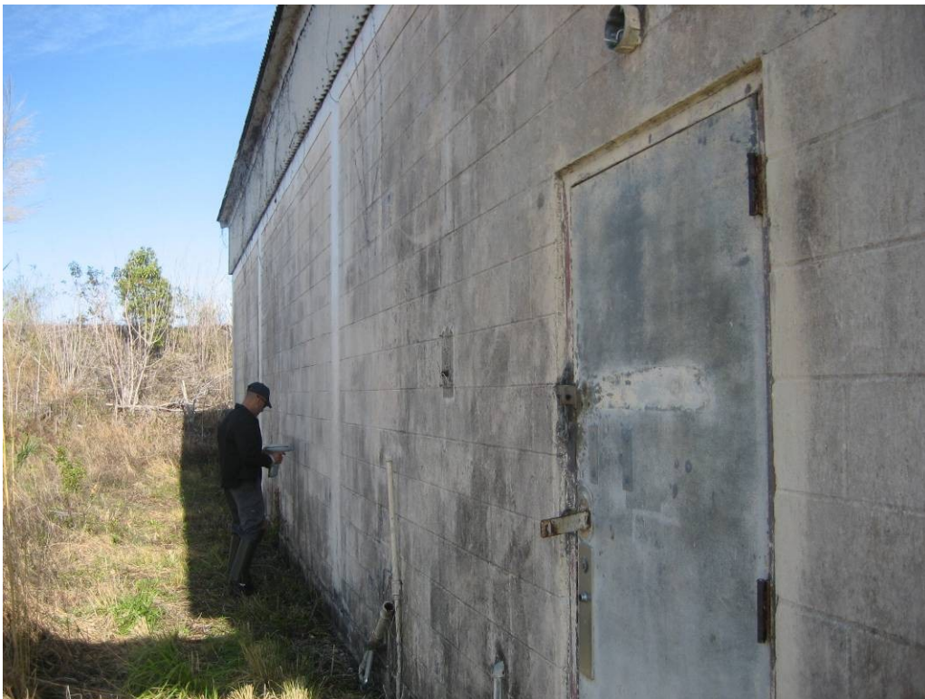
Missile Barn B: Chalking pink exterior paint on concrete walls and columns.
