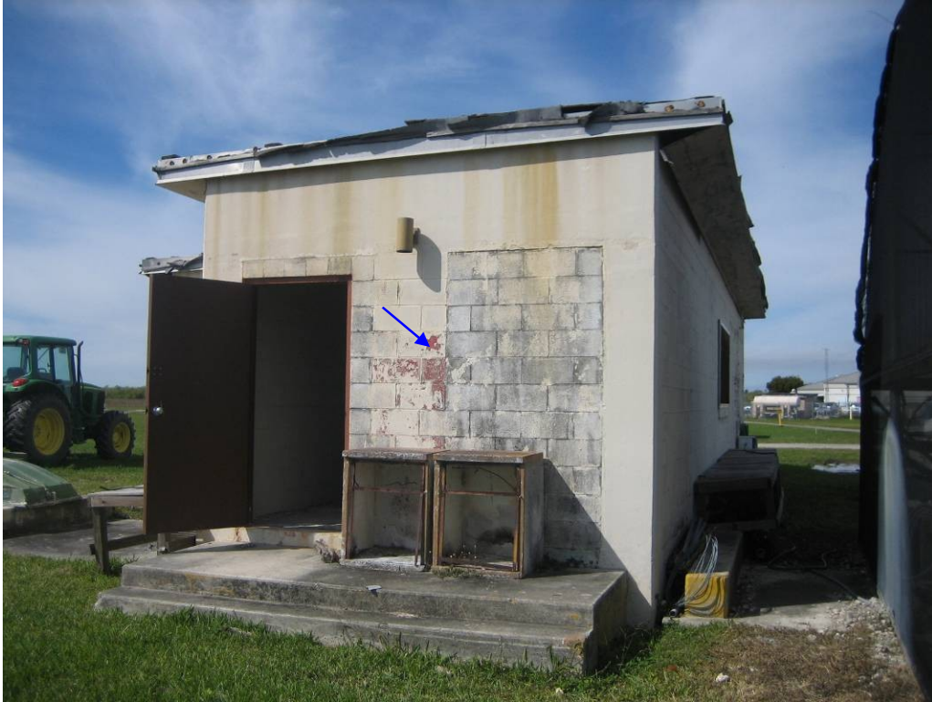
190B Building: Peeling red paint on exterior concrete block wall.
