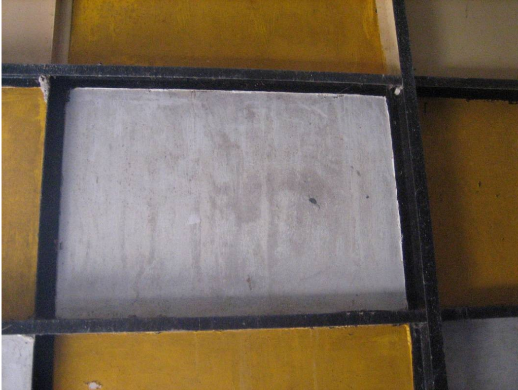
Missile Barn A: Chalking white paint on interior of barn door.
