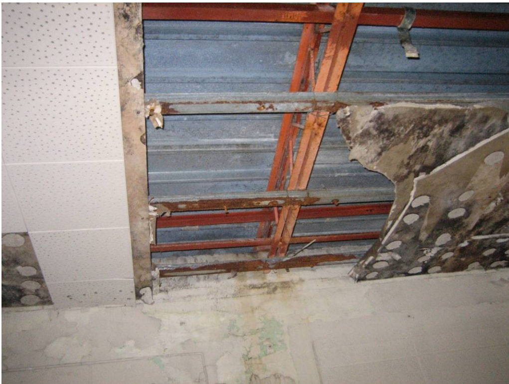
190B Building: Intact red paint on metal support beams.
