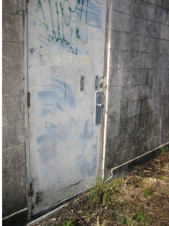
Missile Barn B: Cracked pink paint on exterior metal exit door.
