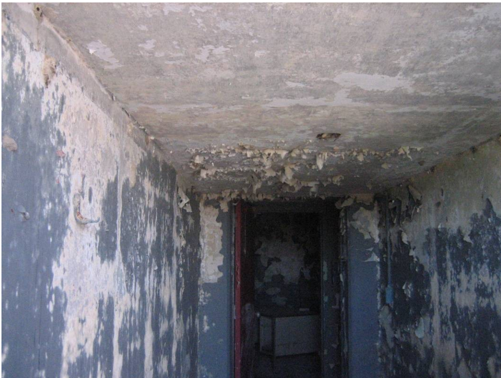
Fire-control Bunker A: Peeling gray paint on interior concrete walls.
