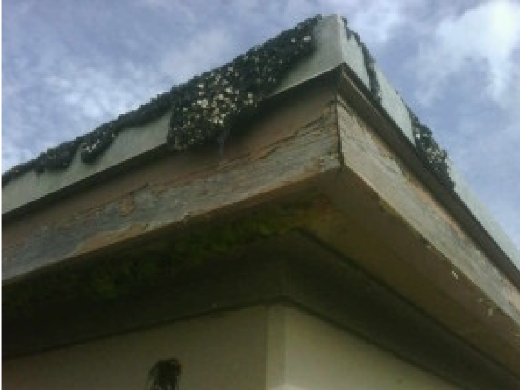
Water Pump House: Brown paint on wood soffit.
