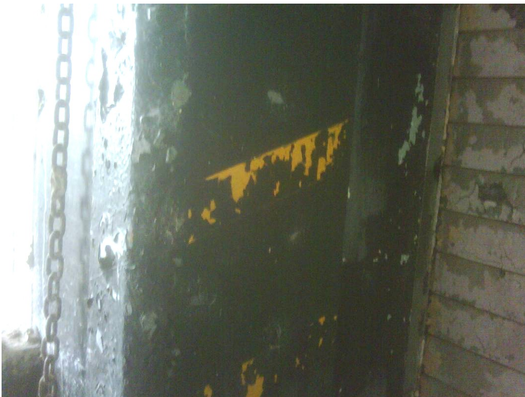
Missile Assembly Building: Peeling black paint on interior metal door and rail.
