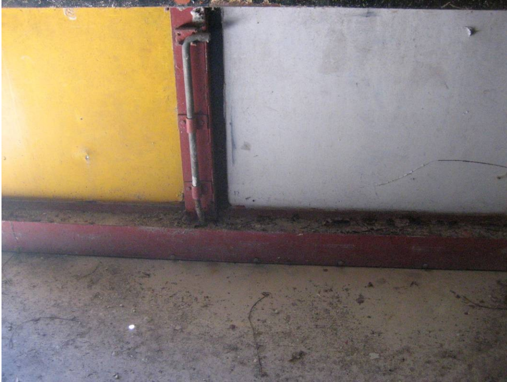
Missile Barn A: Chalking red paint on trim of interior barn door.
