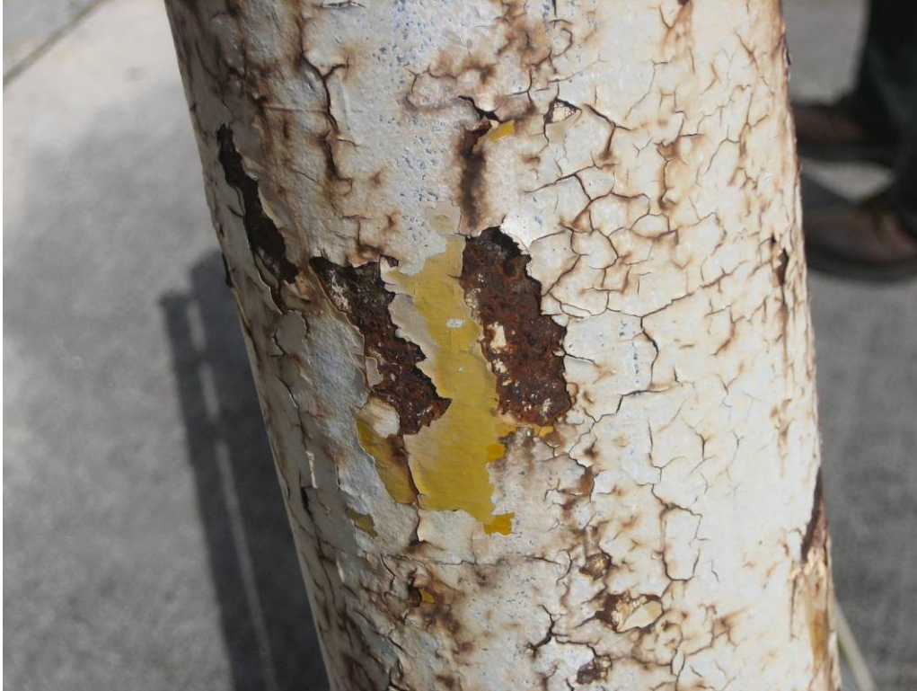
Missile Barn C: Cracked beige (yellow) on supports for rail beam on barn door.
