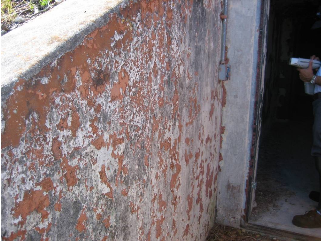
Fire-control Bunker C: Peeling red paint on exterior wall to bunker.
