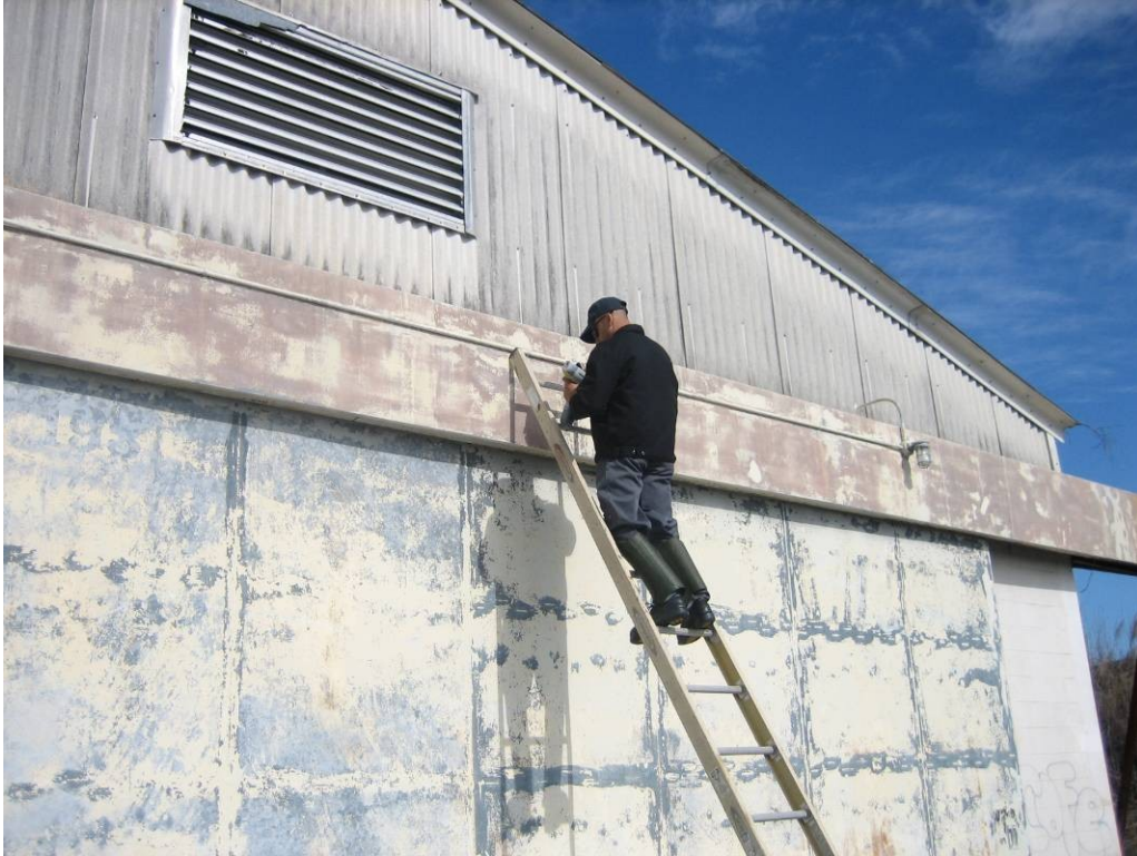
Missile Barn B: Cracked pink paint on metal rail beams on barn door.
