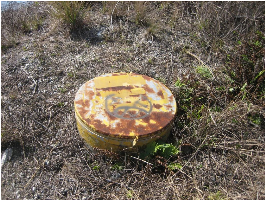
Missile Barn C: Peeling yellow paint on manhole cover near bunker.
