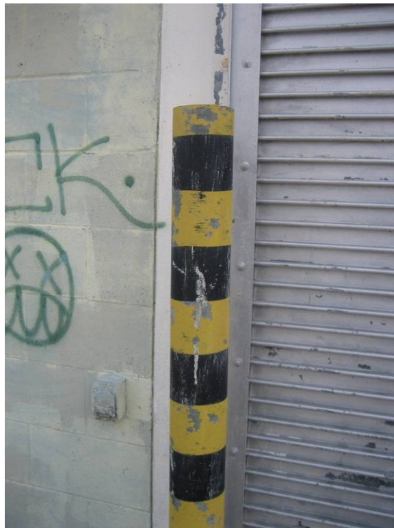
Missile Assembly Building: Cracked yellow paint on concrete bumper.
