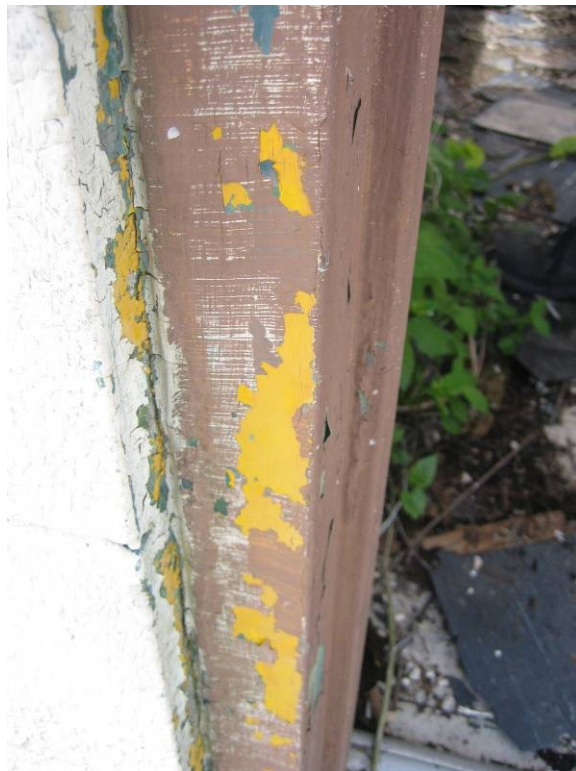
Kennel Building: Chalking brown paint on metal door casing.
