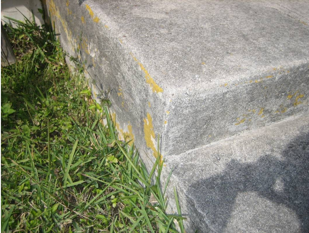
190B Building: Cracked yellow paint on concrete steps.
