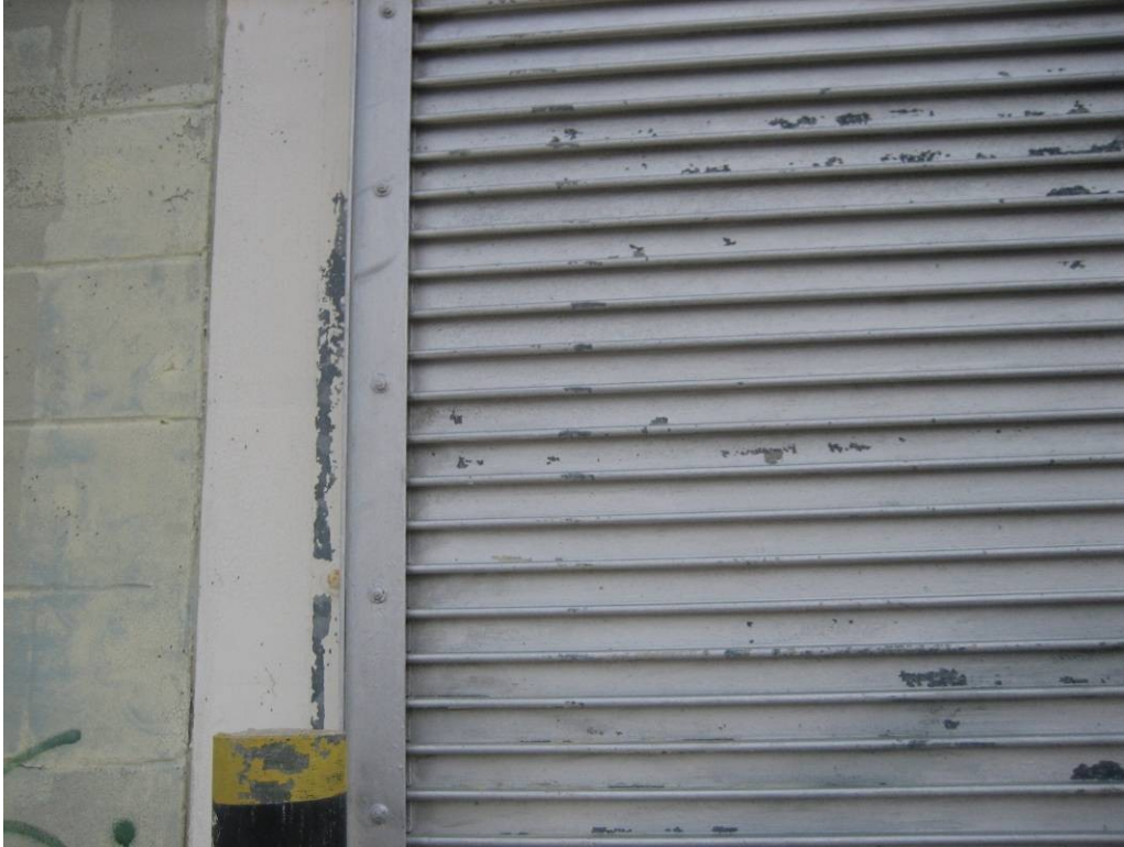
Missile Assembly Building: Cracked gray paint on exterior metal door and rails.
