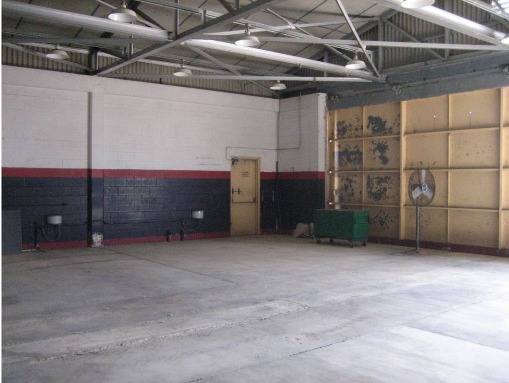
Missile Barn B: Blue paint on concrete block walls.
