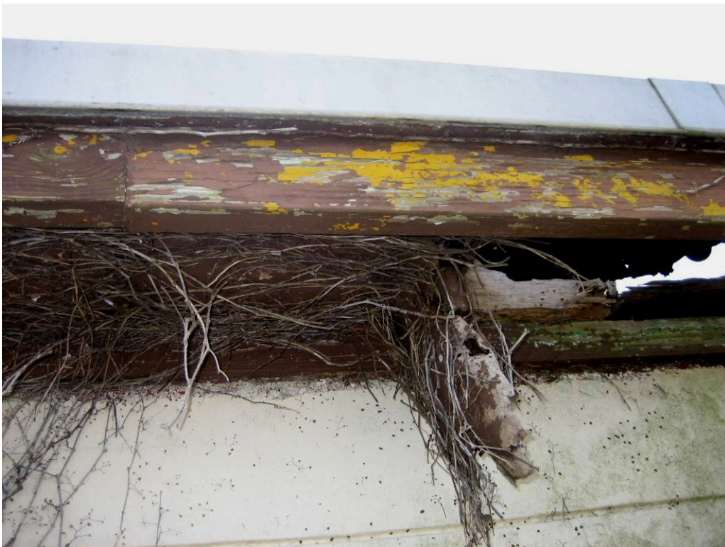
Kennel Building: Peeling brown (yellow) paint on exterior soffit trim.
