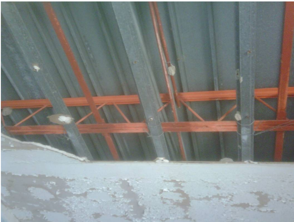
Missile Assembly Building: Intact red paint on red iron metal support beams.
