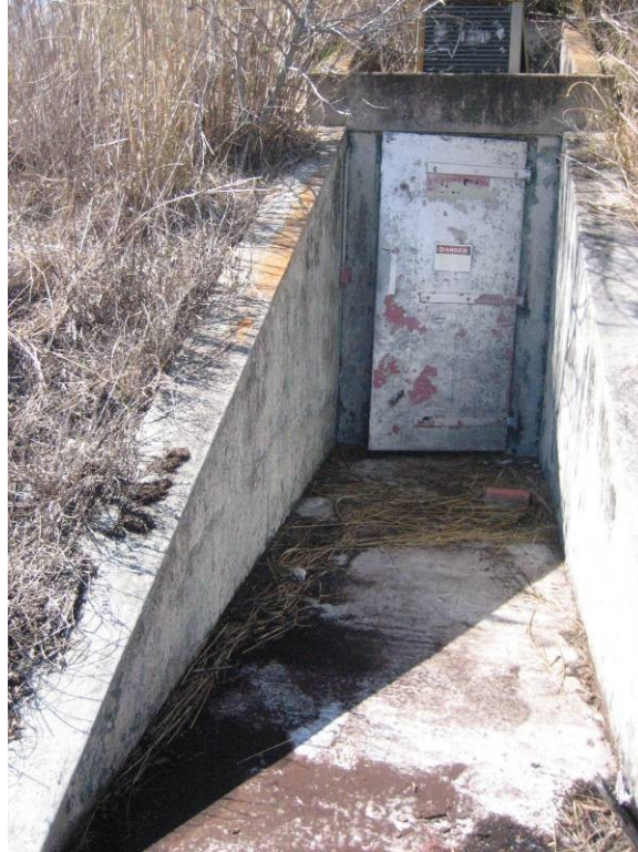
Fire-control Bunker B: Peeling red paint on exterior metal door.
