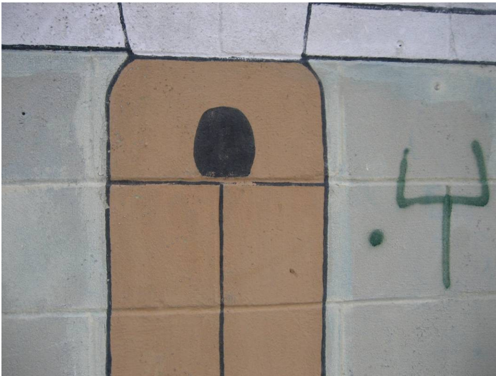
Missile Assembly Building: Detail of cracked beige and black paint on insignia.
