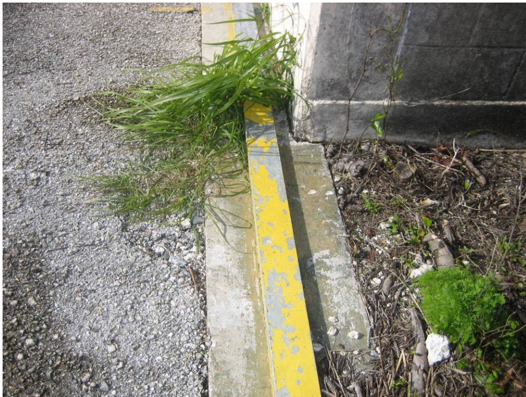
Missile Barn B: Cracked yellow paint on base rail of barn door.
