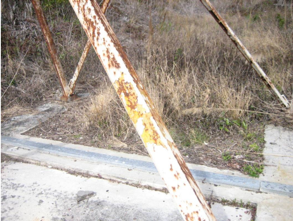
Missile Barn B: Cracked beige (yellow) paint on supports for rail beam on barn door.
