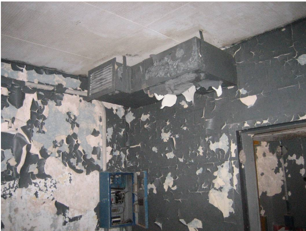
Fire-control Bunker A: Peeling gray paint on concrete walls.
