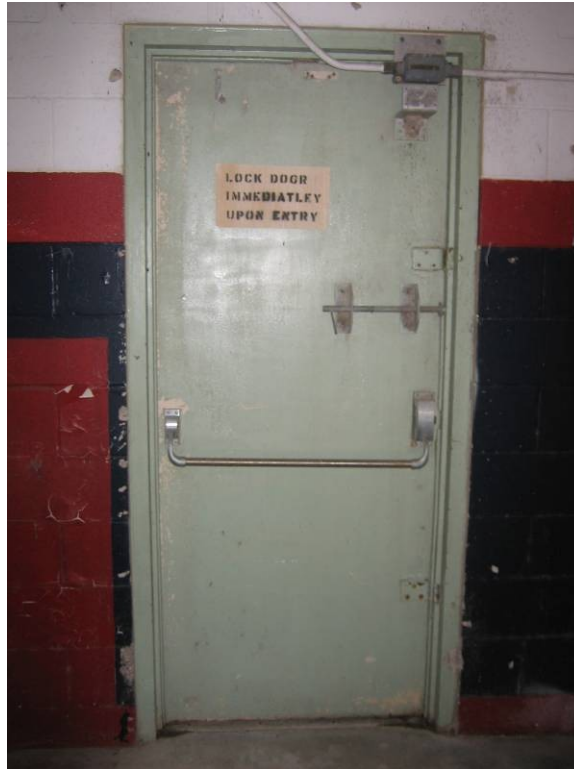
Missile Barn B: Peeling green paint on interior metal exit door.
