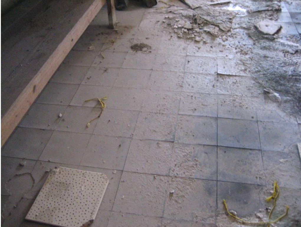
190 B Building: East side ACM 9" black vinyl floor tile and mastic.
