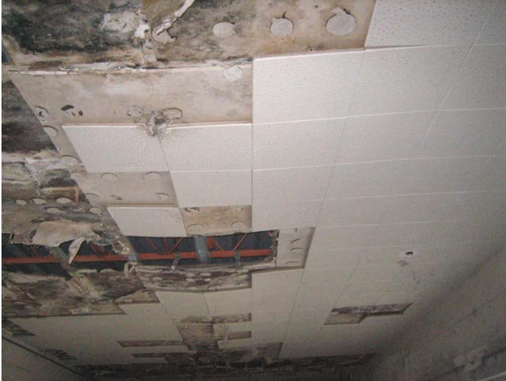
190 B Building: East side nonACM drywall, plaster, ceiling tile glue, and ceiling tile.
