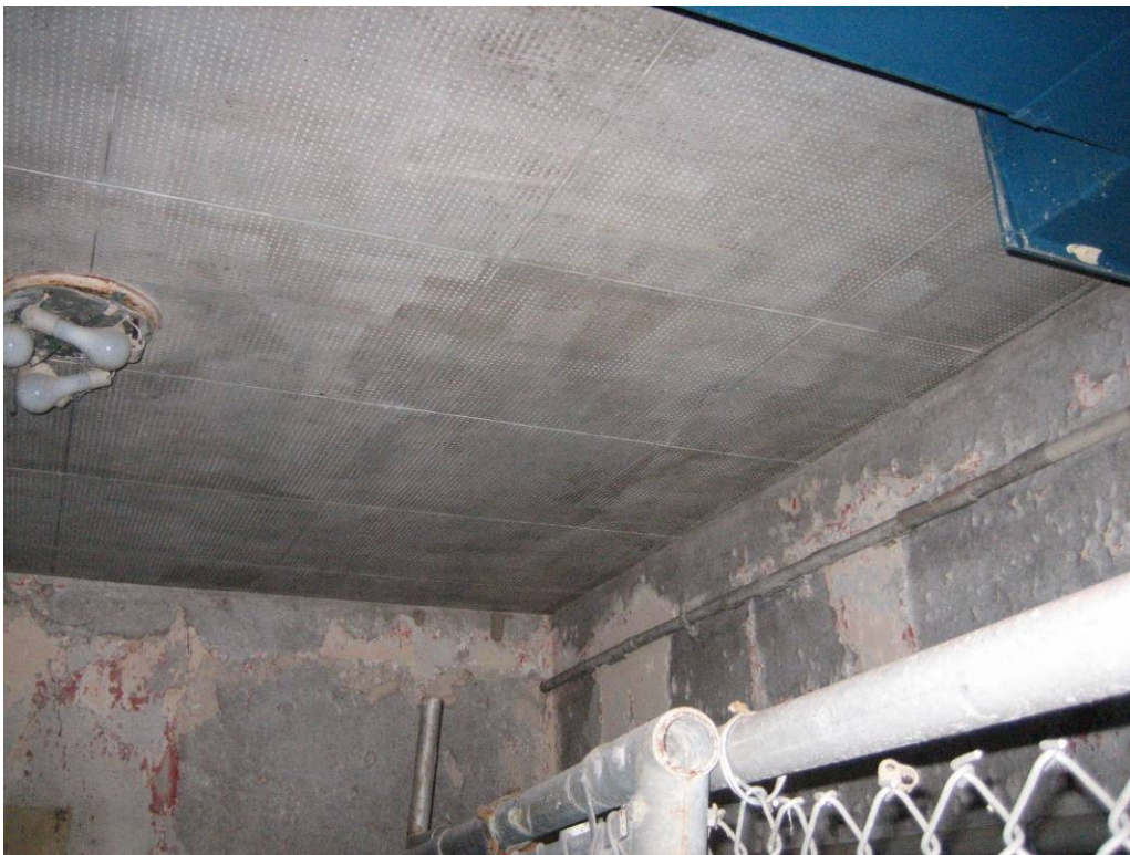
Fire-control Bunker B: ACM interior cementitious ceiling tiles.
