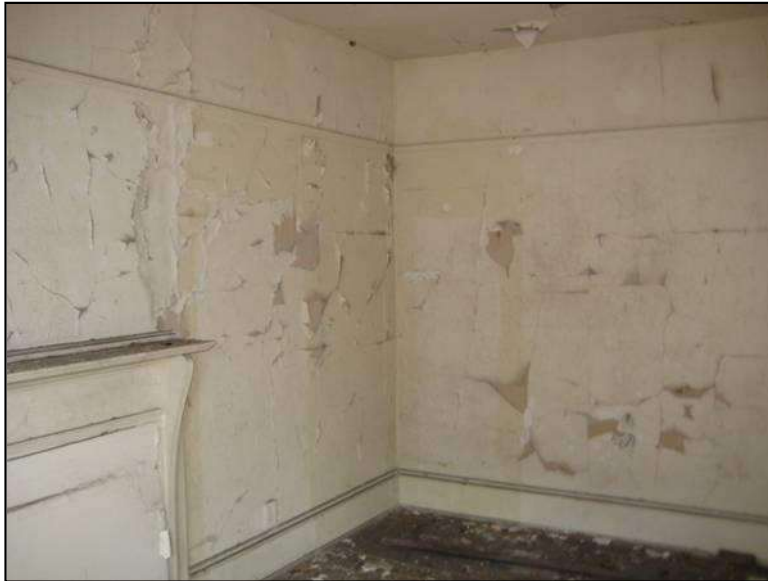
Figure 18 – Peeling plaster in room 203, southwest
