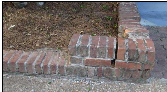
Figure 14 - Detail of loose brick, north
