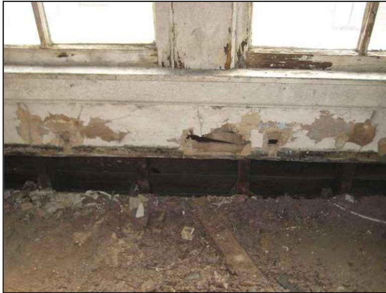
Figure 21 – Non-existent baseboard in room 203, east wall
