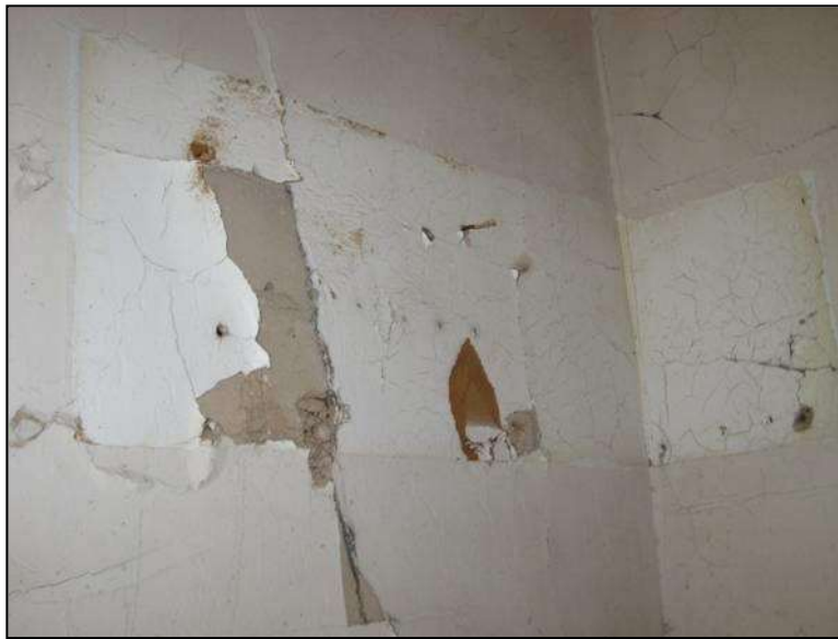
Figure 13 – Room 204 ghosting from cabinets, southeast wall
