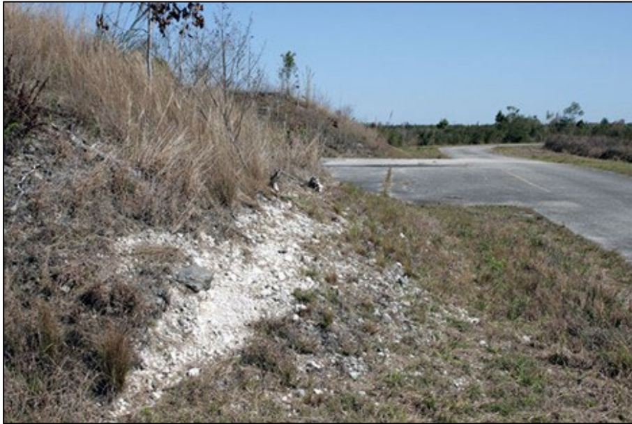
Fig 20. Mower wheels have damaged the berms. Source: JMA, 2010
