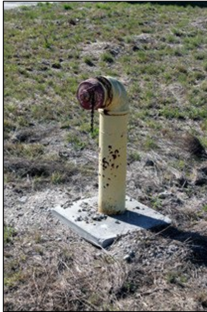
Fig 106. Dry hydrant adjacent to the missile assembly and test building. Source: JMA, 2010.
