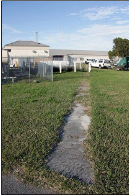
Fig 40. The concrete sidewalk along the pumphouse complex is in poor condition. Source: JMA, 2010.
