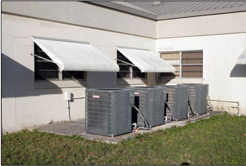
Fig 91. Air conditioning condenser units located behind the administration and barracks building. Source: JMA, 2010
