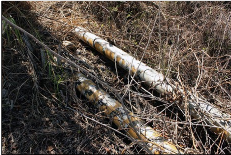
Fig 113. Metal cable conduits adjacent to launcher section control center B. Source: JMA, 2010.
