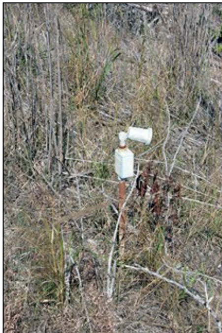
Fig 117. Each berm has several small luminaires on the north and south sides. Source: JMA, 2010.
