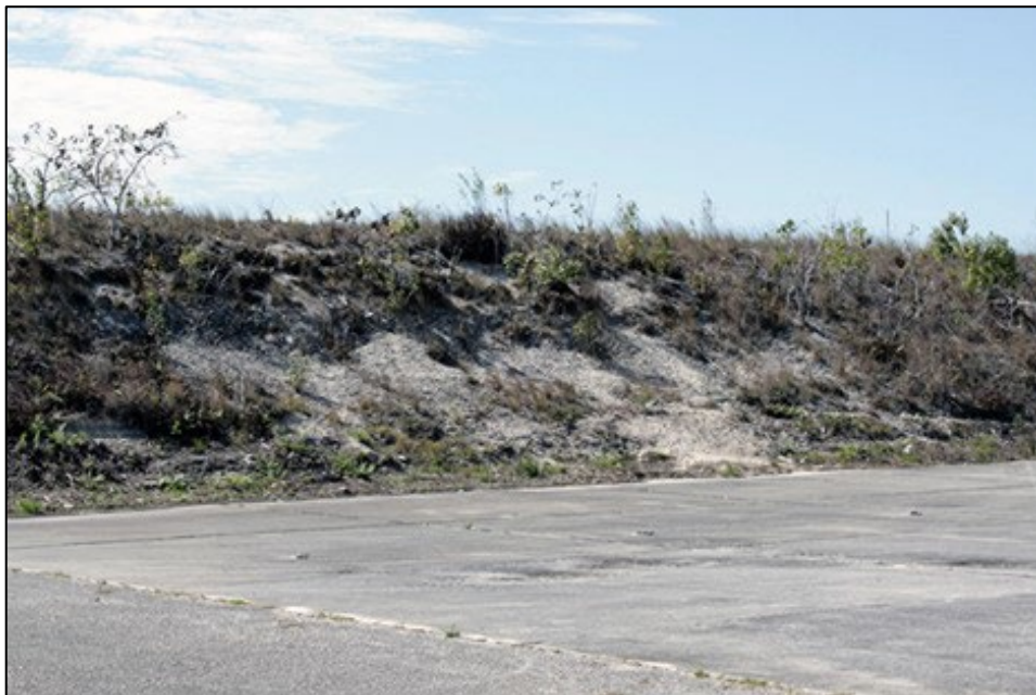
Fig 21. Launcher section B was used as a shooting range, damaging the berm. Source: JMA, 2010.
