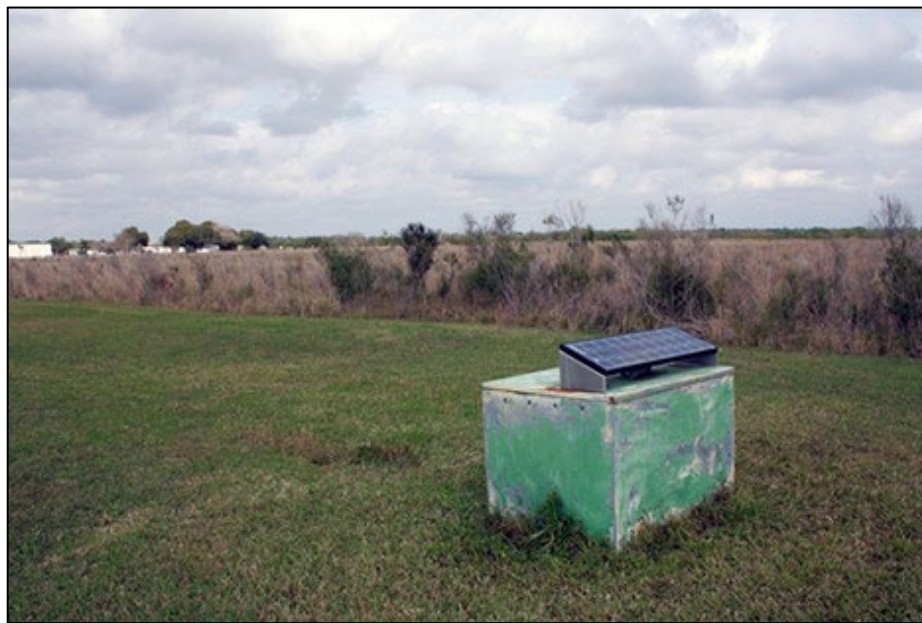
Fig 90. A box with solar panels located in the southeast corner of the Control Area. Source: JMA, 2010.
