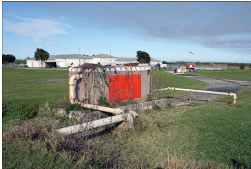
Fig 103. Pipes and pipe supports adjacent to and running into the drainfield from the septic tank. Source: JMA, 2010
