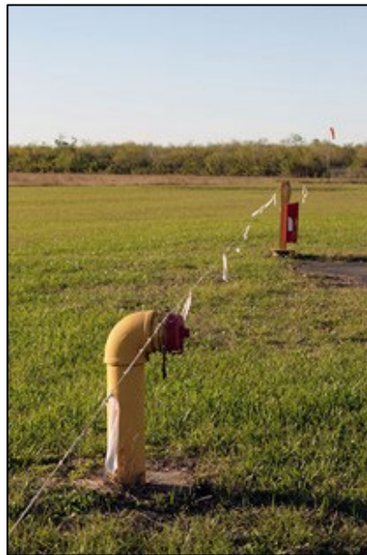
Fig 92. Three dry hydrants are located within the Control Area. Source: JMA, 2010
