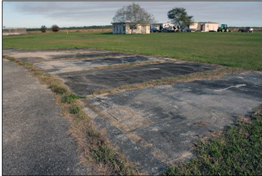
Fig 43. Cracked asphalt parking spaces near the Control Area drainfield. Source: JMA, 2010.
