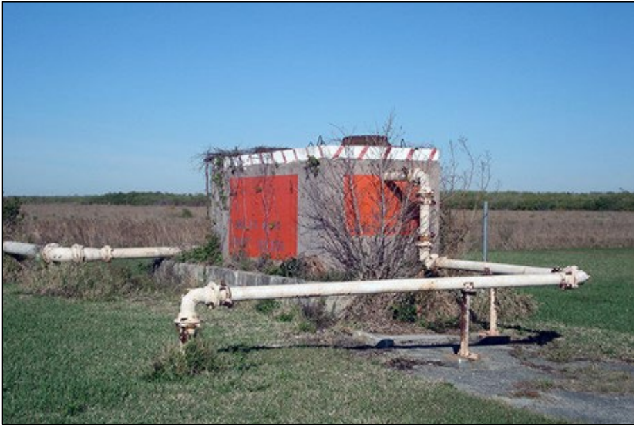
Fig 67. Septic tank. Source: JMA, 2010
