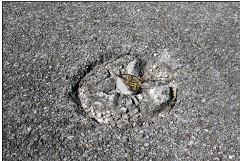
Fig 50. Remnants of the Launch Area security gates are still embedded in the loop road. Source: JMA, 2010.
