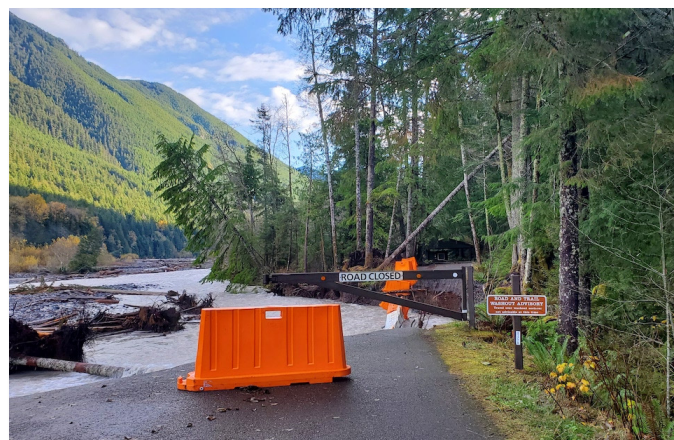
Figure 1. Asphalt roadbed that was eroded by high water from the storm event, November 2021 (NPS photo).
