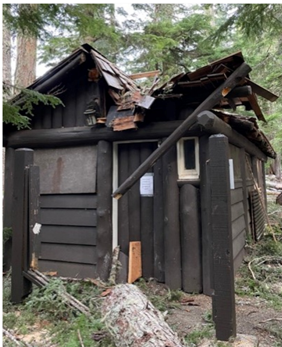
Figure 3. Treefall during high winds damaged buildings near the White River Entrance during the November 2021 storm (NPS photo).
