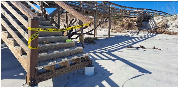
Damage from Tropical Storm Ian at Fort Matanzas National Monument. NPS photo / Kurt Foote, FOMA staff.
