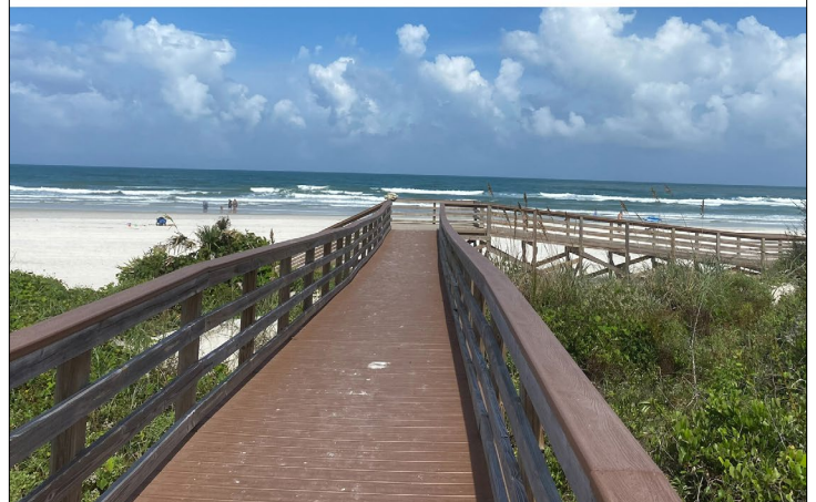
Top, damage to the Fort Matanzas National Monument beach access ramp due to shoreline erosion from Hurricane Nicole in November 2022 (NPS photo / Kurt Foote, FOMA staff). Bottom, beach access boardwalk before the storm on August 28, 2021 (Photo by Melanie Vervaeke).
