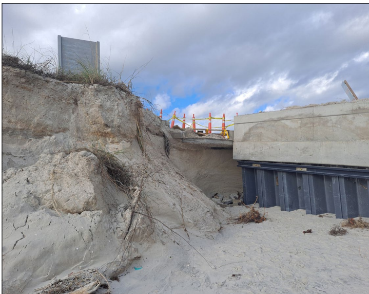
Erosional damage to the car ramp on the Atlantic beachfront at Fort Matanzas National Monument. NPS photo / Kurt Foote, FOMA Staff.
