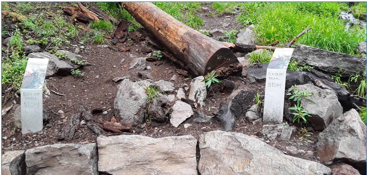
Figure 3. The condition of the trail terminus prior to fence installation. Photo by Jen Hooke.
