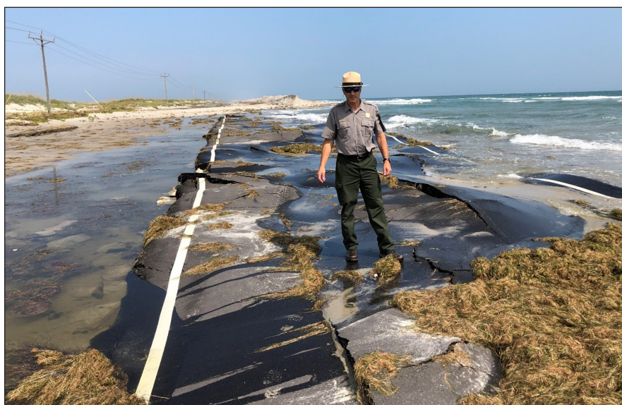
Figure 3. Superintendent of Cape Hatteras National Seashore standing on a damaged stretch of NC-12 on Ocracoke Island post-Dorian (NPS 2019).
