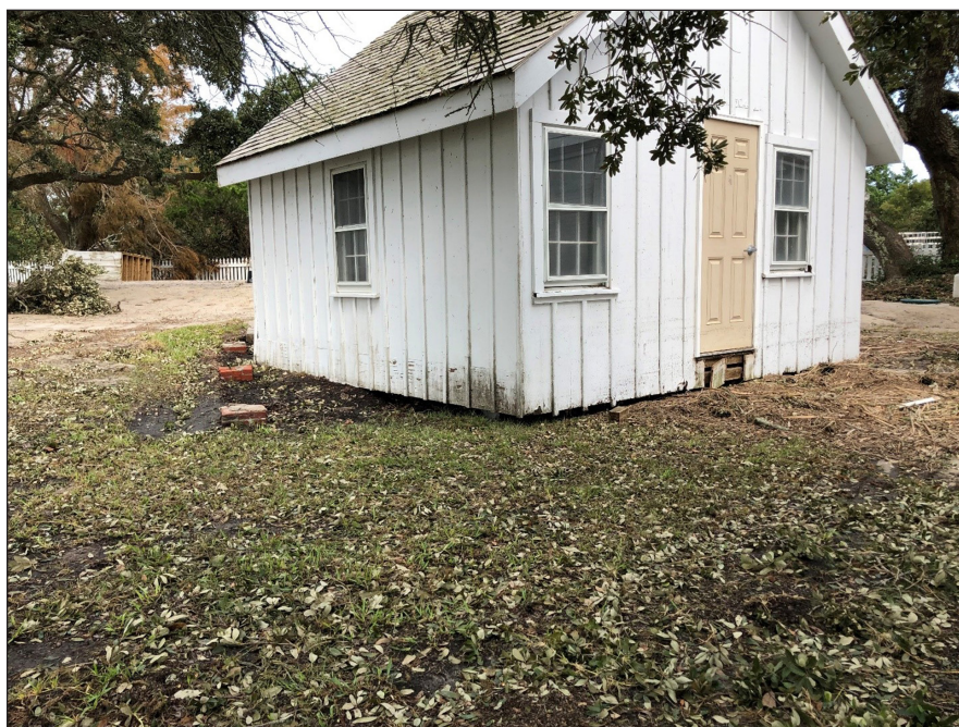
Figure 2. Storm surge from Hurricane Dorian flooded the inside of the old store house at the Ocracoke Light Station with over a meter of water and lifted it off its foundation (NPS 2019).
